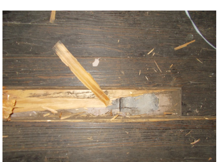
Photo 18 – Paper under wooden flooring throughout
