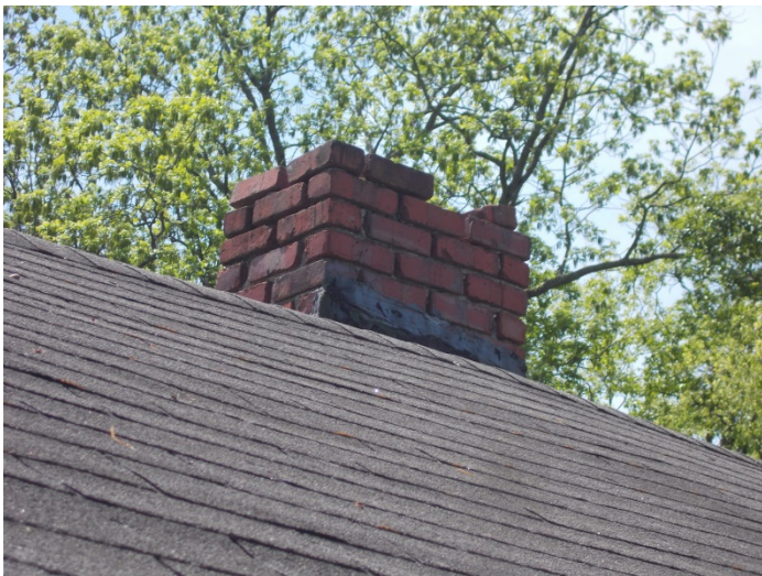
Photo 3 – 1 chimney with mastic/tar in middle of roof
