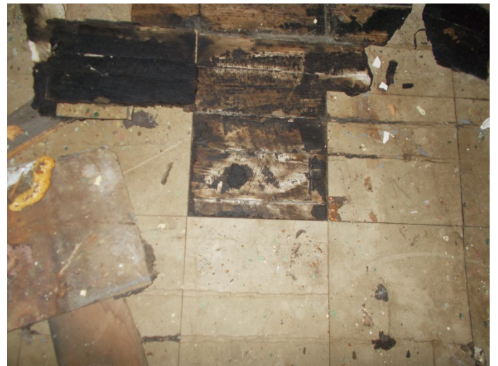
Photo 10 – 9" x 9" brown speckled floor tile & felt in the kitchen
