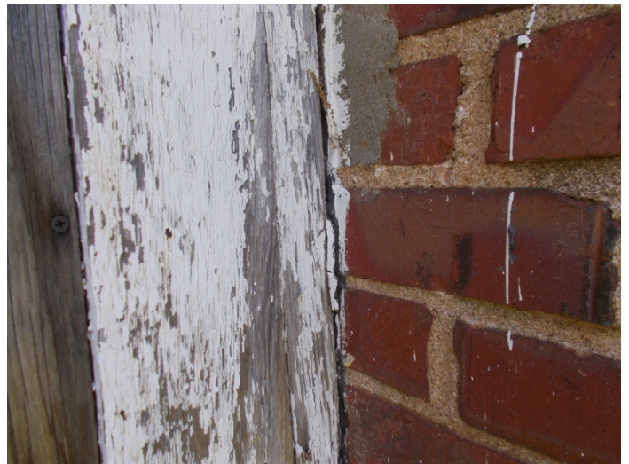
Photo 6 – caulk on 2 chimneys & adjacent siding on the right side of the house
