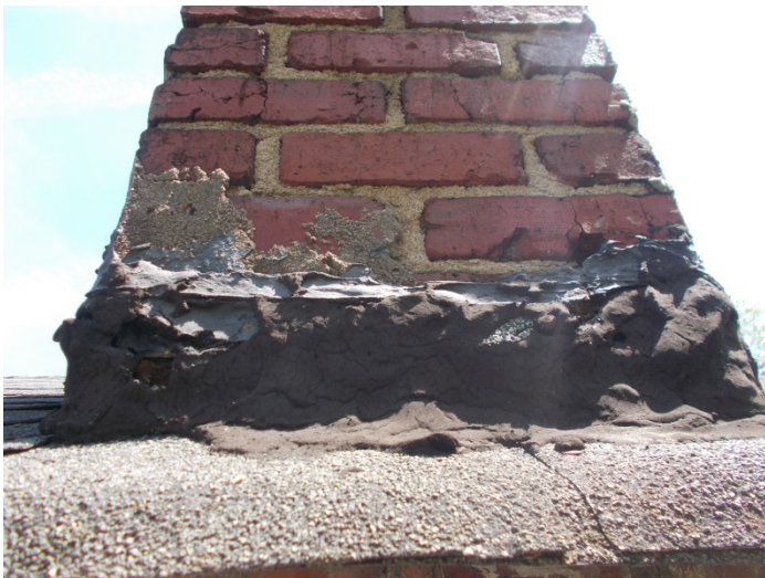
Photo 5 – mastic/tar on chimney
