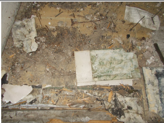
Photo 11 – Beige square pattern vinyl floor with mastic over floor tile & felt in the bathroom
