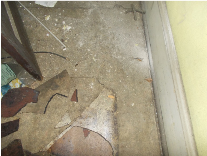
Photo 13 – Tan & brown digital pattern vinyl floor & mastic in the hallway (2 layers) & front left bedroom (top layer)
