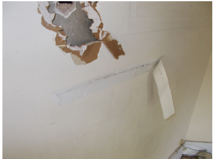
Photo 8 – Drywall with joint compound & tape throughout
