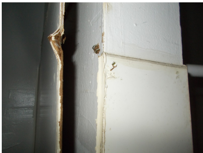
Photo 20 – Tub/shower surround caulk in the front & back bathrooms
