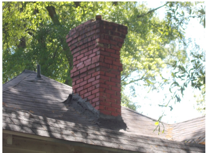
Photo 6 – mastic/tar on 2 chimneys – assumed positive.
