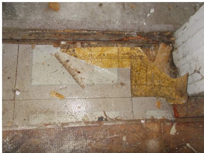
Photo 19 – 12" x 12" grey pattern self-stick floor tile & mastic over yellow square pattern vinyl floor & mastic in the back entry hallway (under wood)
