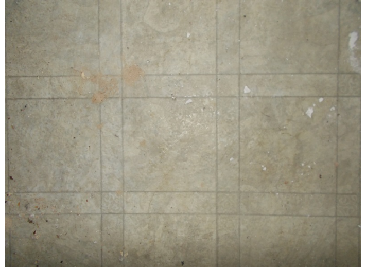
Photo 16 – Beige square pattern vinyl floor with no mastic in the front bathroom (2nd layer); kitchen (top layer) & back bathroom (top layer)
