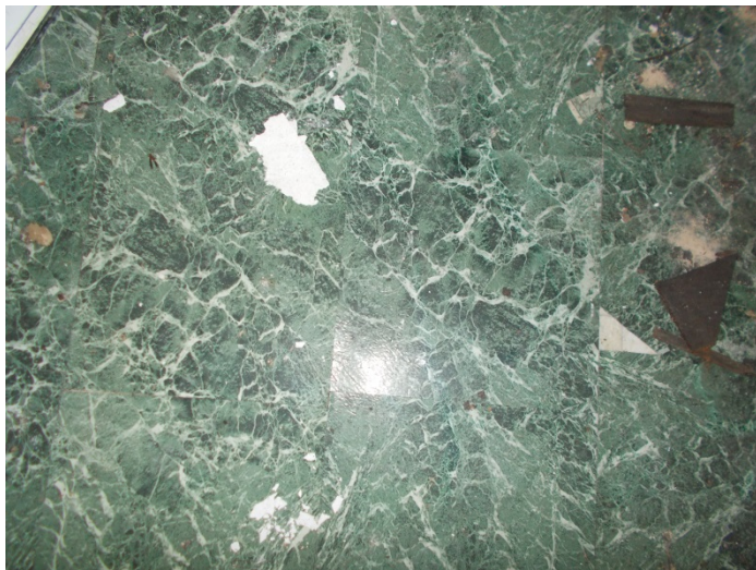
Photo 15 – 12" x 12" green marble pattern self-stick floor tile & mastic in the front bathroom (top layer)
