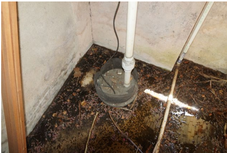
Exterior sump pump under mail stairs
