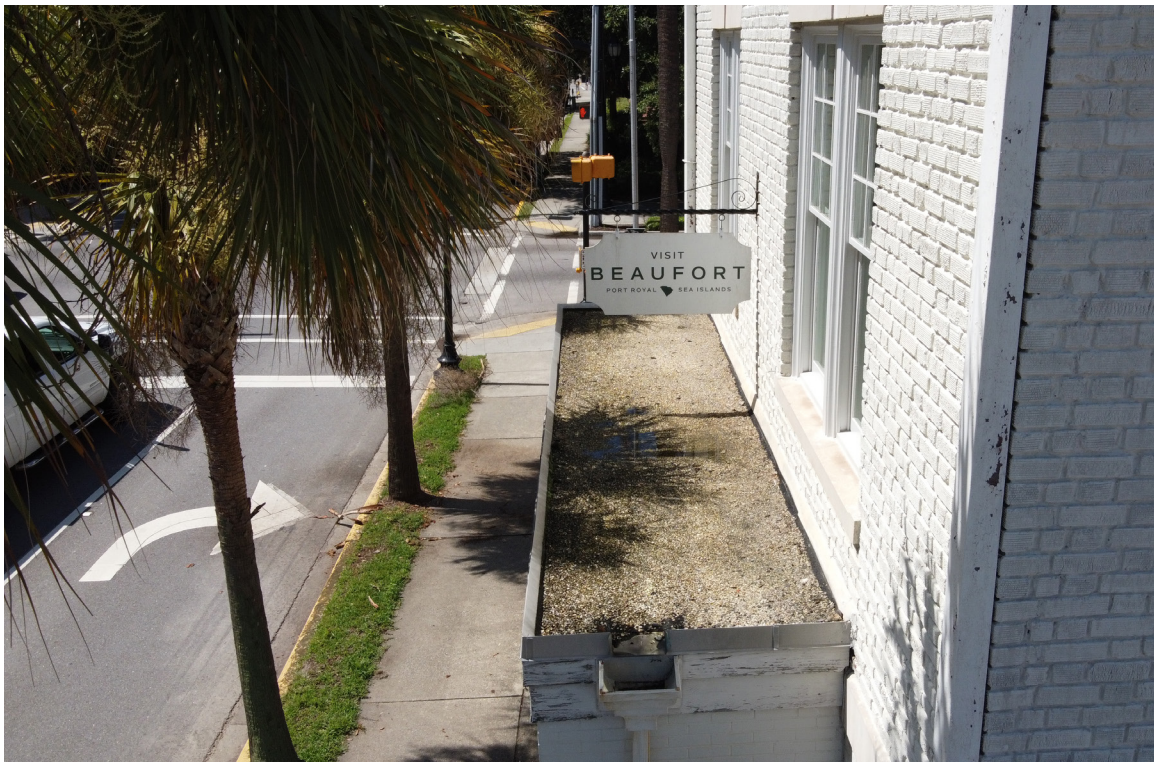
Figure 57: Beaufort Carnegie Library Building, East Elevation Addition Roof: View of the asphalt roof with ballast. The roof appears to hold water, but no evidence of water infiltration was found on the interior.
