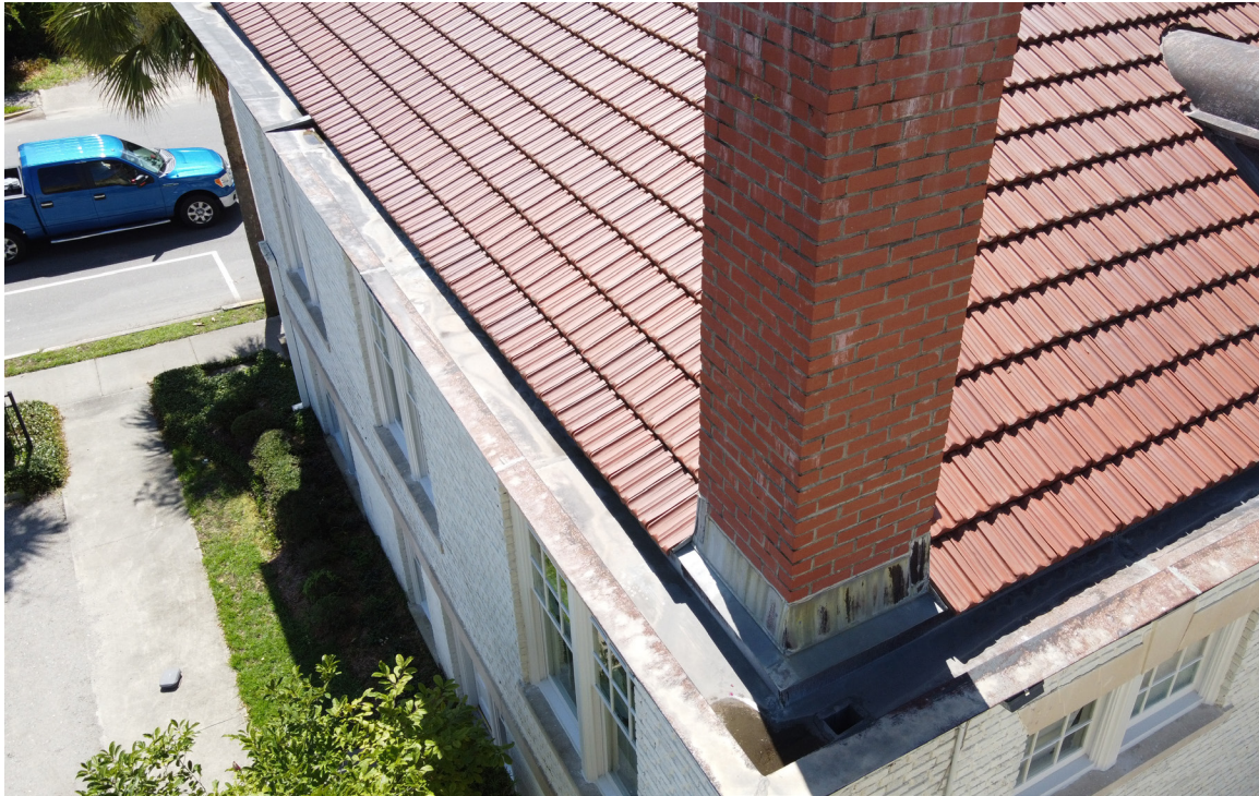
Figure 46: Beaufort Carnegie Library Building, View of flashing on the corner chimney. The reglet should be recaulked where it intersects the masonry.
