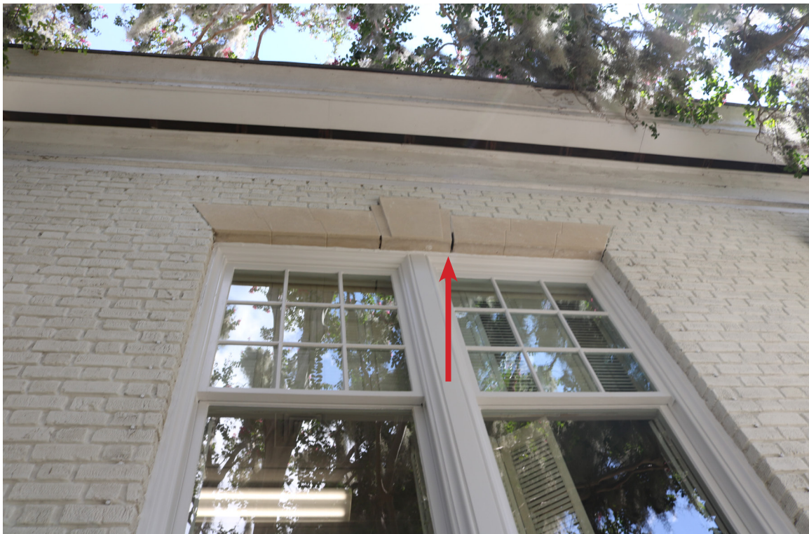
Figure 22: Beaufort Carnegie Library Building, Masonry Keystone: View of mortar loss next to the limestone keystone (arrow).
