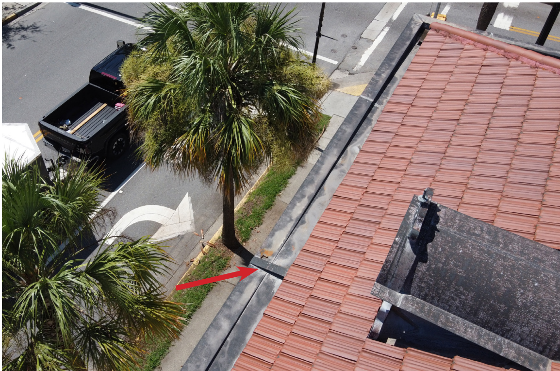
Figure 55: Beaufort Carnegie Library Building, East Elevation Aerial: The expansion joint on the east elevation is in good condition. A loose fastener is visible in the gutter (arrow).
