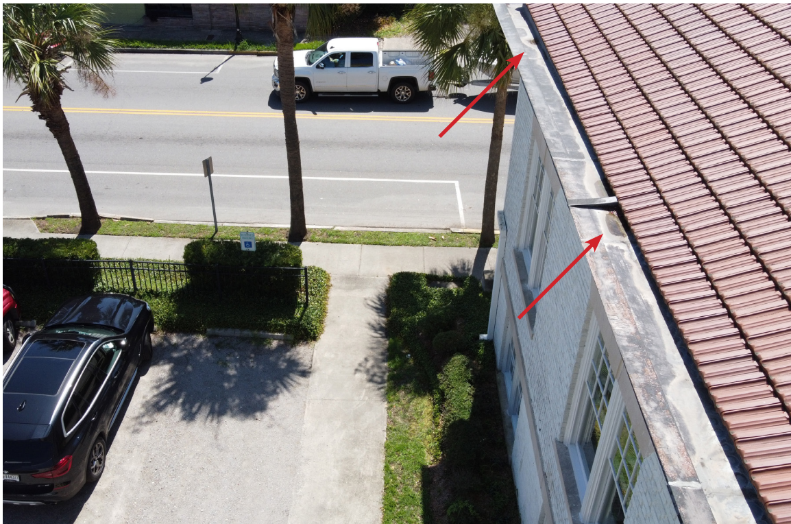
Figure 53: Beaufort Carnegie Library Building, North Elevation: Detail of built-in gutter on this side of the building. Standing water is present next to the expansion joint and on the east side (arrows).
