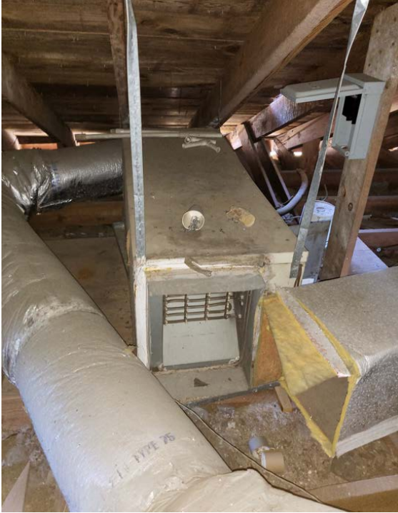
Abandoned AHU and ductwork
