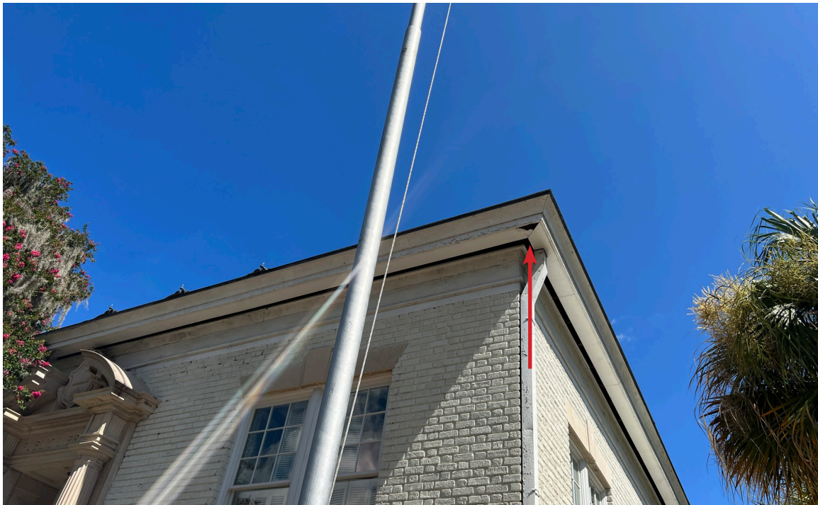
Figure 62: Beaufort Carnegie Library Building, Southeast Corner: The soffit has deteriorated at this corner.
