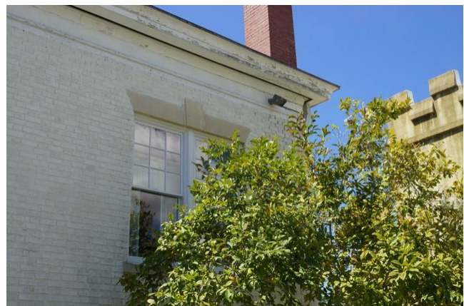
Exterior flood light
