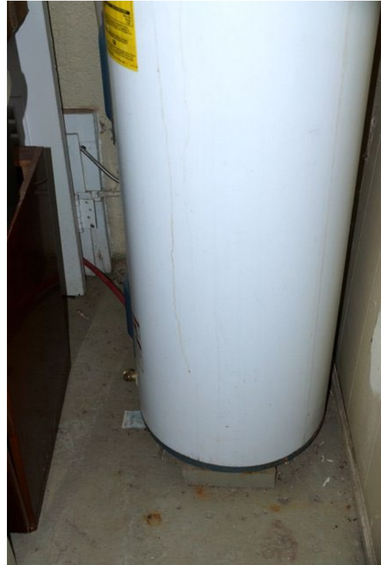
Water heater, no drain pan
