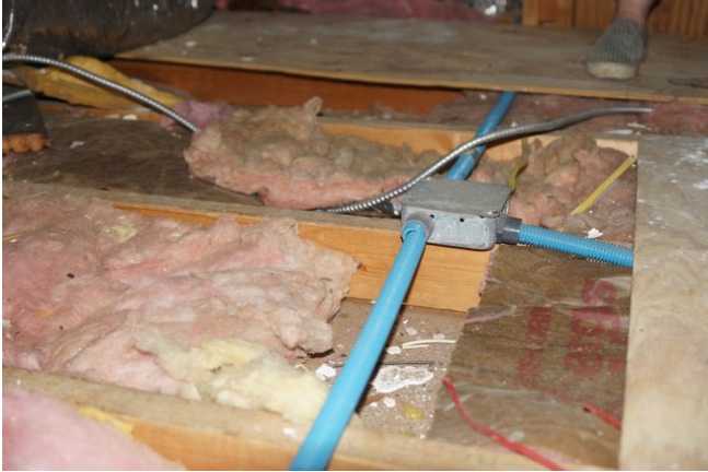
MC, ENT and NM cable in attic
