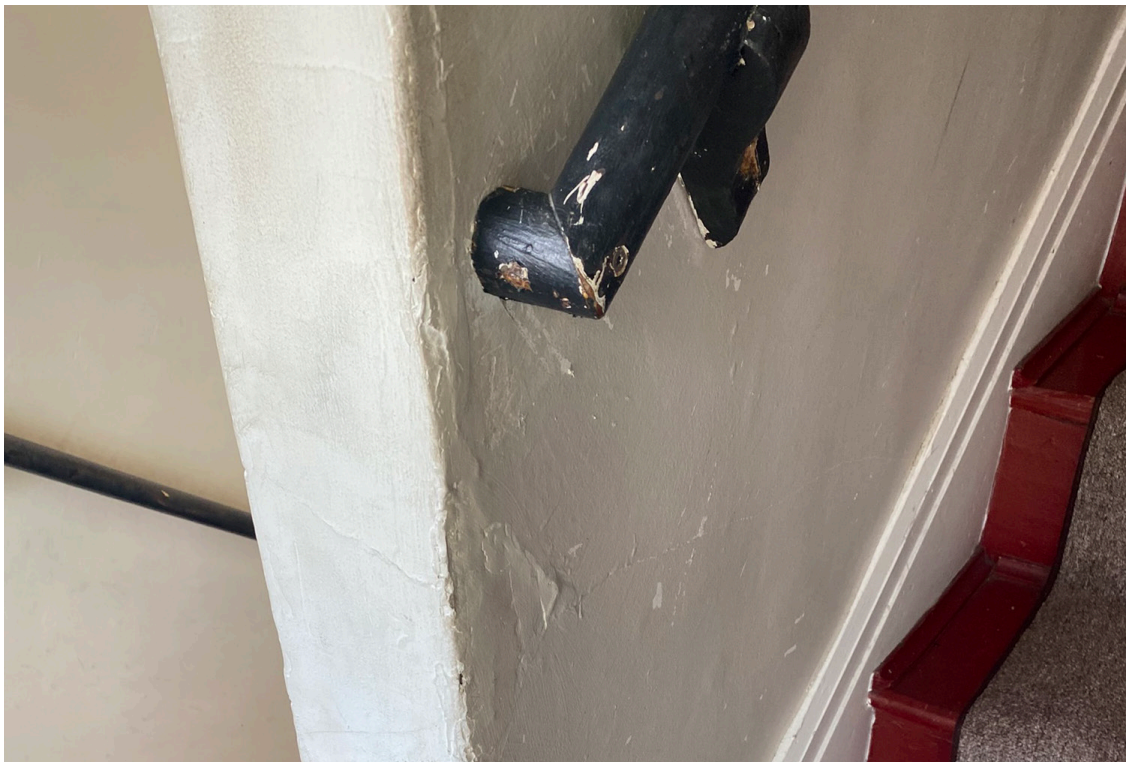
Figure 94: Beaufort Carnegie Library Building, First-Floor Landing: View of plaster damage and paint loss in the interior stair hall.
