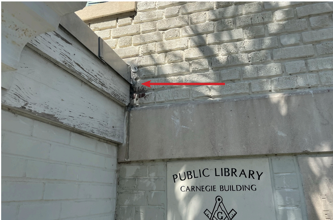
Figure 31: Beaufort Carnegie Library Building, East Elevation. View of the intersection of the east entrance addition and the masonry wall. A gap is present between the wood and brick (arrow).
