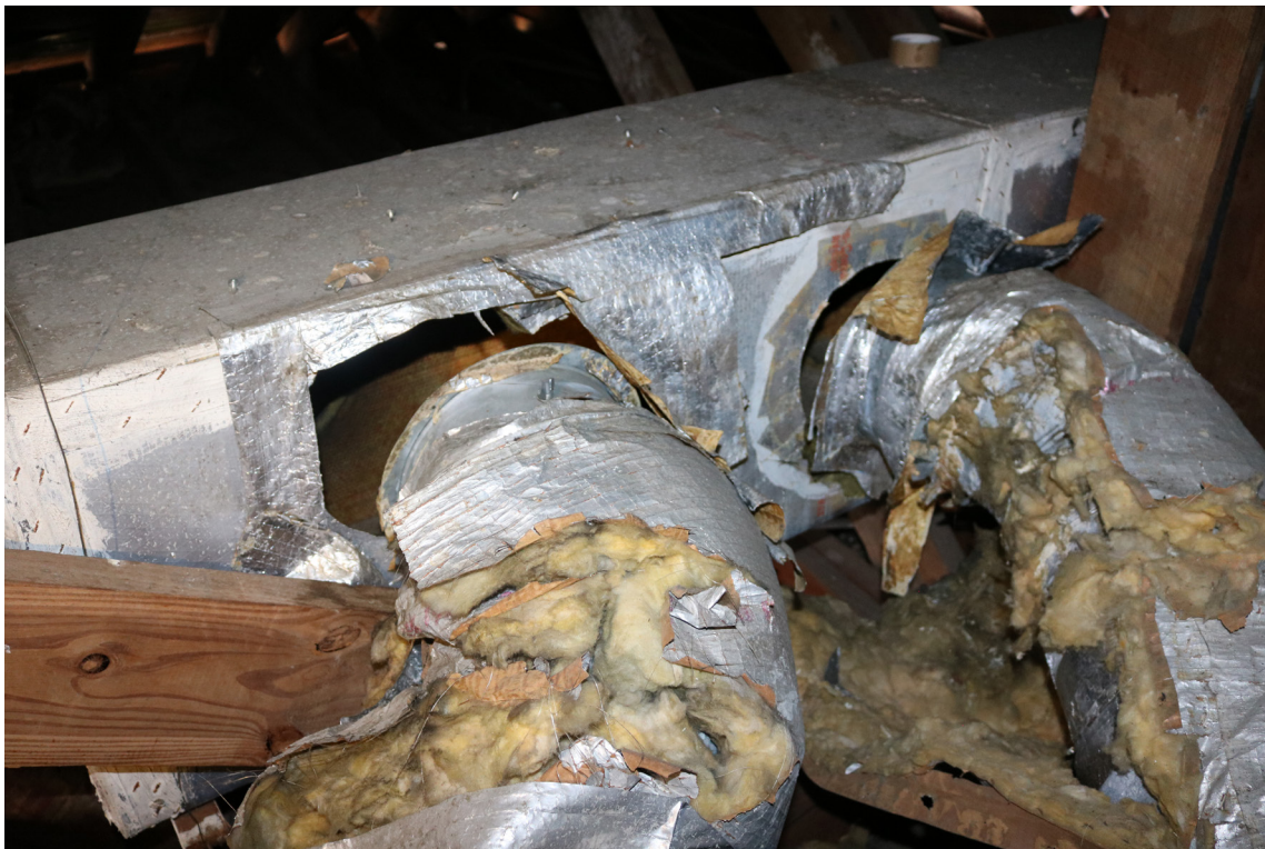
Figure 78: Beaufort Carnegie Library Building, Attic, Upper Level: View of disconnected ductwork.
