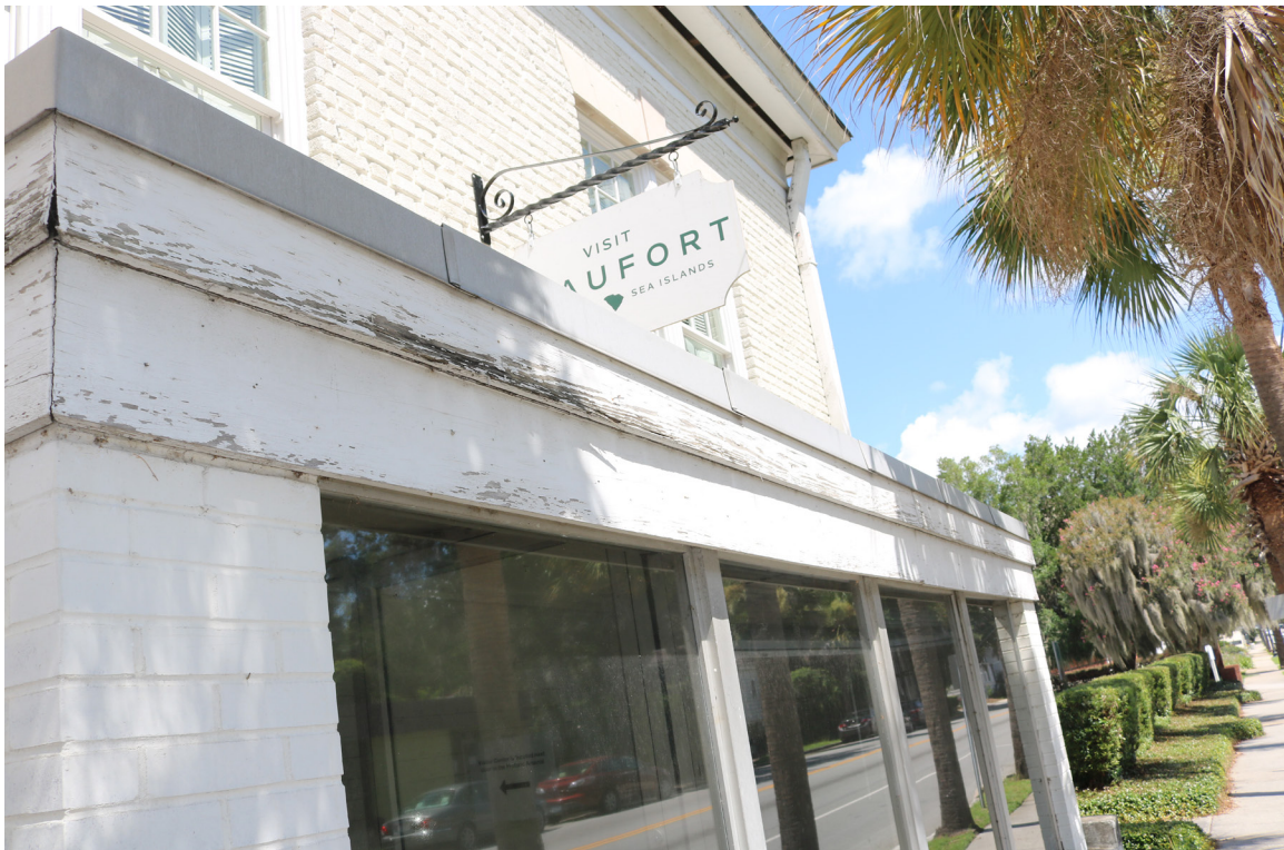
Figure 69: Beaufort Carnegie Library Building, East Addition: The woodwork on the addition has extensive paint failure.
