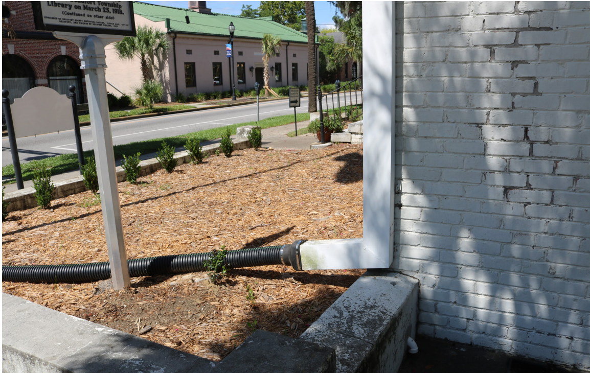
Figure 58: Beaufort Carnegie Library Building, Southeast Downspout: The downspout at this corner connects to an extender that drains to the garden bed and sidewalk.
