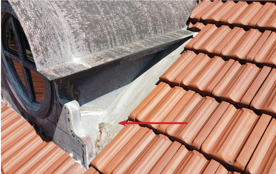
Figure 37: Beaufort Carnegie Library Building, South Elevation Dormers: The dormers are installed over two layers of felt roofing, and the tiles are laid around the dormer openings. This area has been recalced several times (arrow).
