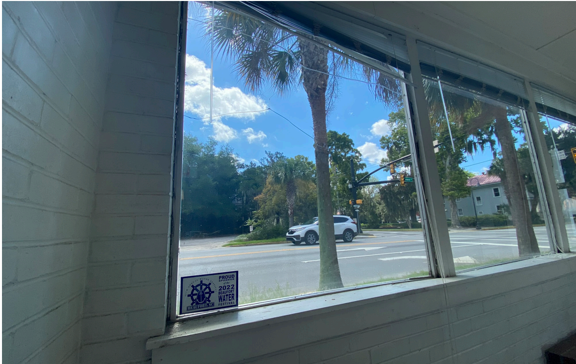
Figure 71: Beaufort Carnegie Library Building, East Addition: The windows should be replaced. The exterior window sills have a negative slope, allowing water to enter the building.
