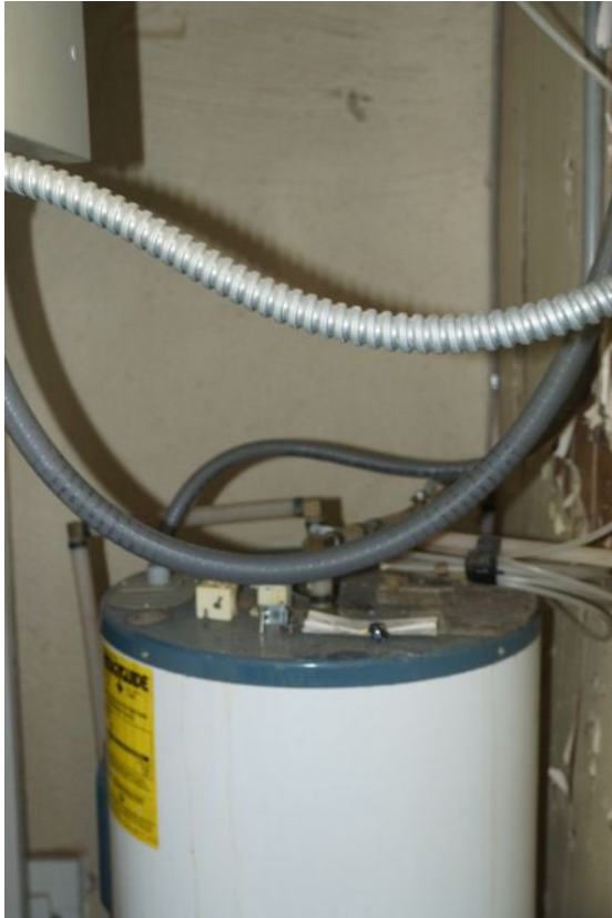
Water heater, PEX B piping, no expansion tank
