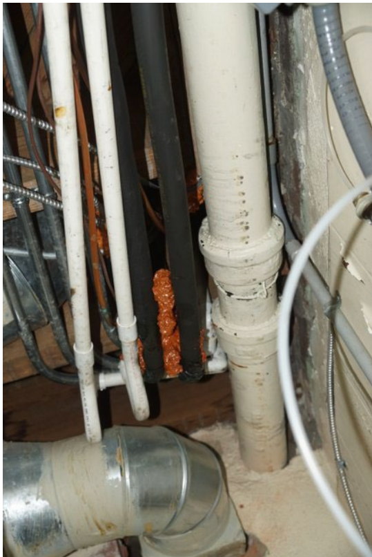
Cast iron waste piping
