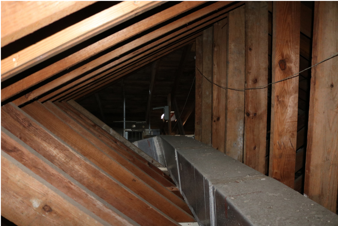
Figure 76: Beaufort Carnegie Library Building, Attic, Upper Level: View of the original attic with exposed rafters. A central HVAC line runs in the middle of the upper attic.
