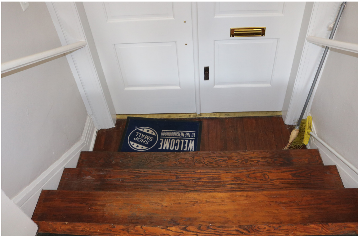
Figure 90: Beaufort Carnegie Library Building, South Vestibule: The original pine flooring and stair treads are exposed at this location. The original wood flooring appears to be preserved beneath the office carpet, but the condition is unknown.
