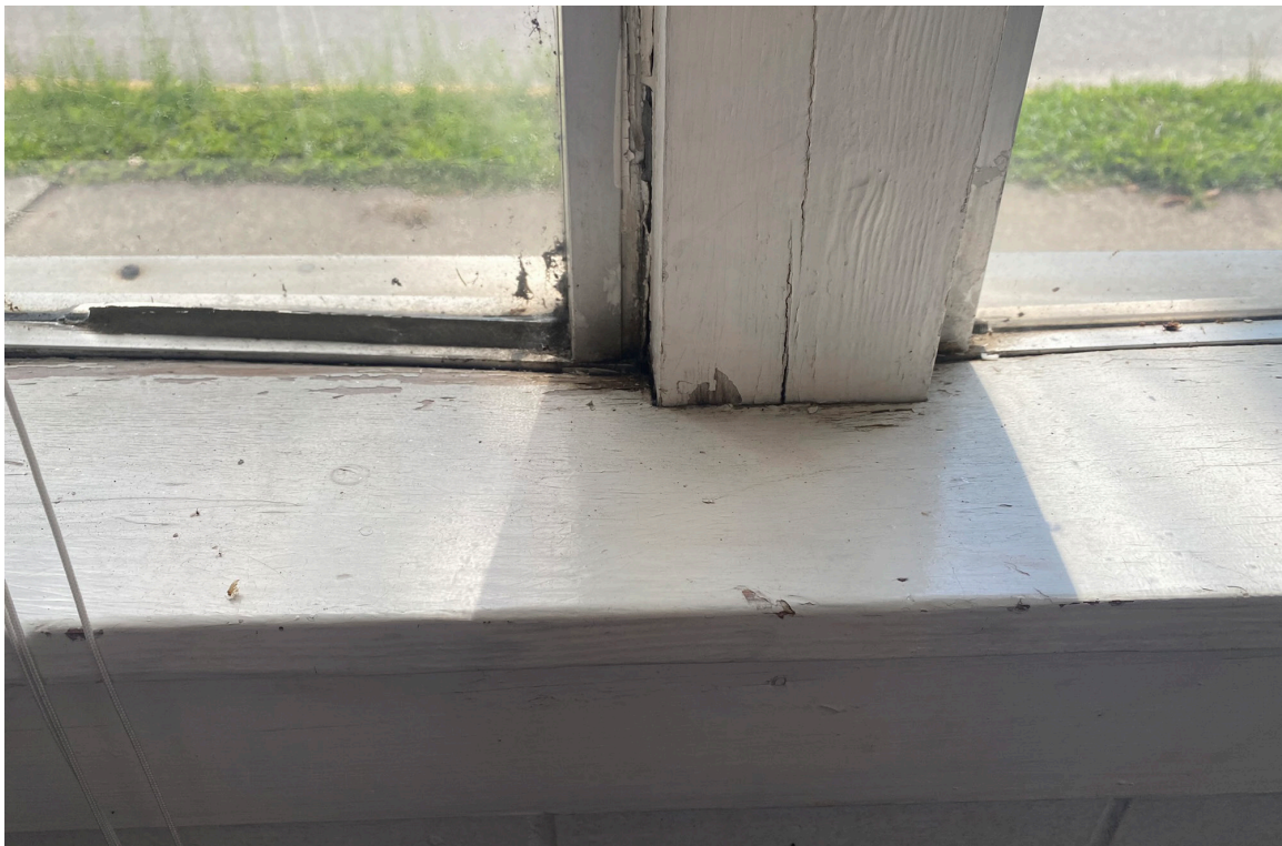
Figure 72: Beaufort Carnegie Library Building, East Addition: The interior stools should be replaced. The stools are damaged from water infiltration.
