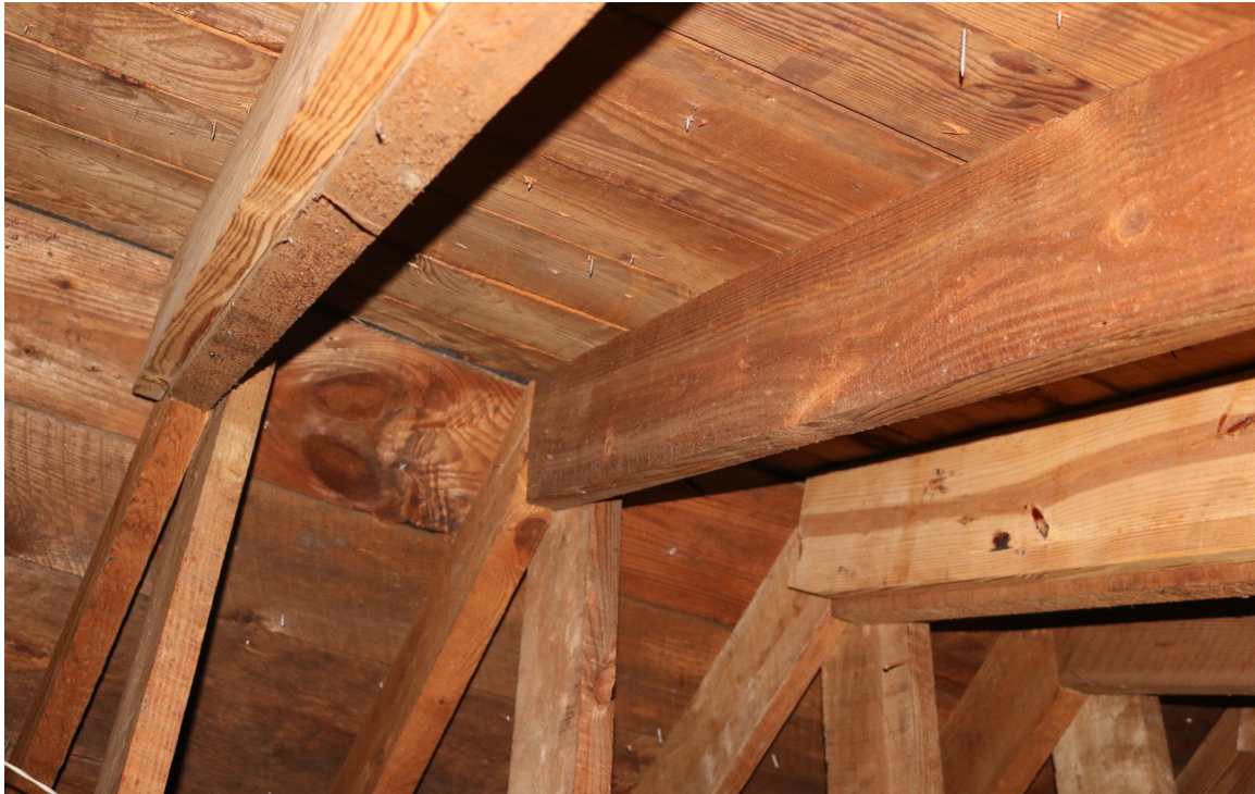
Figure 83: Beaufort Carnegie Library Building, Attic Ridge: No evidence of water damage was observed at the ridge despite the mortar loss on the exterior.
