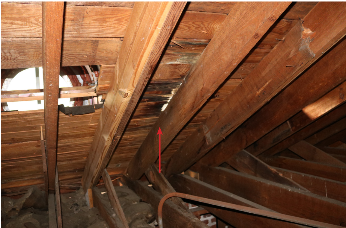
Figure 80: Beaufort Carnegie Library Building, Attic, Looking South: View of deteriorated roof decking and mold growth to the west of the southeast dormer (arrow).
