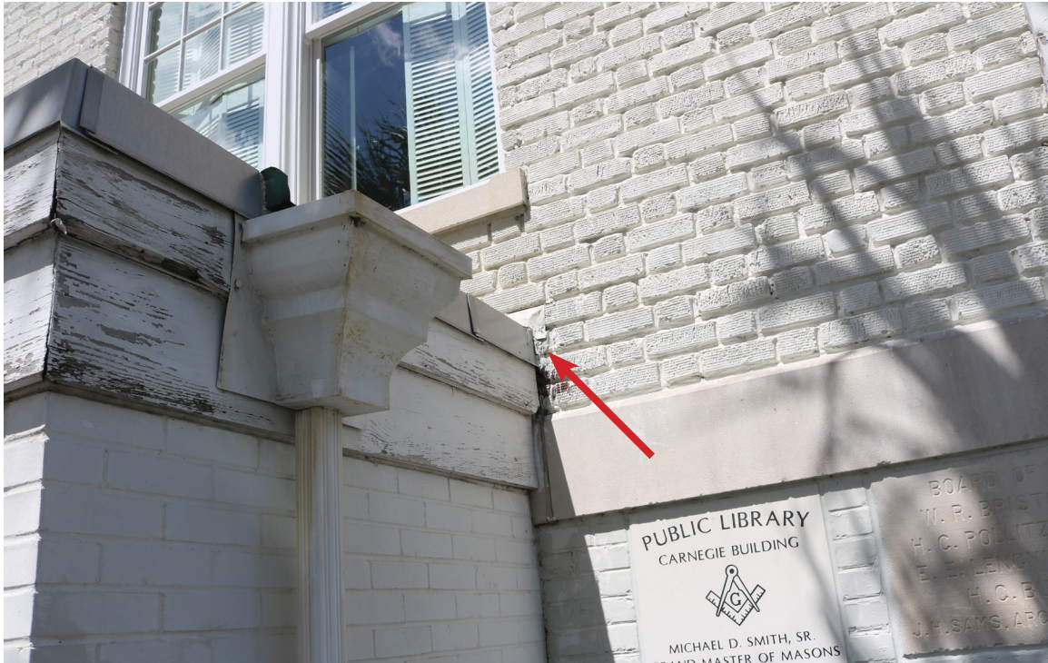
Figure 68: Beaufort Carnegie Library Building, East Addition: There is a gap between the brick masonry and the wood cornice on the addition (arrow).
