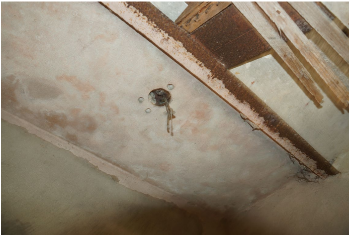
Abandoned wiring under main stairs
