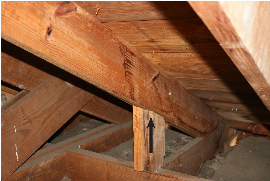
Figure 82: Beaufort Carnegie Library Building, Attic, Looking West: View of water-stained rafters to the south of the west dormer (arrow).
