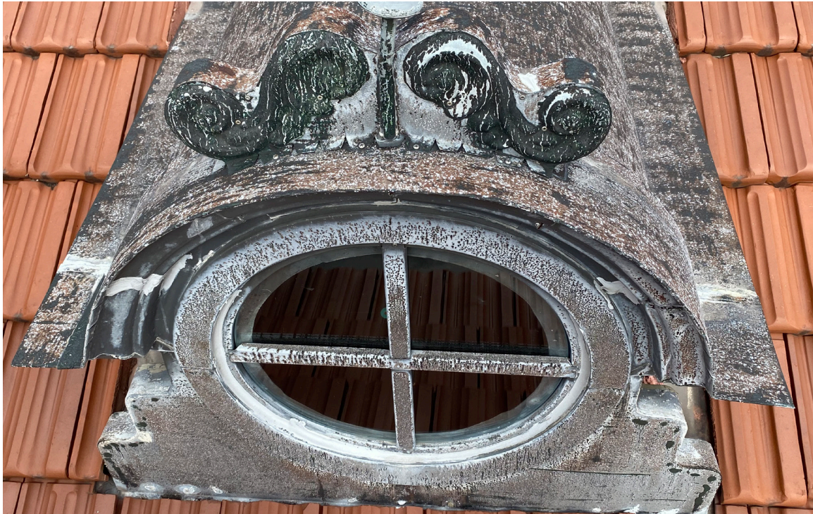
Figure 38: Beaufort Carnegie Library Building, South Elevation Dormers: East Side. View of dormer face. The metal is in good condition. The flashing between the roof and dormer is suspect.
