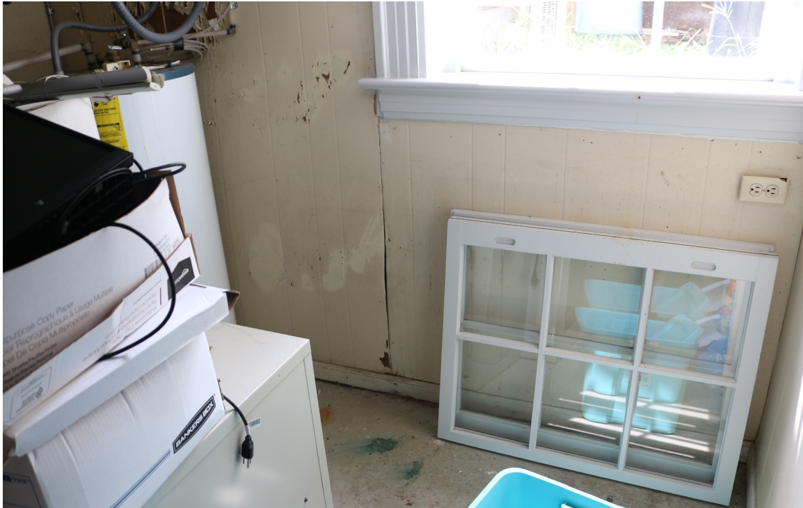
Figure 95: Beaufort Carnegie Library Building, Basement: View of paneling damage possibly caused by rising damp.
