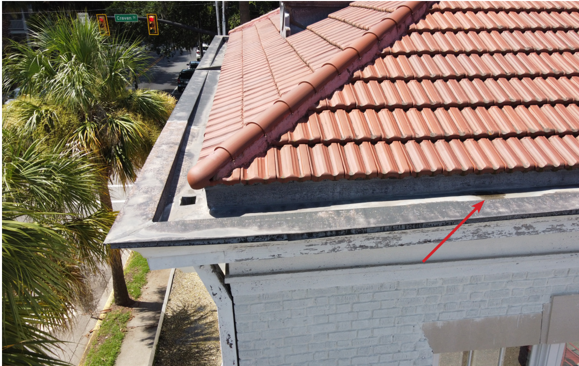
Figure 54: Beaufort Carnegie Library Building, Northeast Corner: Standing water is visible near the corner. The gutter inlet is in good condition.
