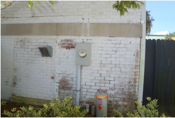
200 amp, 120/240 volt electrical service
