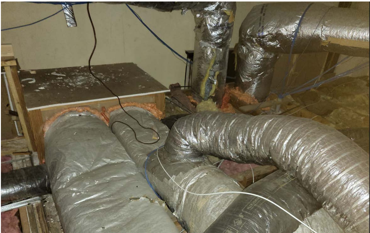
Pinched and damaged ductwork
