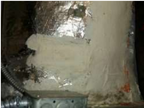
HOMOGENEOUS AREA 03 HVAC DUCT MASTIC (WHITE)
