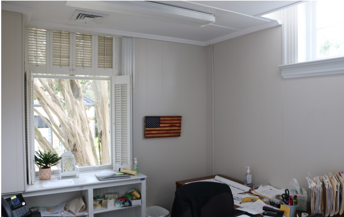
Figure 91: Beaufort Carnegie Library Building, First-Floor Offices: View the surface-mounted electrical wiring and the metal ceiling vents.
