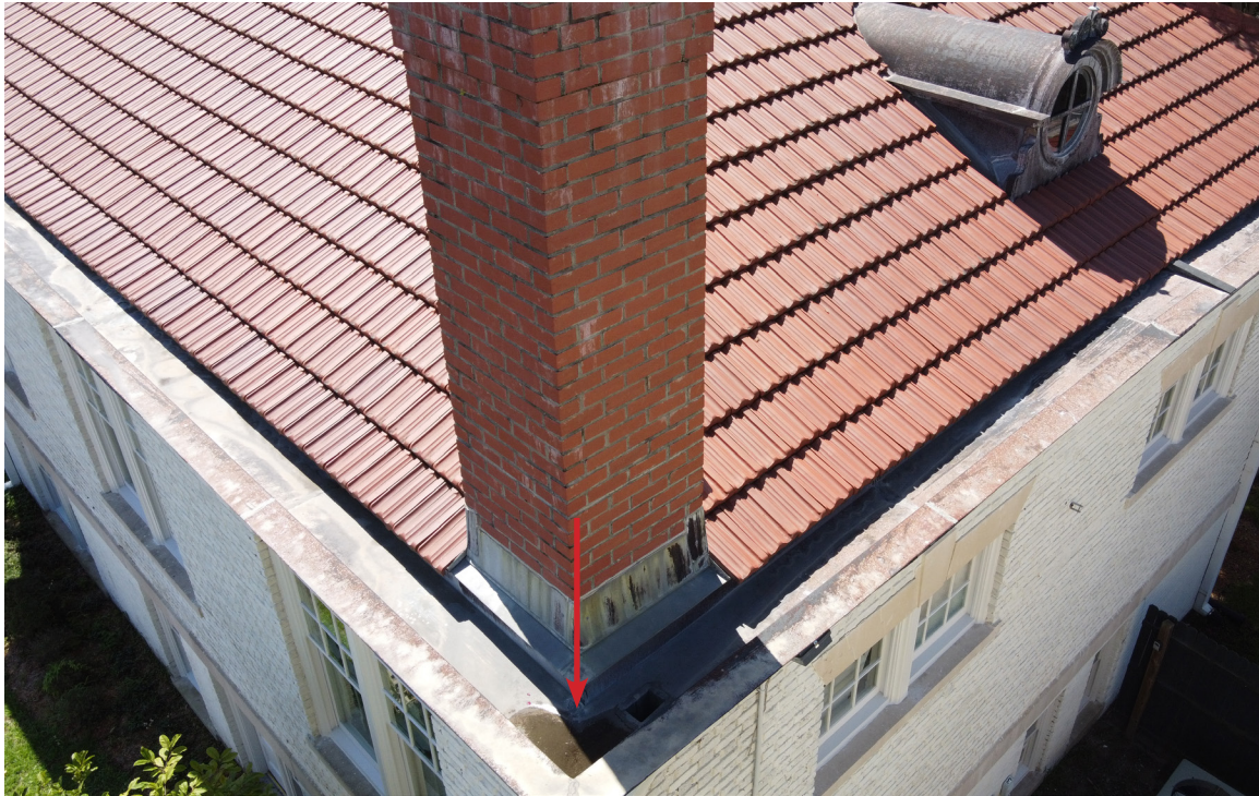
Figure 52: Beaufort Carnegie Library Building, Northwest Corner: Detail of built-in gutter at the corner. Note the standing water (arrow).
