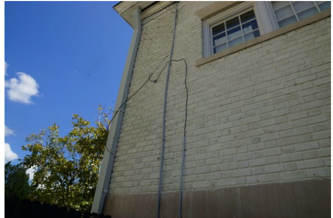
Abandoned overhead phone line and PVC conduit on building exterior
