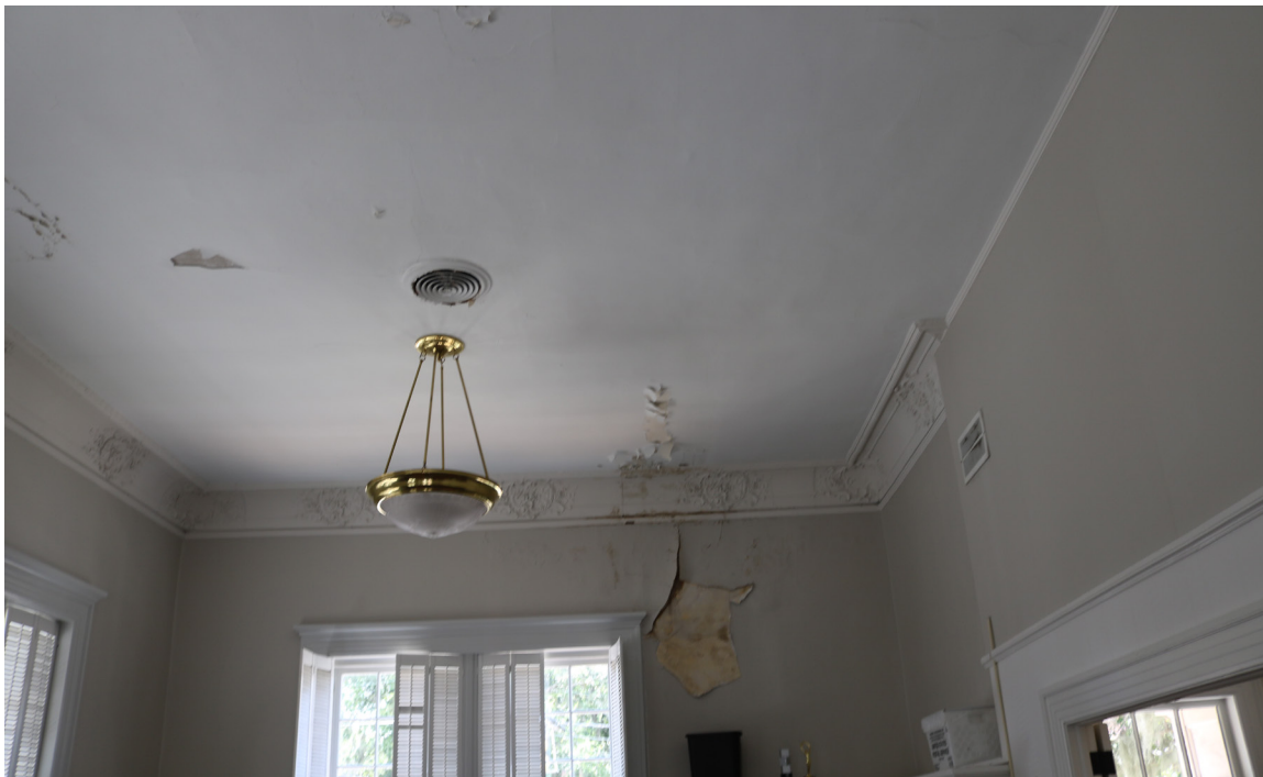
Figure 87: Beaufort Carnegie Library Building, East Conference Room: The interior plaster damage along the south wall is related to the leak at the southeast dormer.
