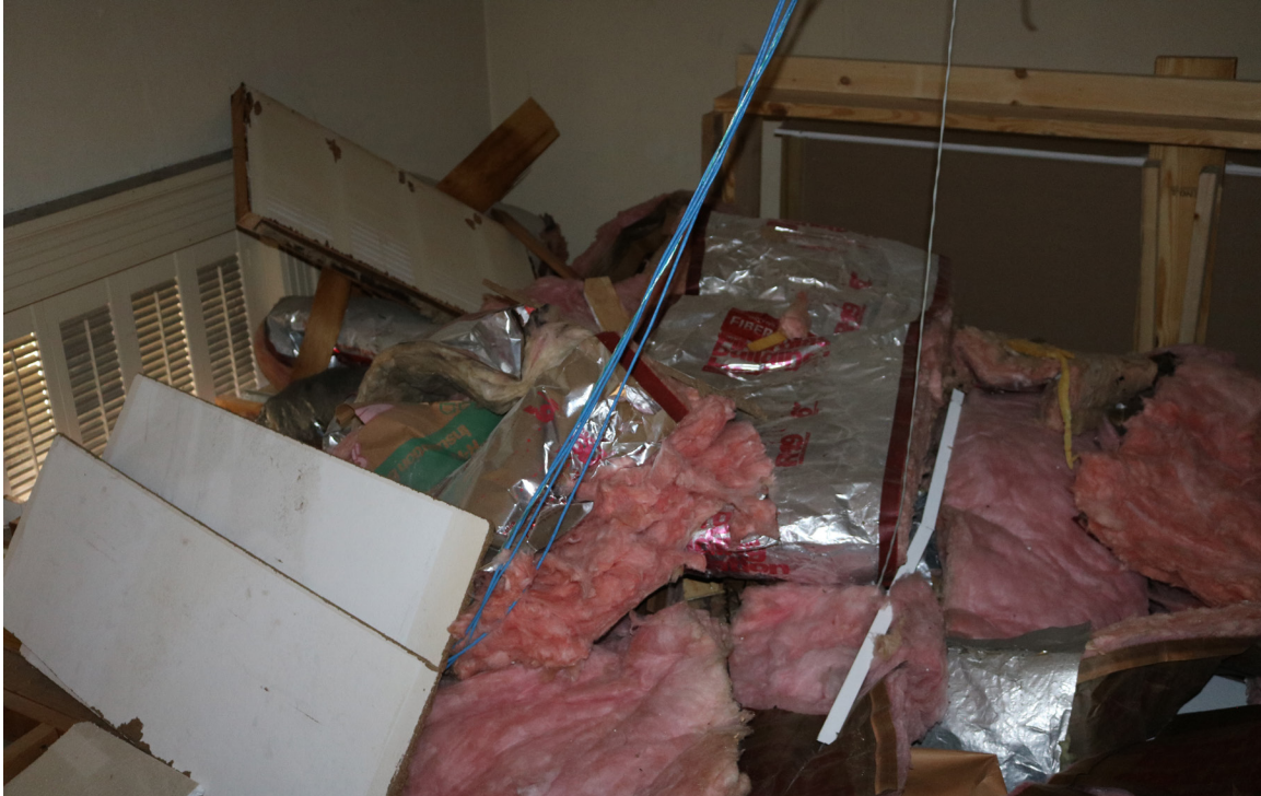
Figure 75: Beaufort Carnegie Library Building, Attic, Lower Level: View of debris and insulation present during the assessment. The debris has since been removed, but the office ceiling below is currently damaged.
