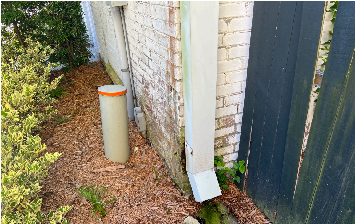
Figure 60: Beaufort Carnegie Library Building, Northwest Downspout: The downspout drains directly onto a broken splash block near the base of the building. A splashblock should be installed beneath the downspout.
