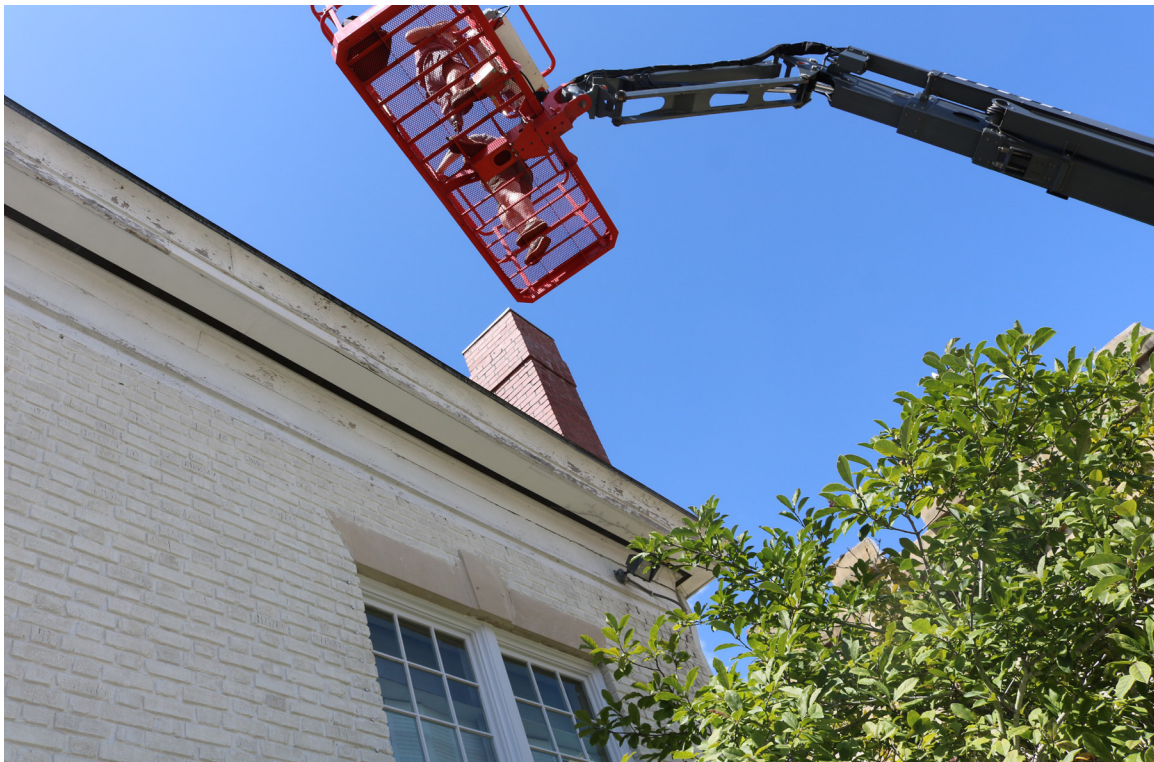
Figure 67: Beaufort Carnegie Library Building, North Facade: The cornice is in fair condition with moderate paint failure.
