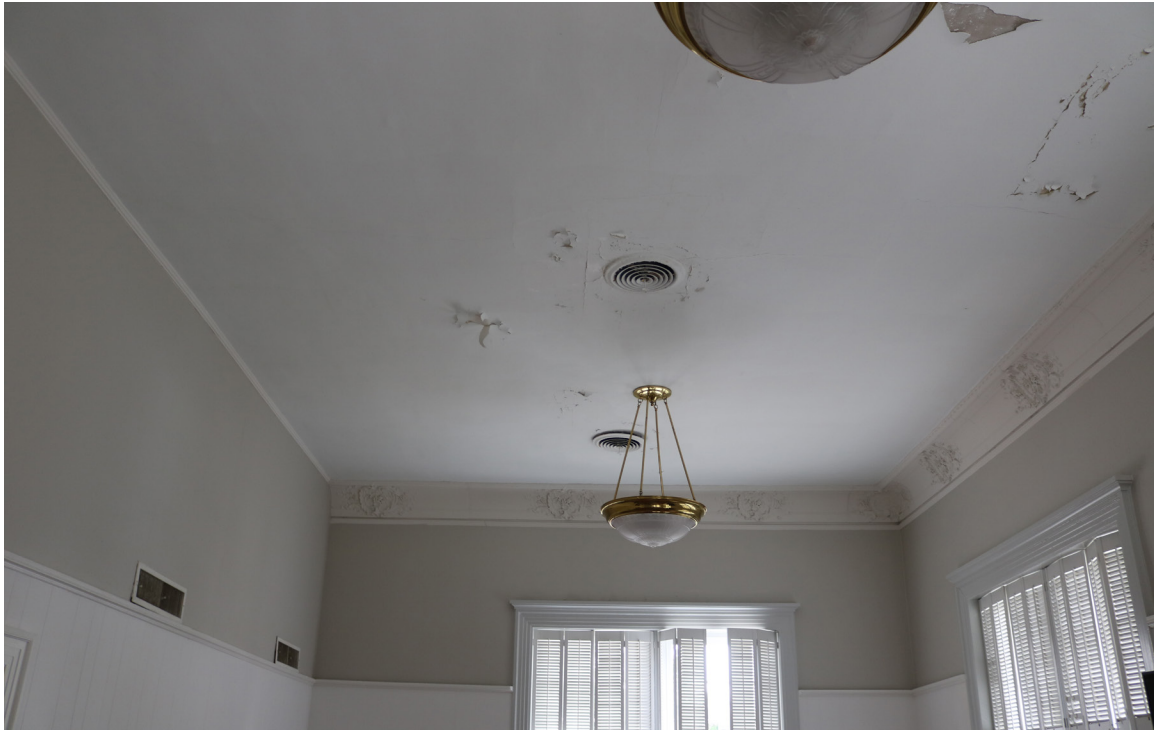
Figure 89: Beaufort Carnegie Library Building, East Conference Room: The ducts connected to the ceiling joists in this room are all disconnected from the main line in the attic.
