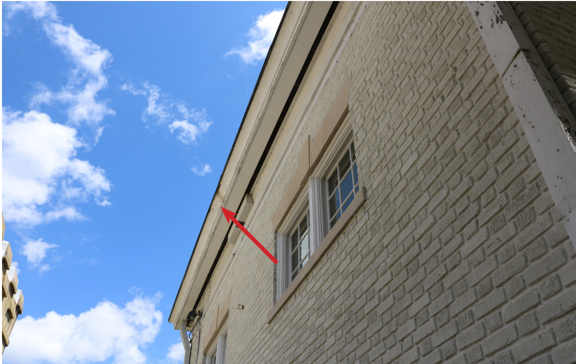
Figure 66: Beaufort Carnegie Library Building, West Facade: The cornice is damaged at the center of this elevation (arrow)
