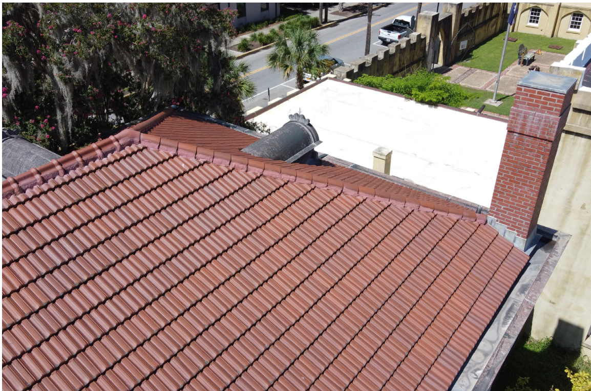
Figure 41: Beaufort Carnegie Library Building, North Elevation and Northwest Corner Chimney. Overview of roof conditions.
