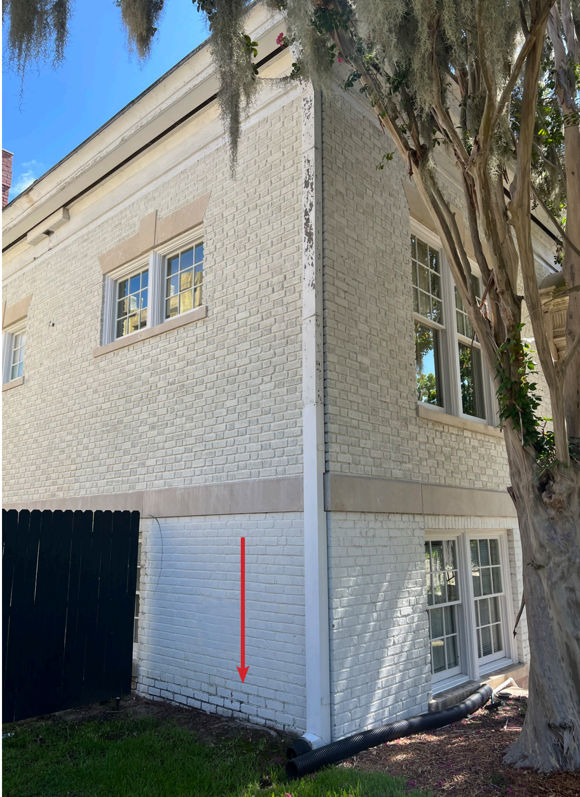
Figure 23: Beaufort Carnegie Library Building, Southwest Corner: The painted masonry is in good condition. Moderate paint loss is present at the base of the building due to rising damp (arrow).
