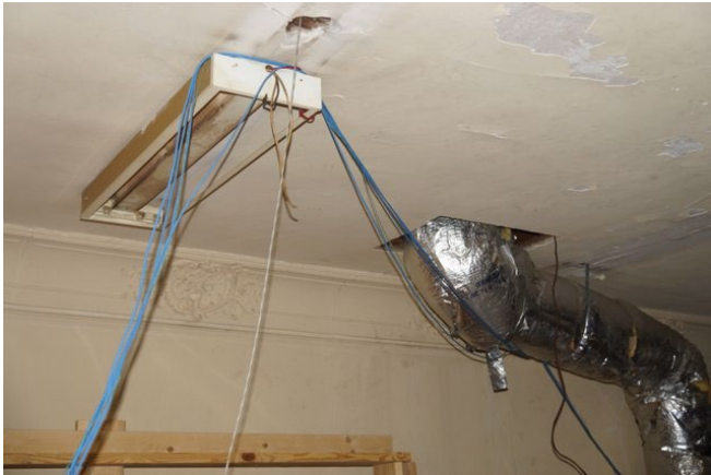
Abandoned lighting fixtures and IT wiring in attic
