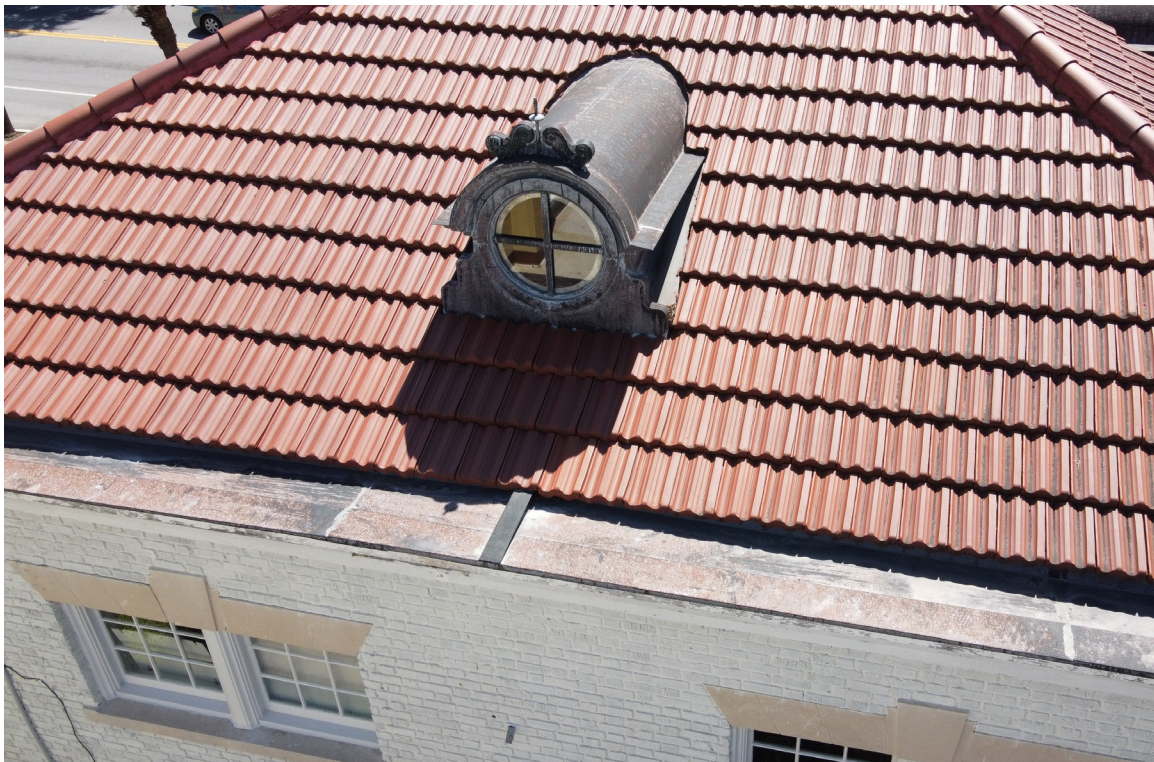
Figure 47: Beaufort Carnegie Library Building, West Dormer. This dormer does not appear to leak, but all the dormer flashing is suspect.
