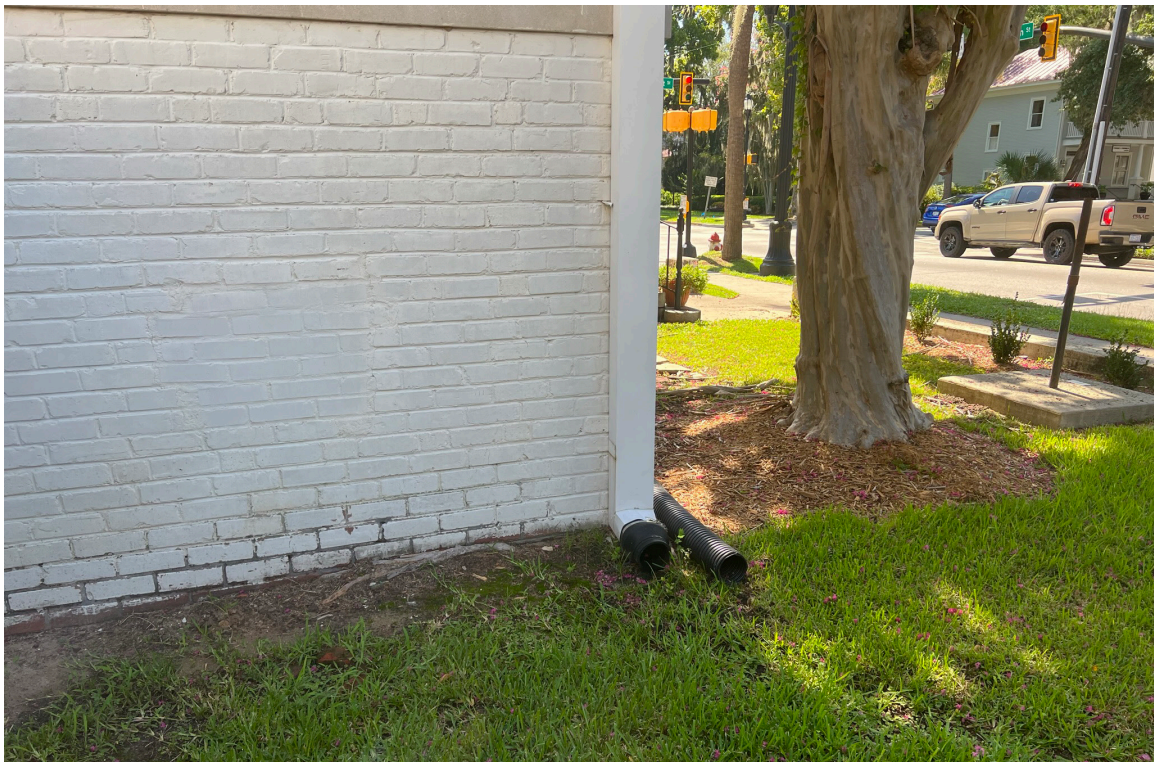
Figure 59: Beaufort Carnegie Library Building, Southwest Downspout: The downspout extender is disconnected, allowing water to drain near the foundation of the building. Both downspouts on the south elevation can be directed underground to drain through a nozzle in the perimeter wall.
