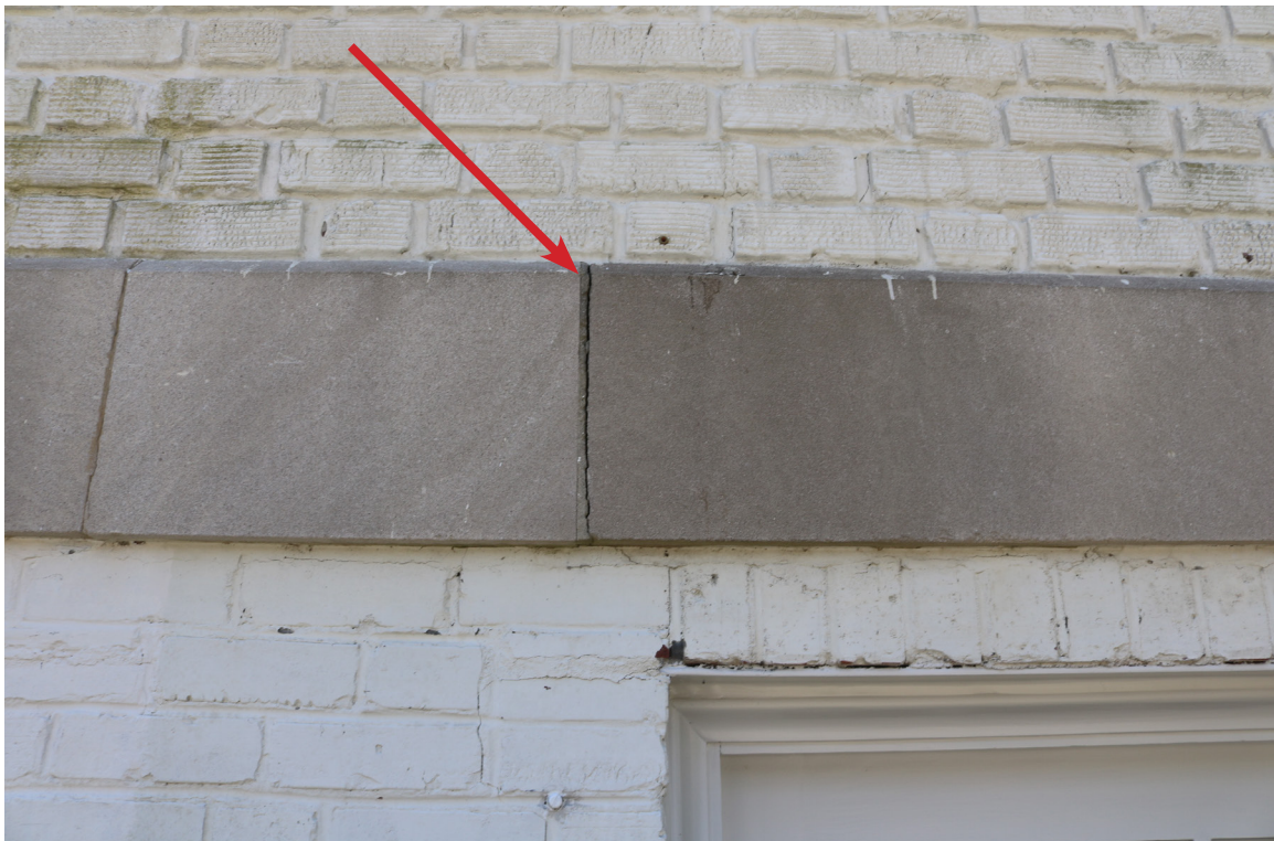
Figure 27: Beaufort Carnegie Library Building, North Elevation: The limestone belt course has isolated mortar loss (arrow).
