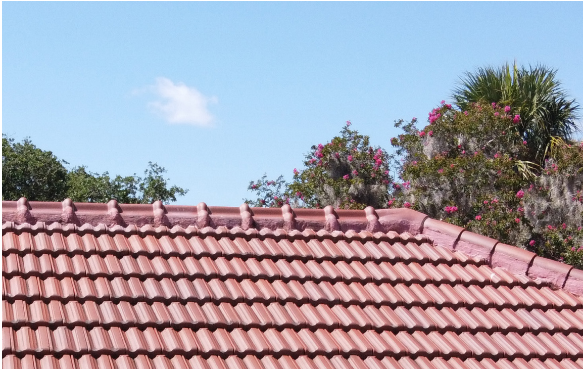
Figure 42: Beaufort Carnegie Library: Roof Ridge. The mortar is releasing from the ridge tiles.
