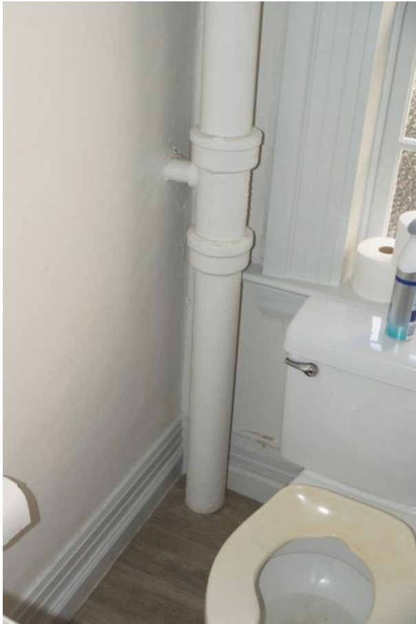
Cast iron waste pipe
