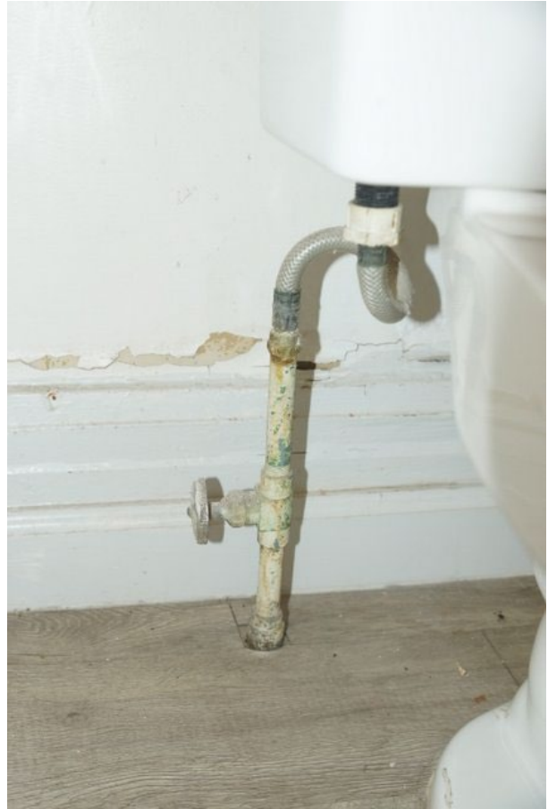
Copper water supply piping
