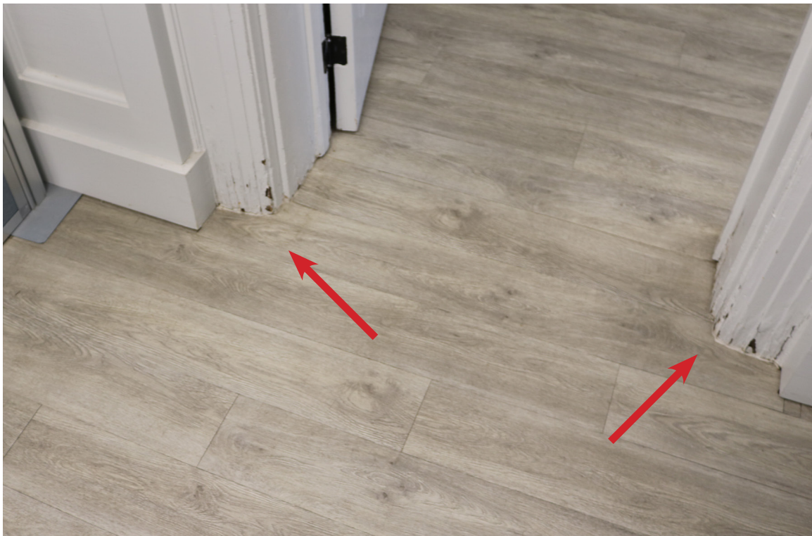
Figure 96: Beaufort Carnegie Library Building, Basement Offices: View of paint finish failure and bubbling on the lower casing (arrows). This may be caused by moisture.
