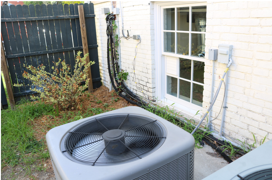
Figure 25: Beaufort Carnegie Library Building, West Elevation at Ground Level: Vines commonly grow on the building at this corner. Note paint damage from rising damp.
