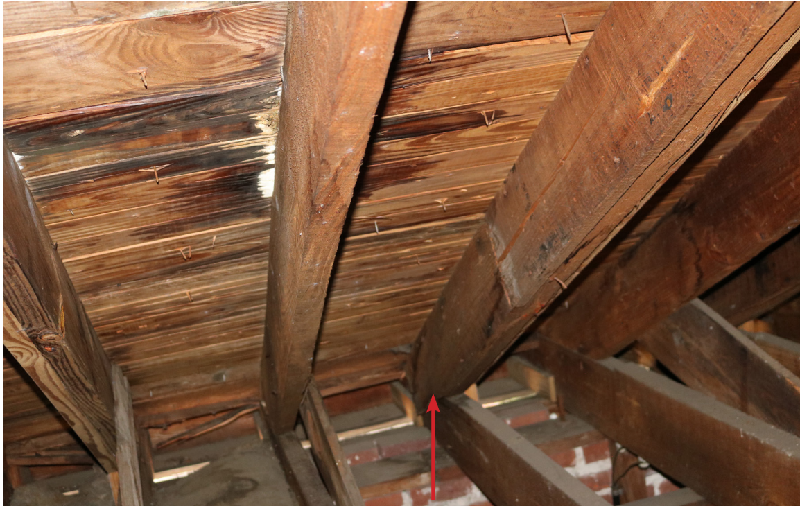
Figure 85: Beaufort Carnegie Library Building, Attic, Looking South. The end of one joist has deteriorated below the south dormers (arrow). White mold from an active leak is visible above.
