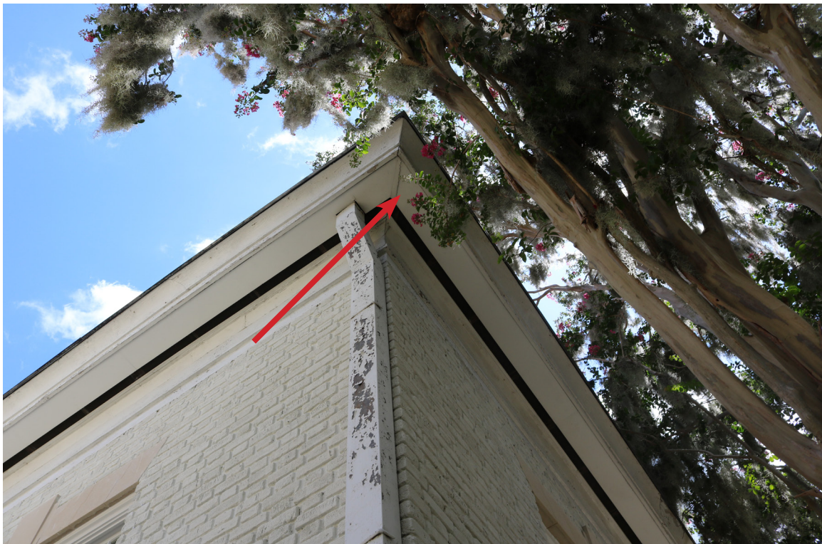
Figure 65: Beaufort Carnegie Library Building, Southwest Corner: The woodwork is beginning to separate at this corner.
