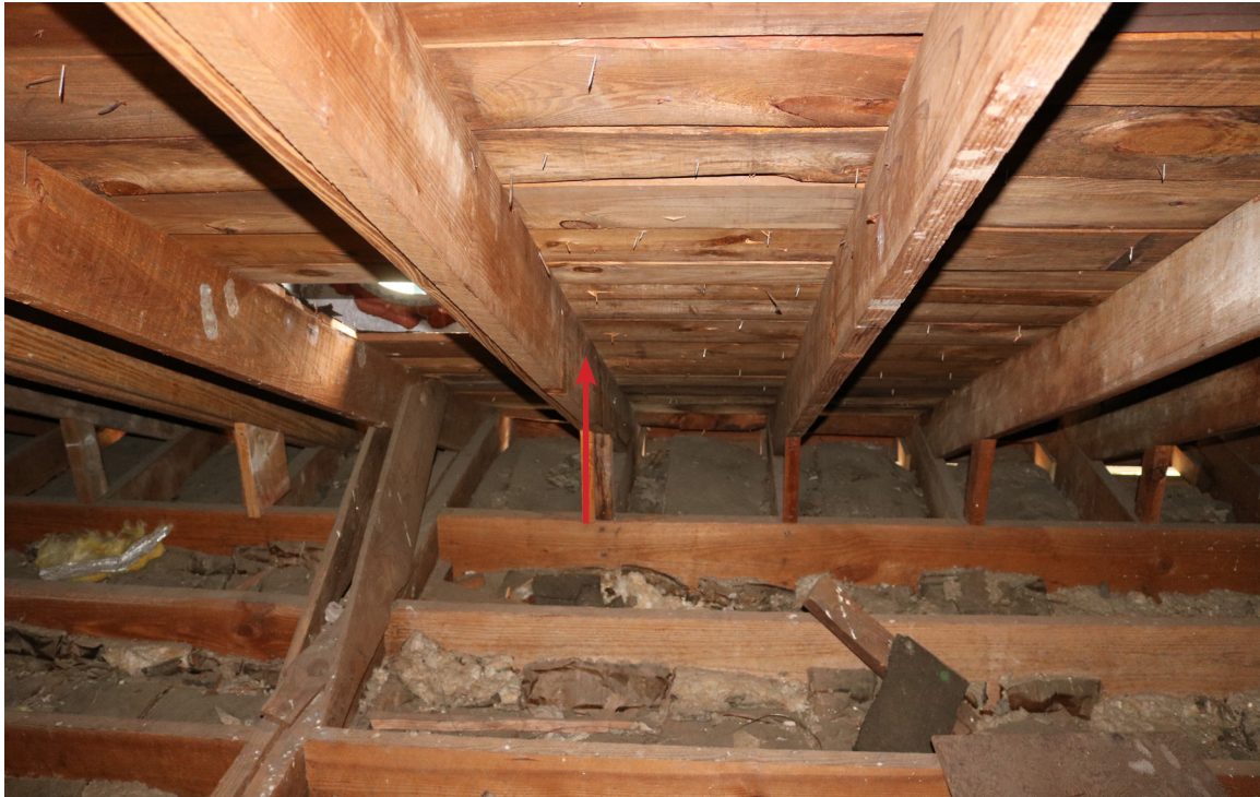
Figure 81: Beaufort Carnegie Library Building, Attic, Looking West: View of deteriorated sheathing to the south of the west dormer (arrow). The ceiling damage below this location is related to the leaking gutters.
