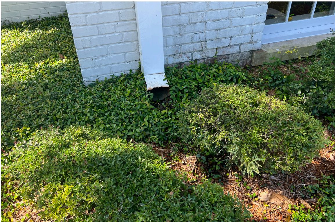
Figure 61: Beaufort Carnegie Library Building, Northeast Downspout: This downspout drains onto the garden bed, which appears to slope away from the building. A splashblock should be installed at this location.
