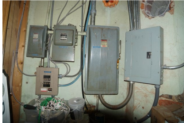
Main electrical equipment
