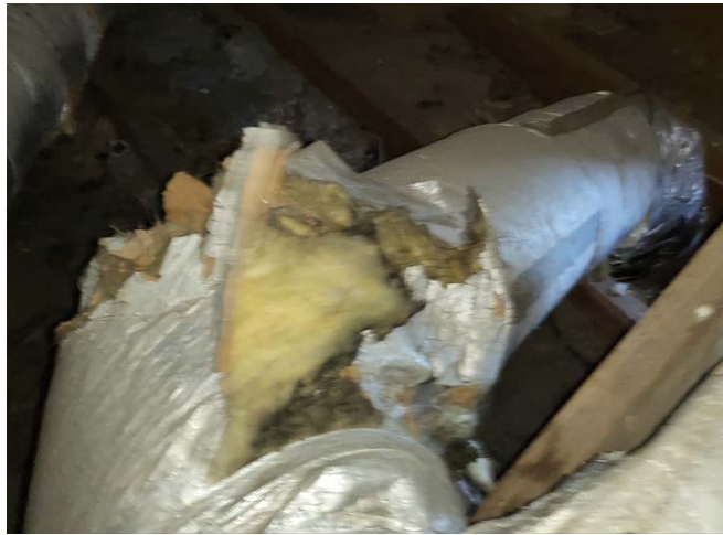
Damaged duct insulation
