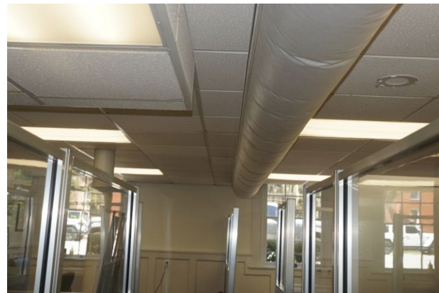
General lighting ground floor
