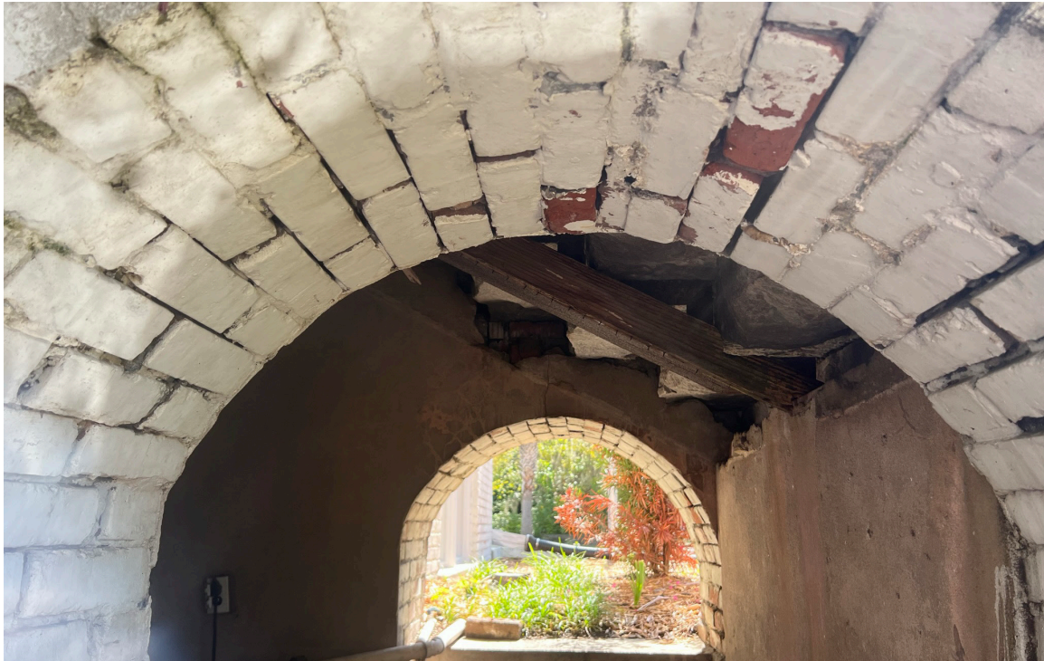
Figure 19: Beaufort Carnegie Library Building, Historic Basement Entrance: View of the masonry beneath the granite treads. A plaster ceiling was once installed at this location. Several cracks are present in the masonry arch, and the treads have settled.
