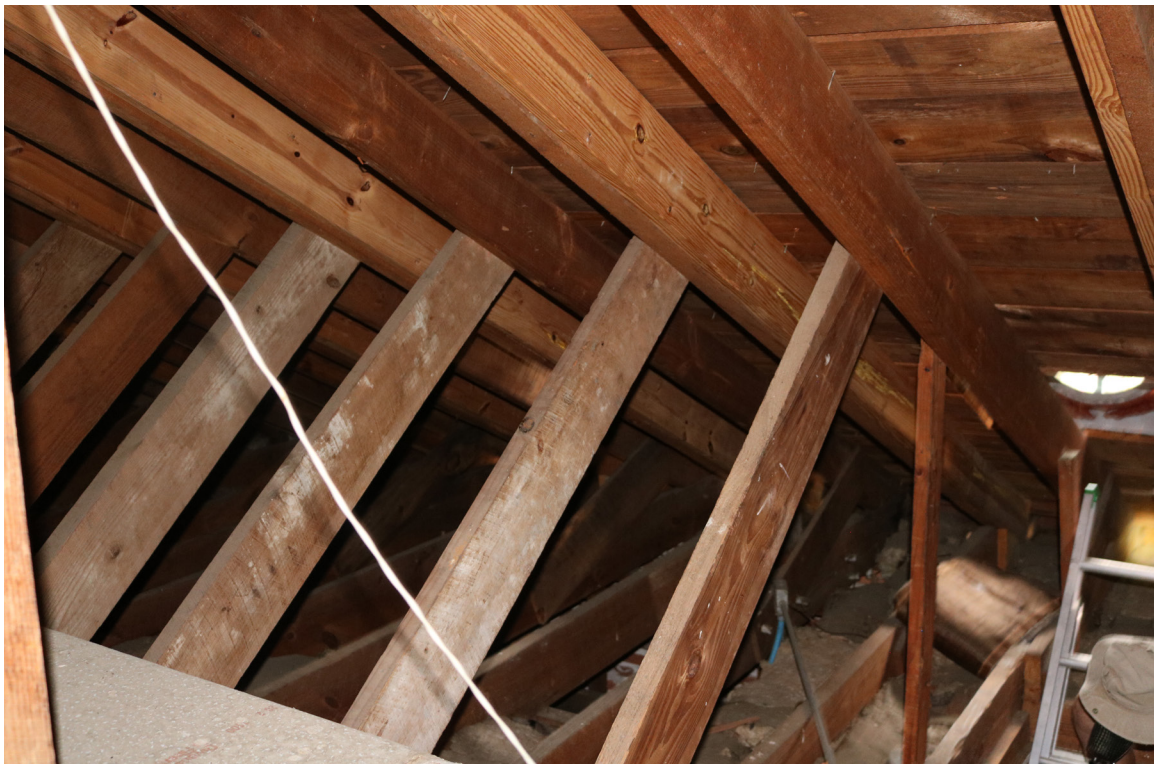
Figure 84: Beaufort Carnegie Library Building, Attic Ridge: The rafters are in good condition.
