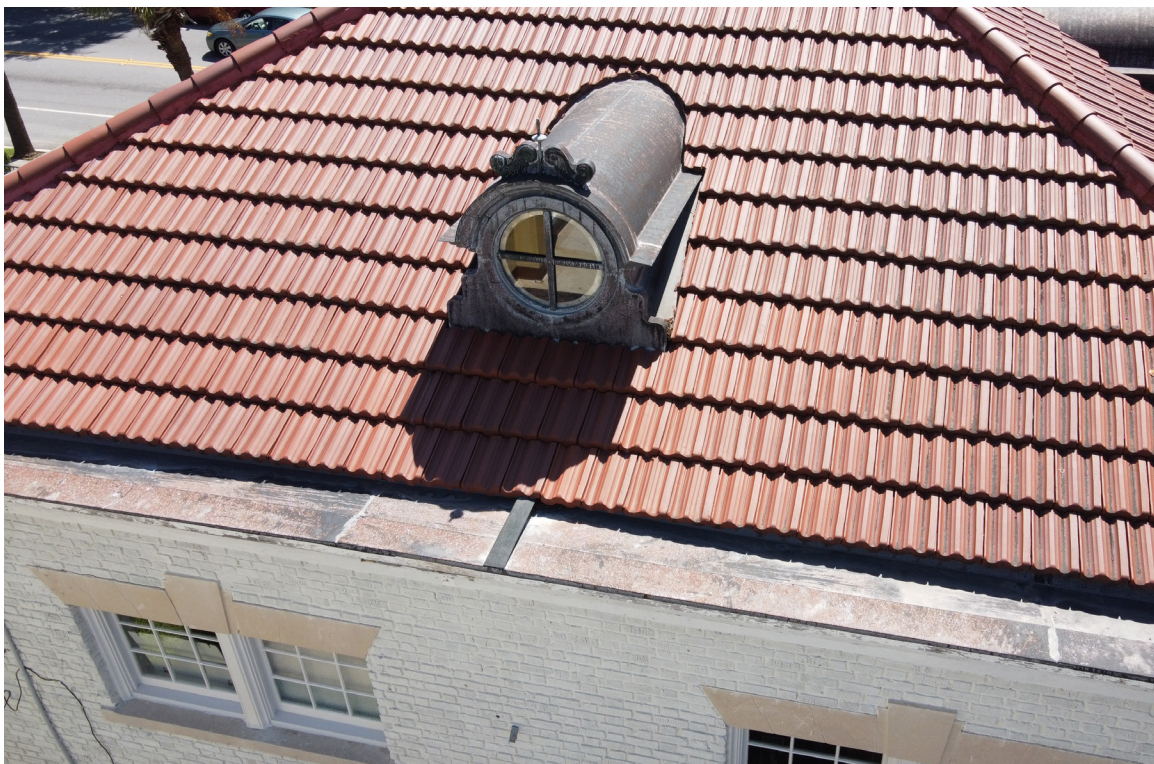
Figure 51: Beaufort Carnegie Library Building, West Elevation: Detail of built-in gutter on this side of the building. The gutter appears to be in good condition.
