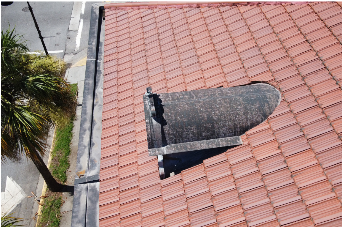
Figure 39: Beaufort Carnegie Library Building, East Elevation Dormer: The dormers are ca. 2000 recreations constructed from lead-coated copper. Red and black lead sulfides have formed on the metal's exterior surface, creating a mottled finish.
