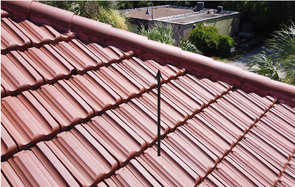
Figure 44: Beaufort Carnegie Library Building, View of Hip Caps. View of cracked mortar.
