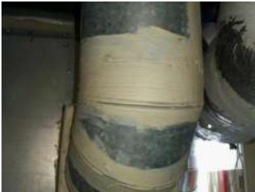
HOMOGENEOUS AREA 11 HVAC DUCT MASTIC (BEIGE)
