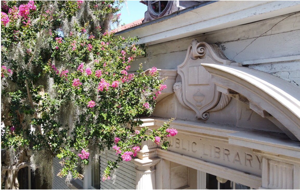
Figure 64: Beaufort Carnegie Library Building, South Entrance: The cornice is in good condition, but the adjacent tree is in direct contact with the wooden elements.
