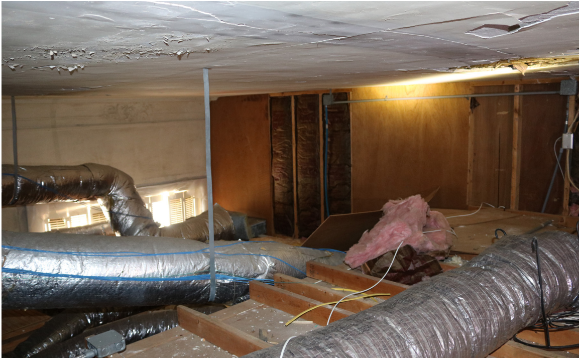
Figure 73: Beaufort Carnegie Library Building, Attic, Lower Level Looking Southwest: View of the attic's lower level directly above the office ceilings.
