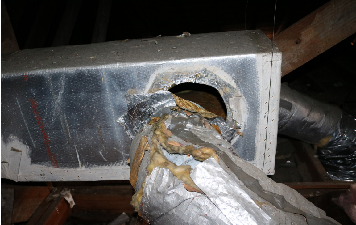
Figure 77: Beaufort Carnegie Library Building, Attic, Upper Level: The HVAC lines were disconnected from the main line. These ducts feed the ceiling vents in the large conference room.
