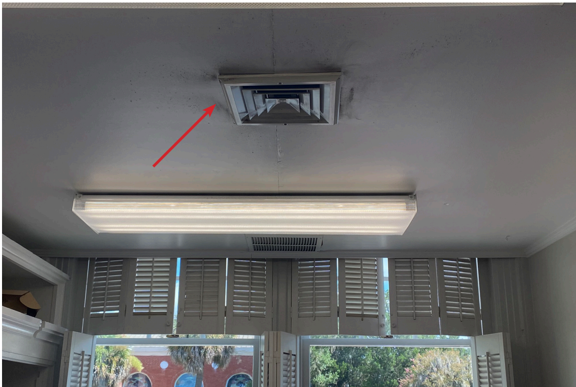
Figure 92: Beaufort Carnegie Library Building, First Floor: View of mold growth around the metal ceiling vents (arrow).
