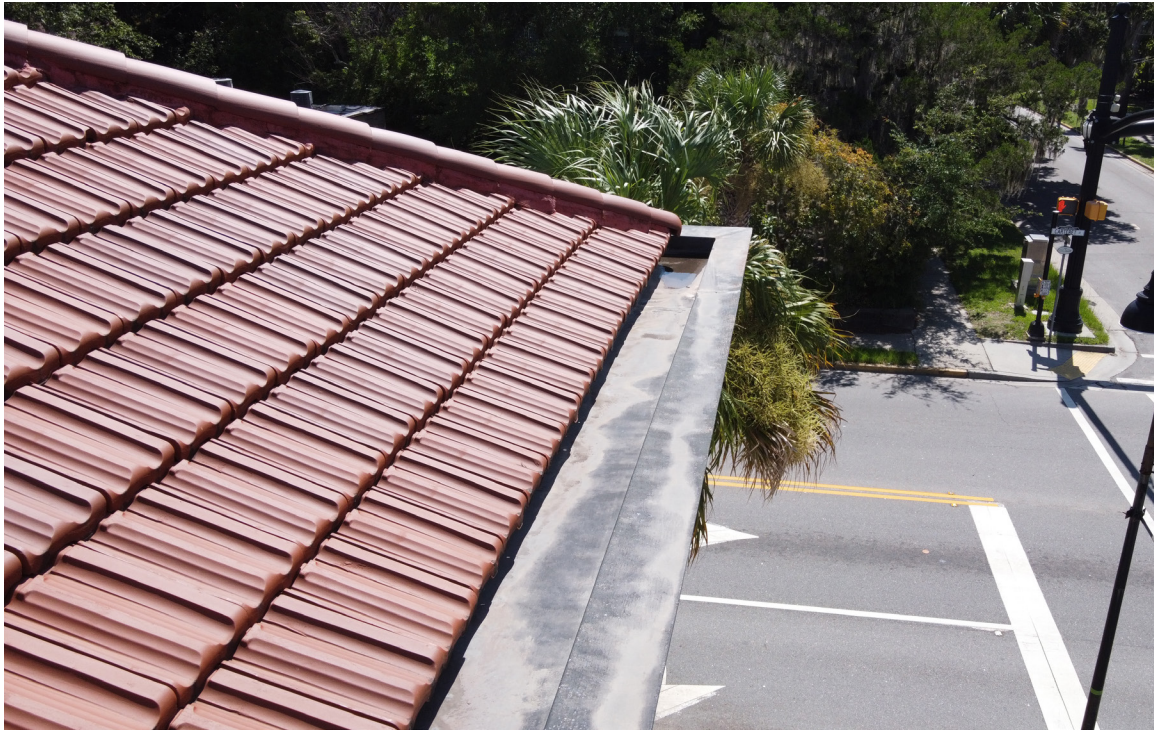
Figure 50: Beaufort Carnegie Library Building, South Elevation, Looking East: Detail of standing water at the southeast corner.
