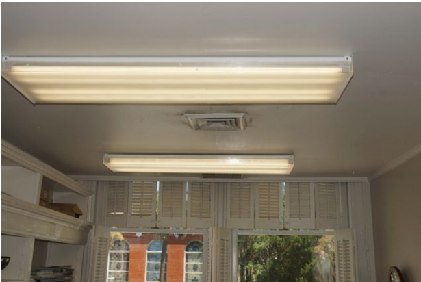
General lighting main floor
