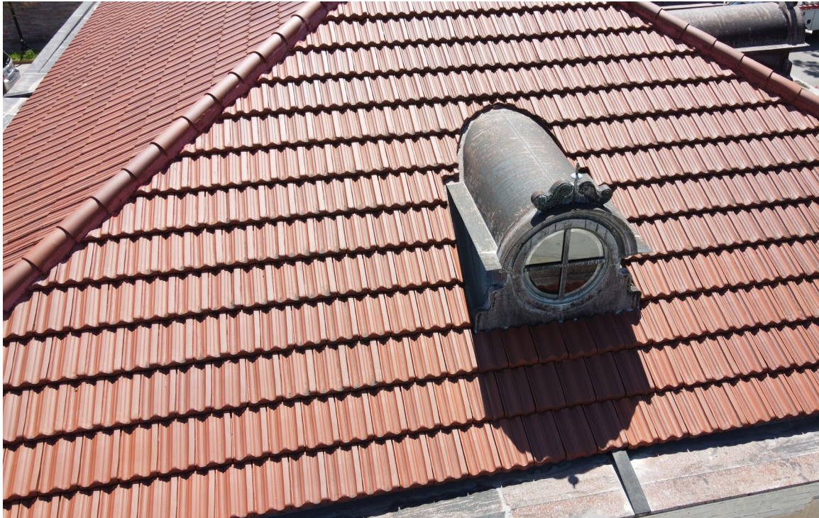
Figure 40: Beaufort Carnegie Library Building, East Elevation Dormer. This dormer also actively leaks on the south side.
