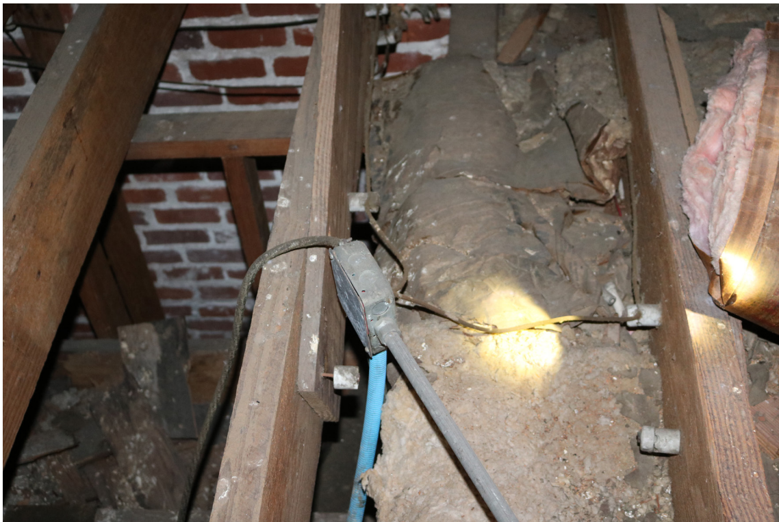
Figure 86: Beaufort Carnegie Library Building, Attic Ceiling Joists: Knob and tube wiring was found spliced into a modern conduit.
