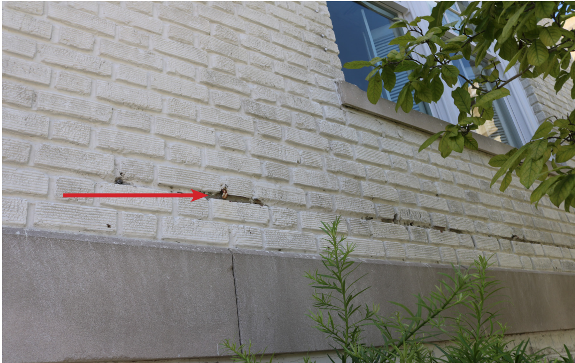
Figure 28: Beaufort Carnegie Library Building, North Elevation, West Side: View of abandoned fasteners and missing paint in an area where a pipe was removed (arrow).
