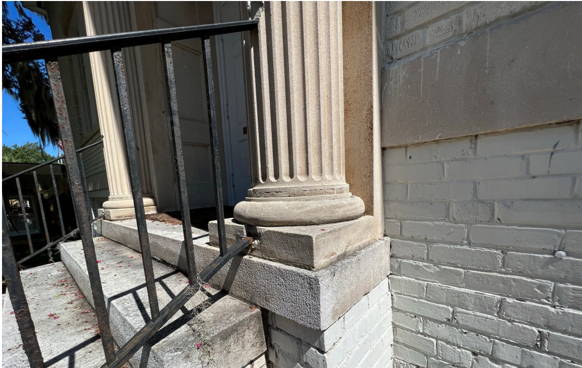
Figure 16: Beaufort Carnegie Library Building, Front Entrance: View of the carved limestone entrance. Mortar loss and stone damage are visible.
