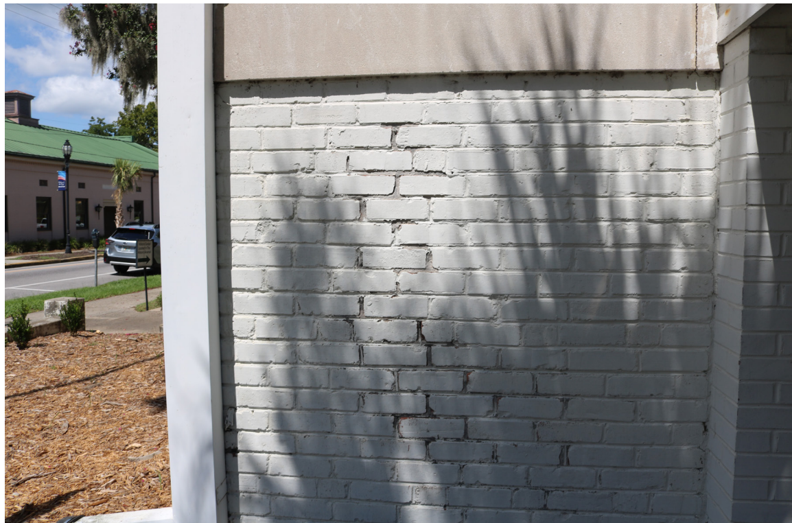
Figure 33: Beaufort Carnegie Library Building, Southeast Corner. Detail of paint loss due to rising damp.
