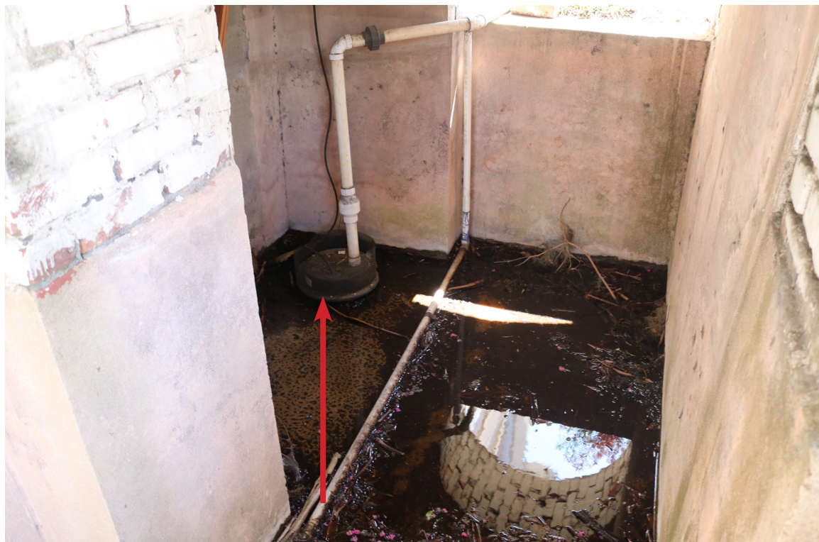
Figure 20: Beaufort Carnegie Library Building, Historic Basement Entrance: View of ponding and the dam created by the irrigation line. The sump pump appears to have been installed higher than the concrete floor (arrow).
