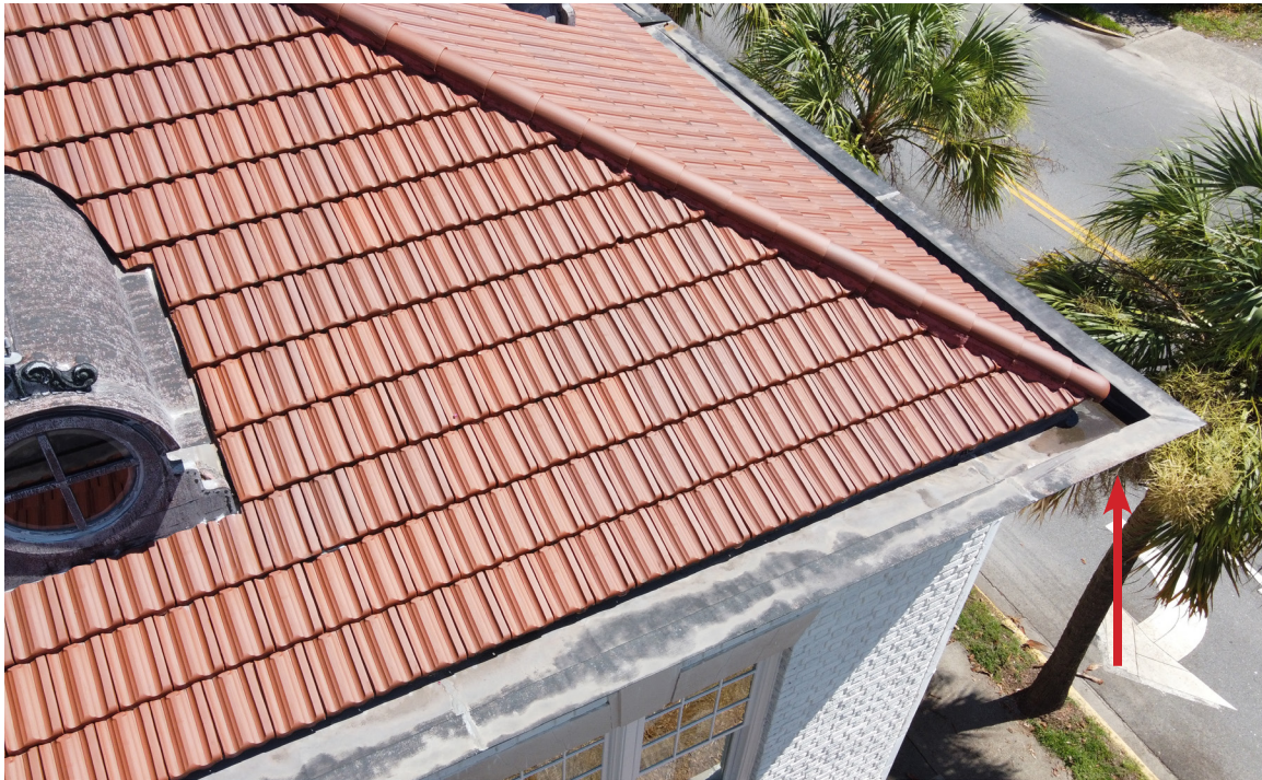
Figure 48: Beaufort Carnegie Library Building, South Elevation, Southeast Corner: The built-in gutter ponds at this corner (arrow). The soffit has deteriorated beneath, indicating there is an active leak.
