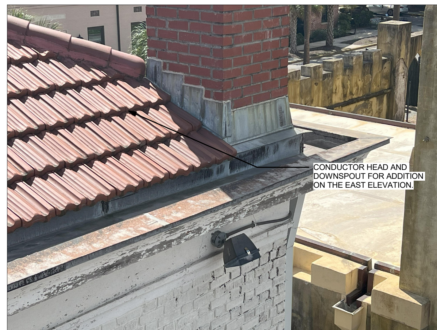
EXISTING CONDITIONS- VIEW AT NORTHWEST CORNER, DETAILED VIEW OF CHIMNEY PENETRATION AT ROOF.
