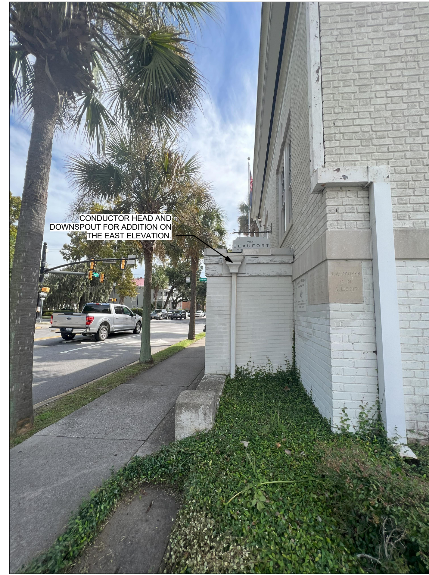
EXISTING CONDITIONS- NORTHEAST CORNER DOWNSPOUT. DOWNSPOUT AND CONDUCTOR/LEADER HEAD AT THE SIDE ADDITION CAN BE SEEN IN THE BACKGROUND.
