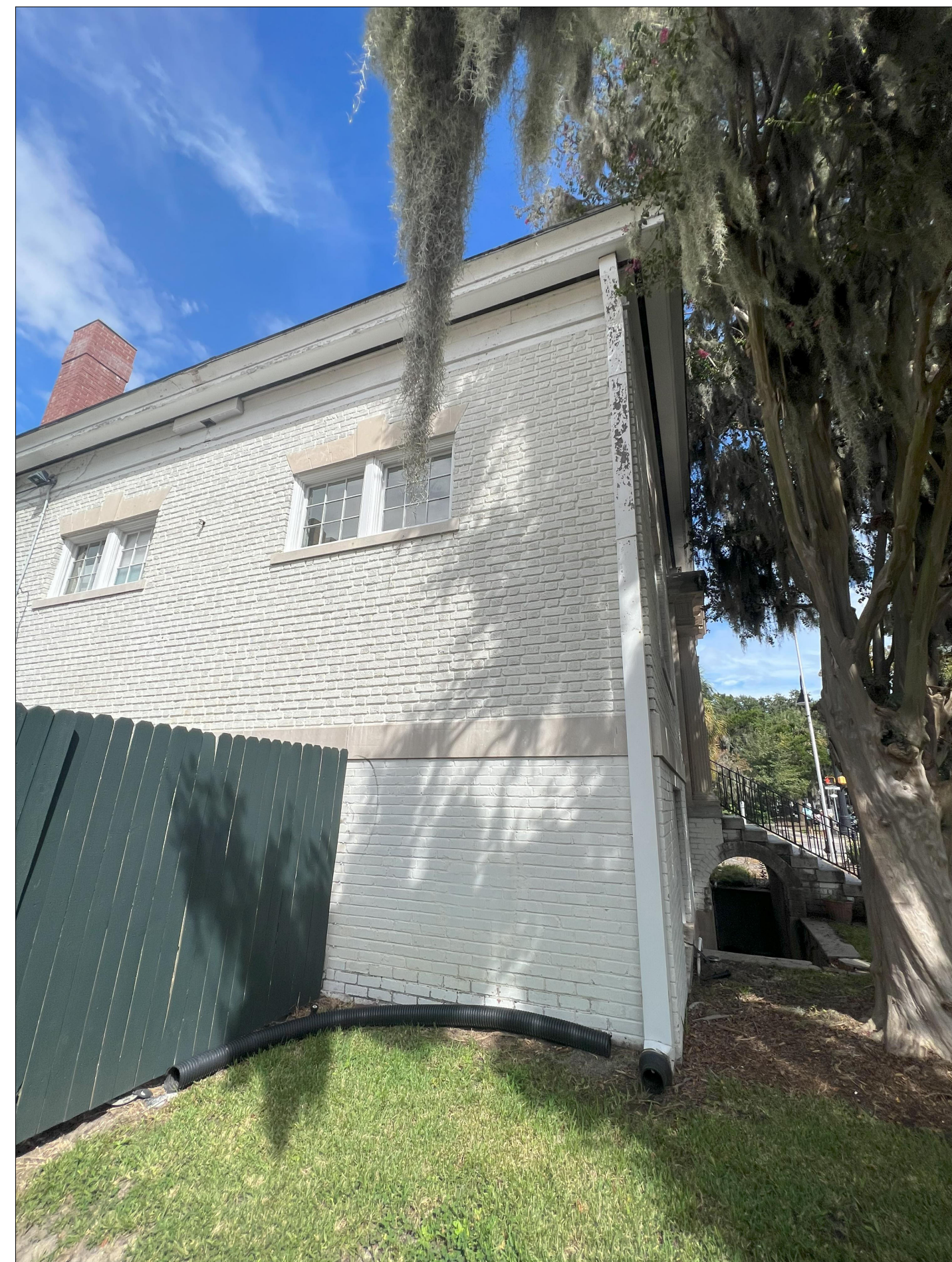
EXISTING CONDITIONS- SOUTHWEST CORNER DOWNSPOUT.
