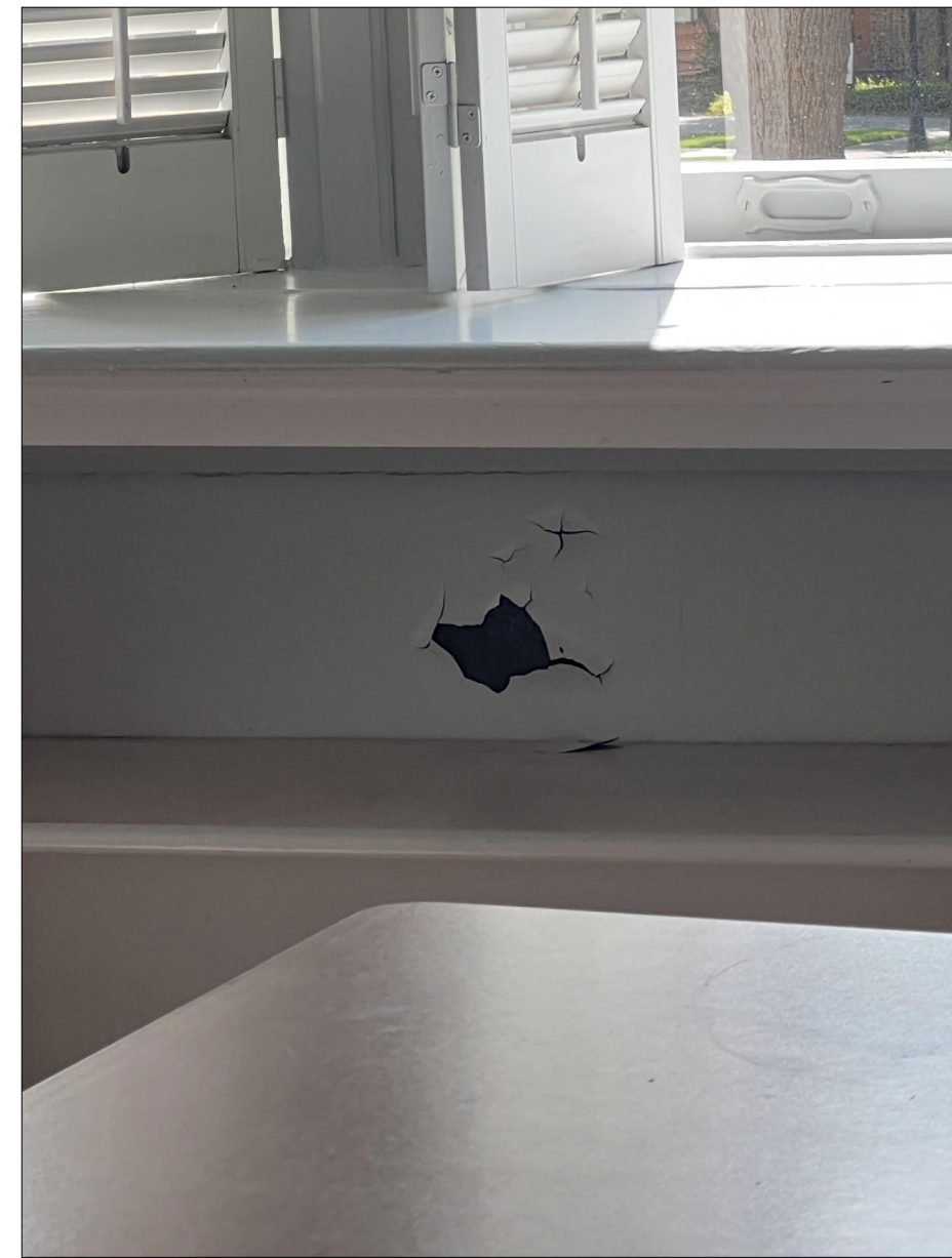
DETAIL PHOTO OF CRACKED PAINT BELOW WINDOWS 14 & 15, TYPICAL CONDITION BELOW WINDOWS.
