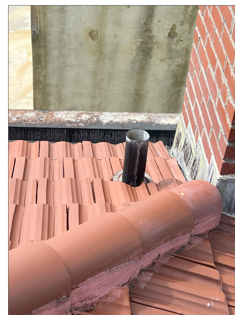
EXISTING CONDITIONS- VIEW AT NORTHWEST CORNER, DETAILED VIEW OF RIDGE AND VENT.
