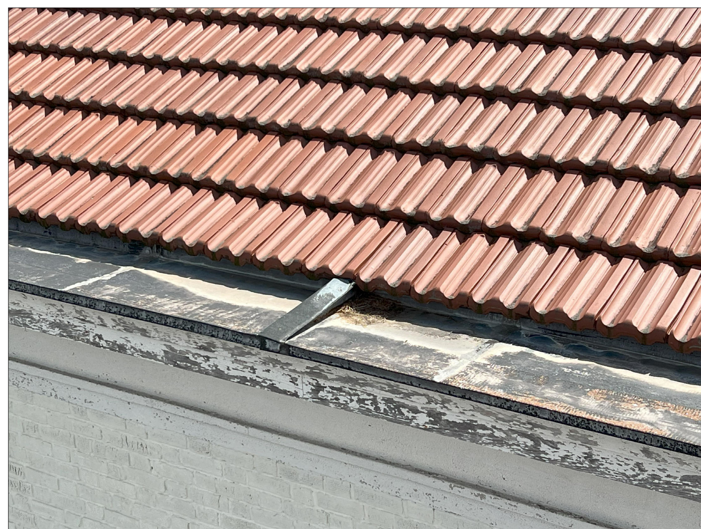
EXISTING CONDITIONS- VIEW LOOKING SOUTH, DETAILED VIEW OF BUILT IN GUTTER AND FRENCH TERRACOTTA TILES.
