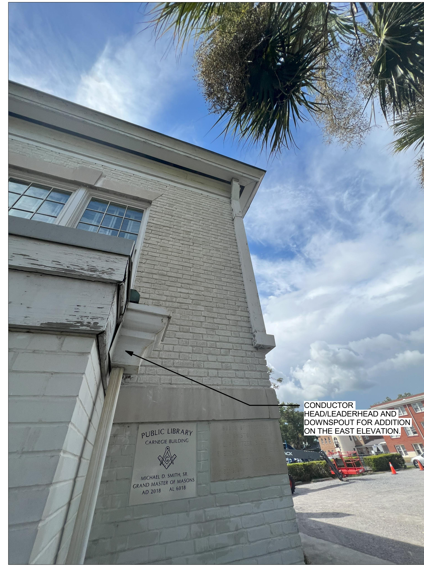
EXISTING CONDITIONS- DOWNSPOUTS ON NORTH SIDE OF THE EAST ELEVATION. CONDUCTOR HEAD/LEADERHEAD ON THE LEFT IS PART OF THE WATER DRAINAGE SYSTEM FOR THE ADDITION ROOF.
