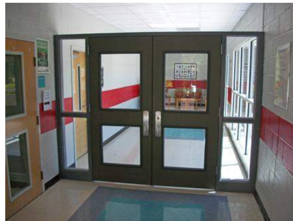
NEW DOUBLE SECURITY DOOR ASSEMBLY (SIMILAR TO ABOVE) (COLOR TO BE SELECTED BY OWNER)
