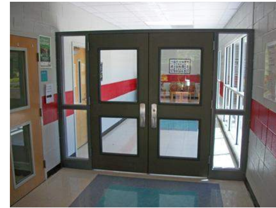
NEW DOUBLE SECURITY DOOR ASSEMBLY (SIMILAR TO ABOVE) (COLOR TO BE SELECTED BY OWNER)
