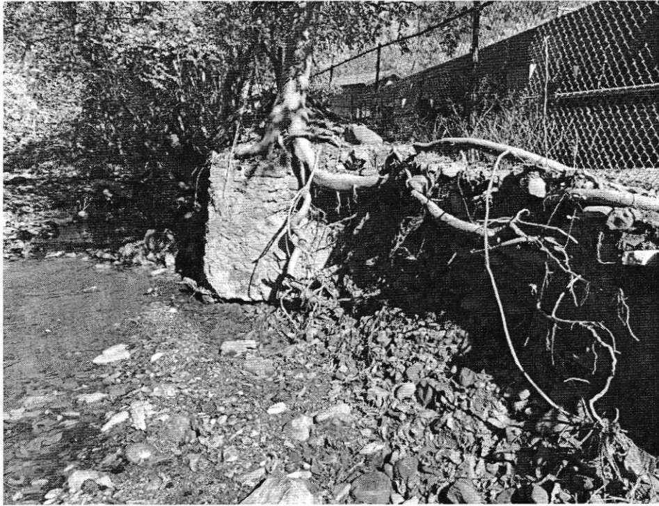
Photo 1: The upper-most section of bank needing stabilization.
