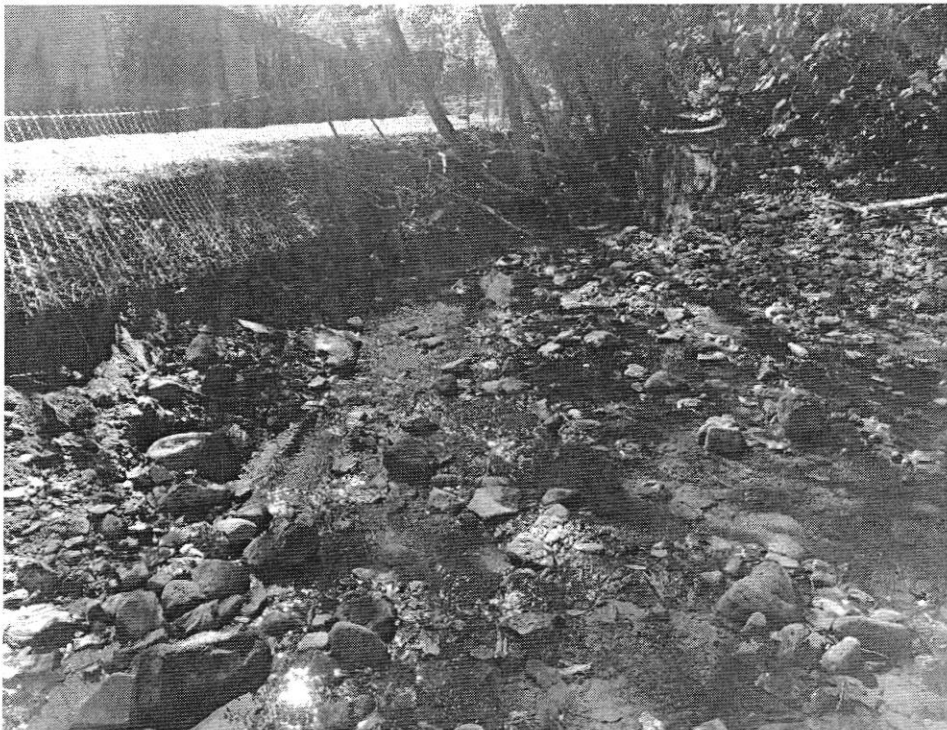
Photo 2: Middle Creek has encroached towards the school, and is now within 25 feet of the main building.
