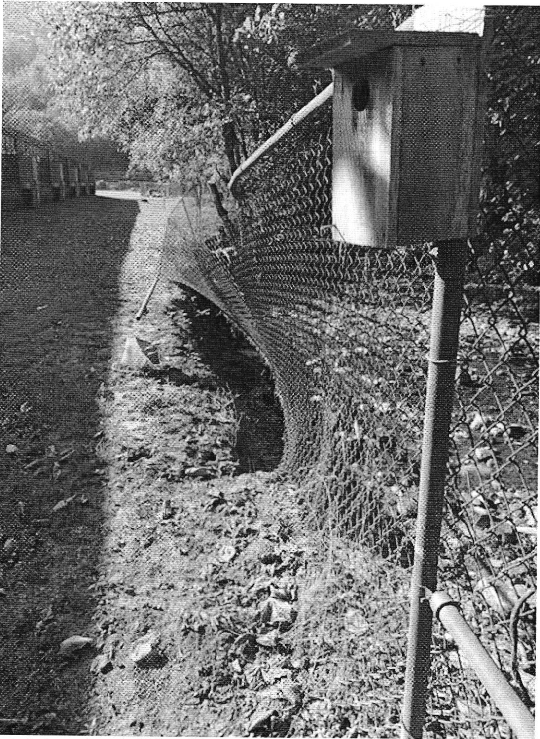
Photo 3: Approximately 75 feet of fencing has been undermined from scouring flood events.
