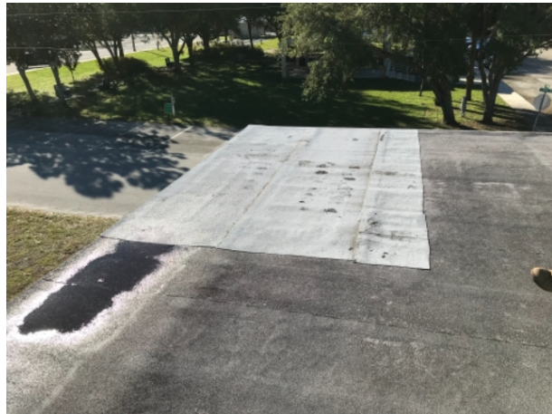
Observation Se and NE corners tore off and deck and roofing replaced. Will require additional attachment through top of modified prior to new roof installation
