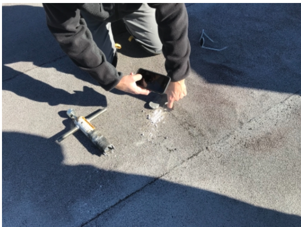
Observation Core cut at loose area of modified Attached to Gypsum deck. Additional attachment will be needed in these areas prior to reroofing
