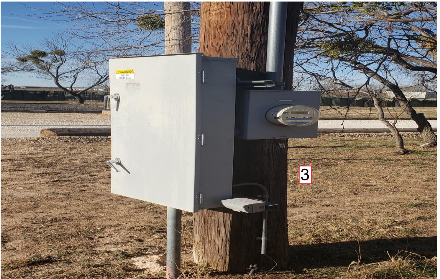
FIO - Construct New FOB North - Existing Electrical Panel and Meter
