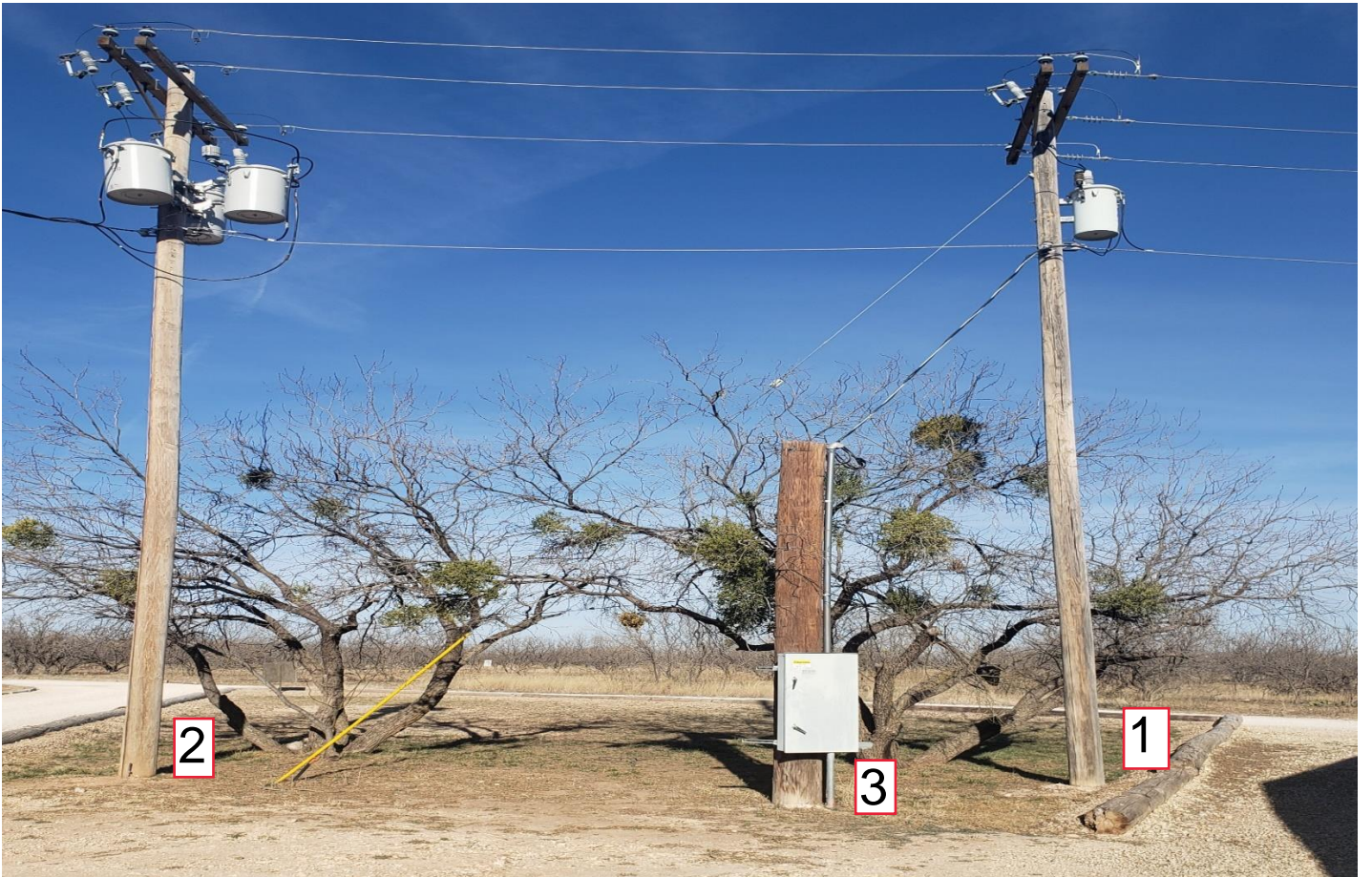
FIO - Construct New FOB North - Existing Power Poles
