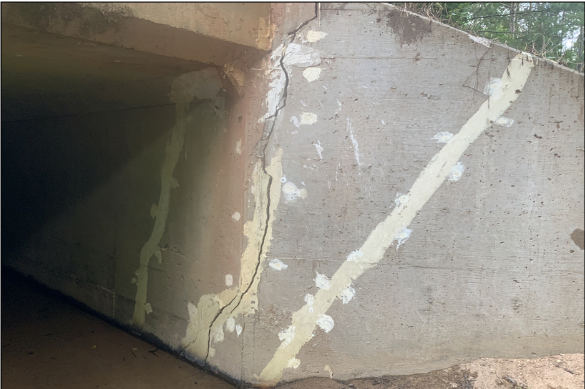
Cracking in the forward outlet wing
