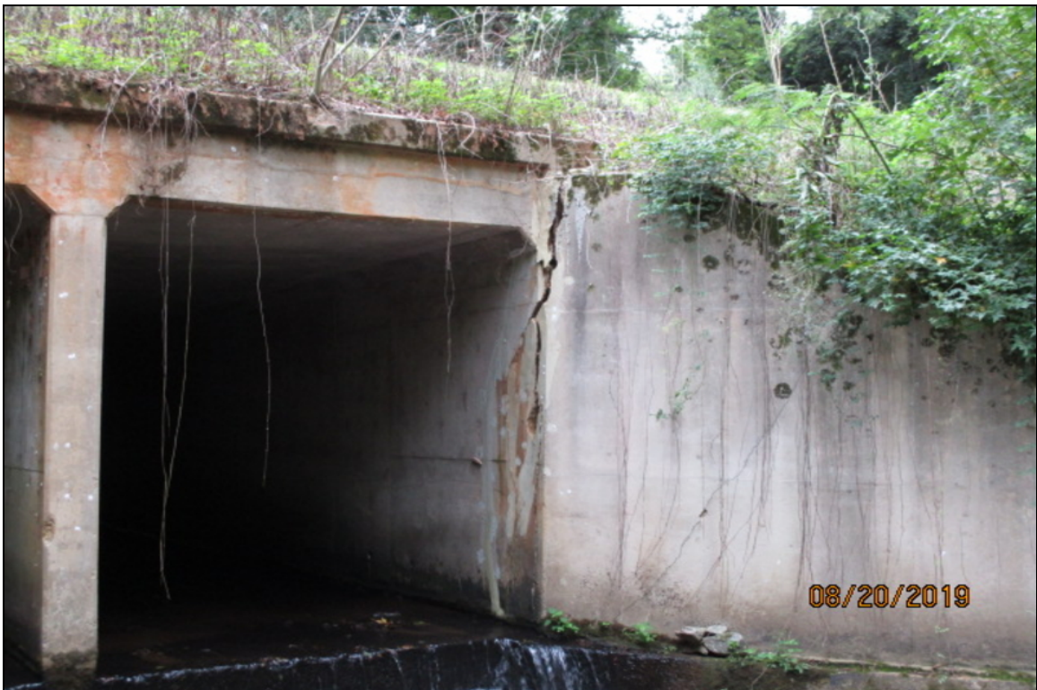
Crack in rear outlet wing
