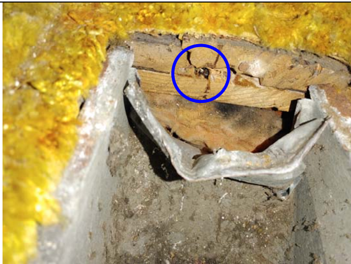
Photo 11 – Felt paper under wooden floor throughout
