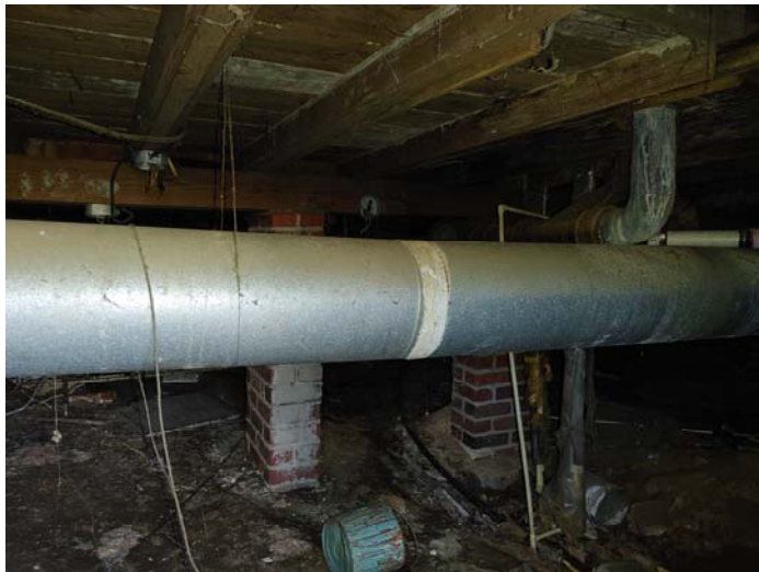
Photo 7 – HVAC A-Tape in the crawlspace
