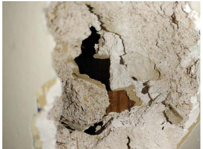
Photo 10 – Unfinished drywall scattered throughout beneath the plaster walls
