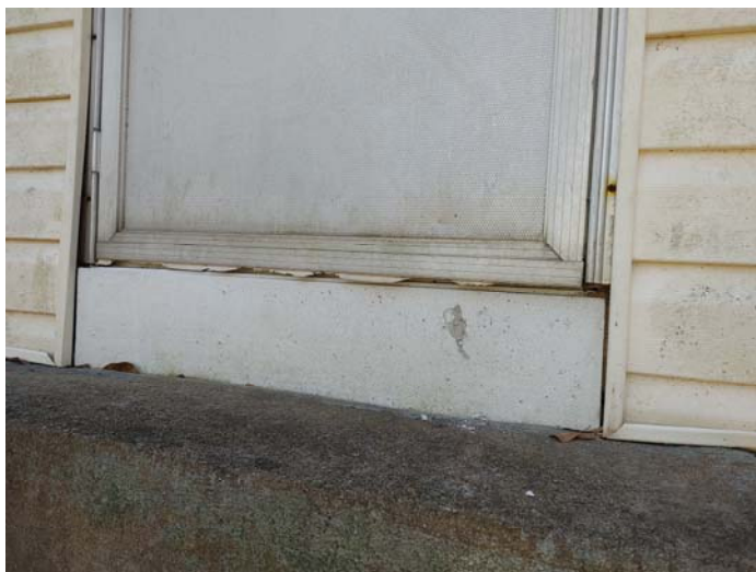
Photo 17 – Transite under back door
