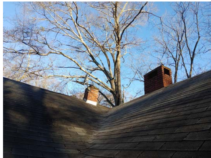
Photo 3 – View of 2 chimney's with tar – assumed positive
