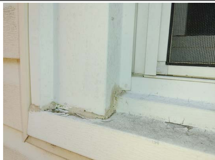
Photo 5 – Caulk on metal wrapping over window casings/frames
