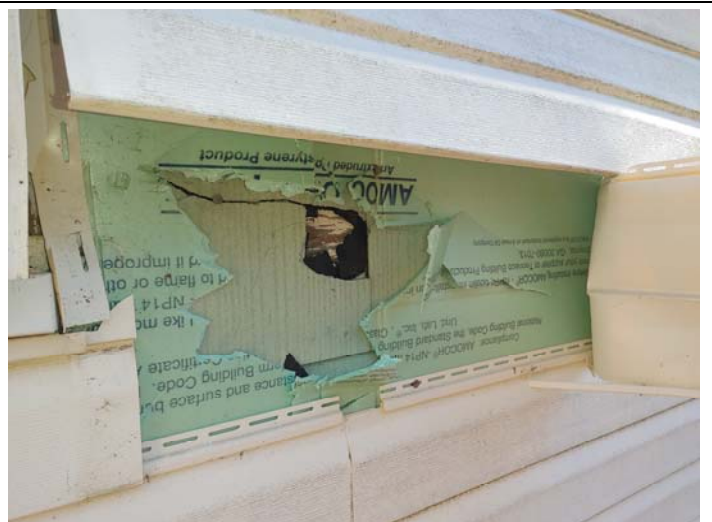
Photo 6 – Transite with felt below the vinyl siding
