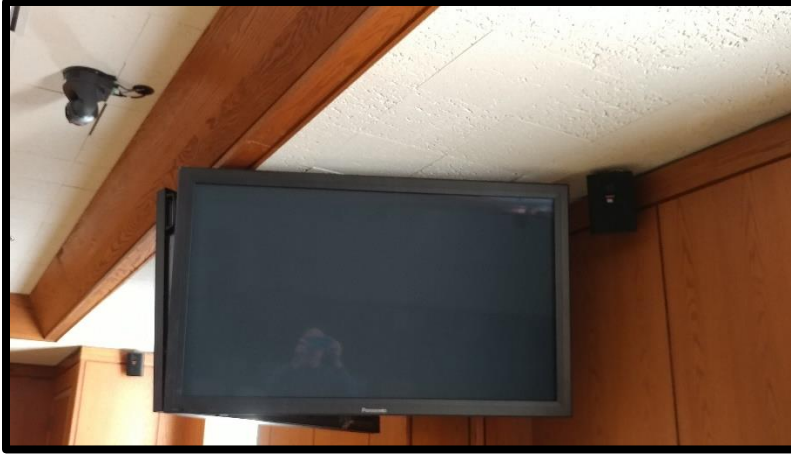
(2) ceiling-mounted video displays
