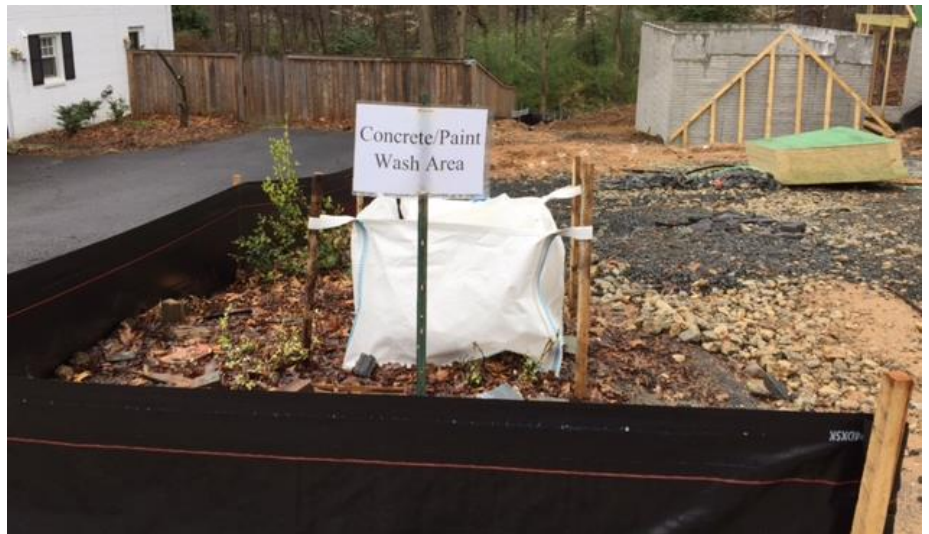
Example small-scale concrete and paint washout area.
