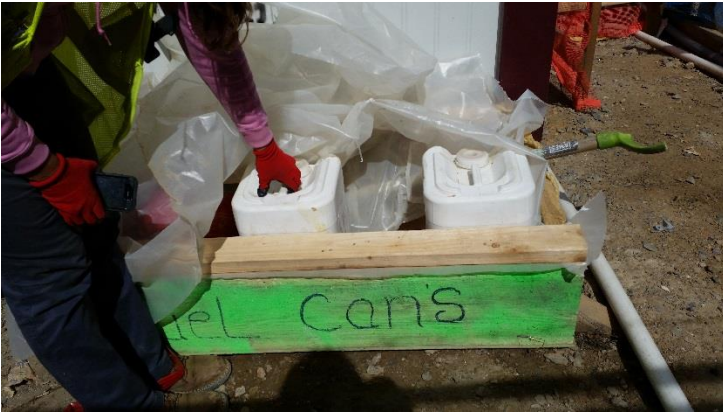
Fuel storage example. Cans are closed and located inside of a lined, secondary containment. The cans are also covered by a plastic liner to protect them from the elements.
