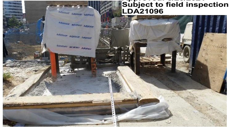
Chemical storage example. Containers are closed, covered by a tarp, and off of the ground.
