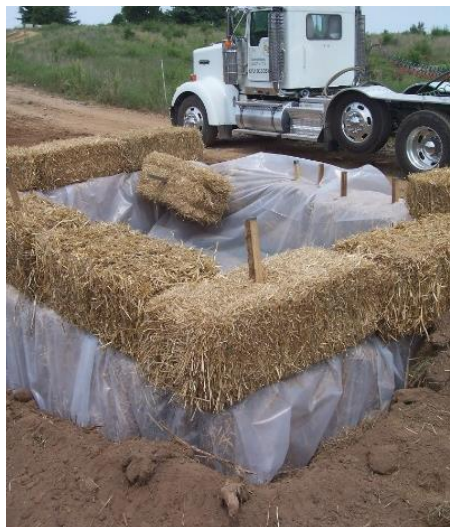
Example washout structures. Note that each example is fully lined and the washout is contained.
