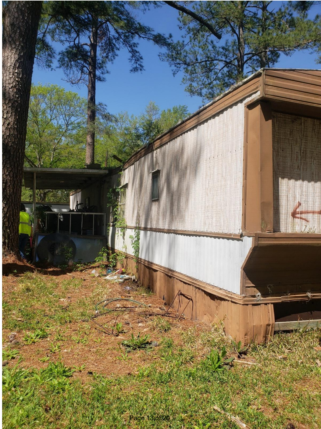
140 Claussen Street, Summerville, SC – Roof caving in and full of storage
