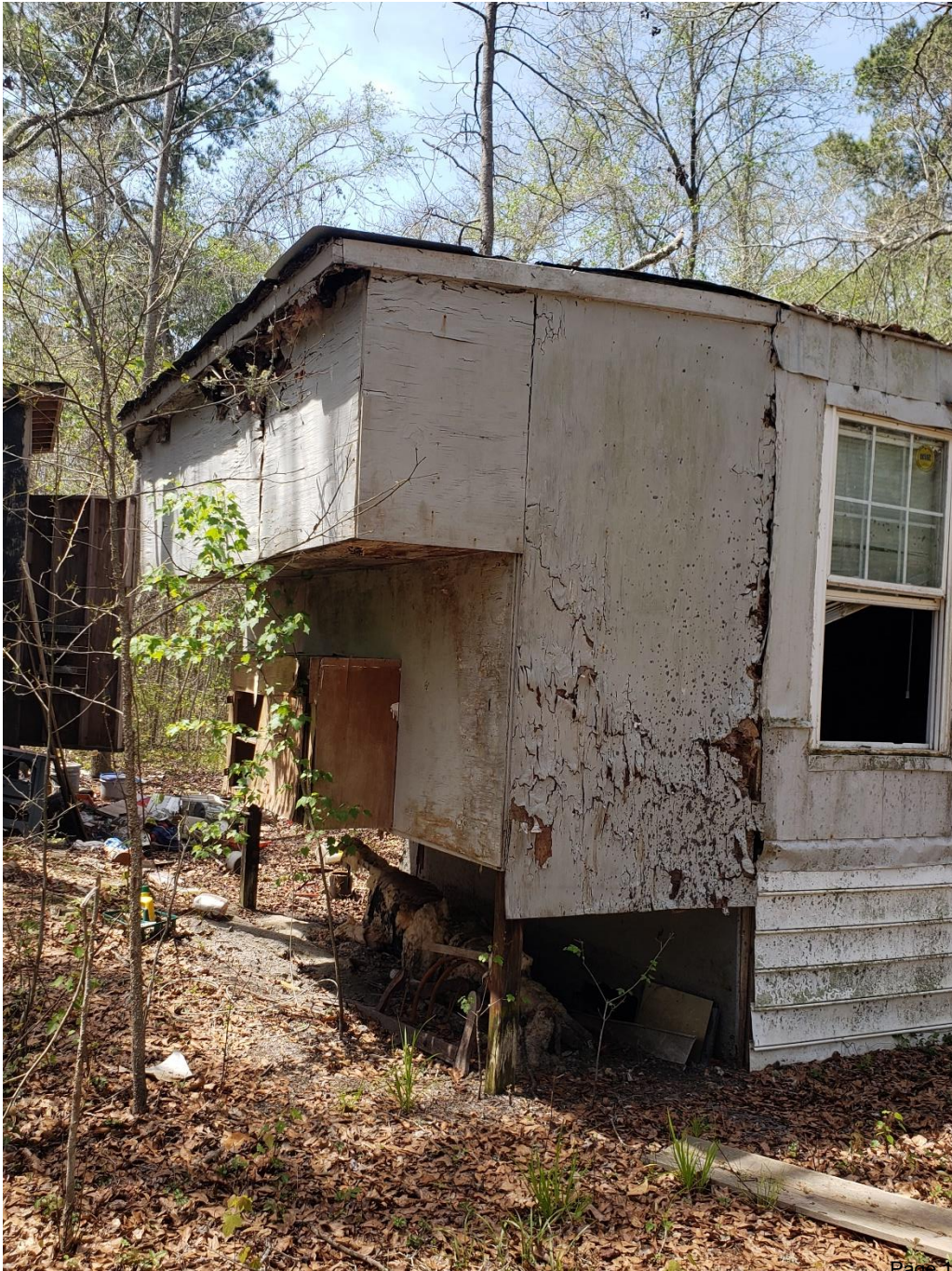
3318 Highway 17A South, Ridgeville, SC – Poor condition, open to elements, caution when crossing “bridge” on driveway
