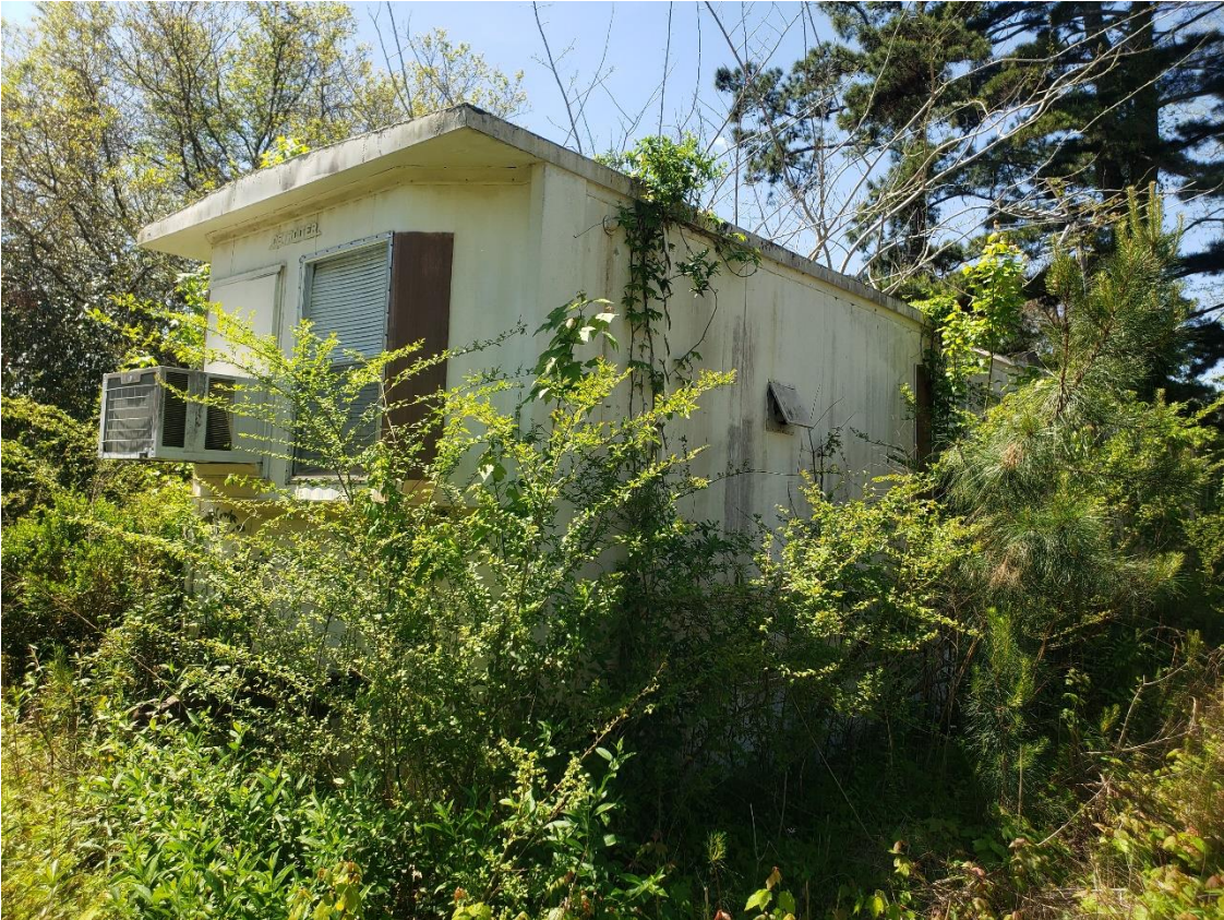
480 Embassy Drive, Summerville, SC – Roof caving in and open to elements
