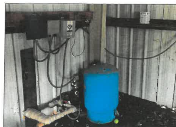
4 EXISTING WELL PUMP SYSTEM E1.1
