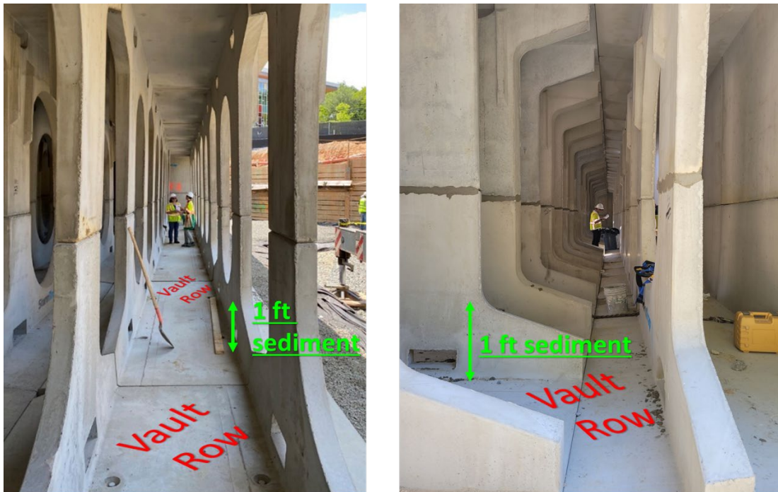
Figure 6. The vault rows and time trigger for maintenance (1 foot of sediment captured in the vault row).
