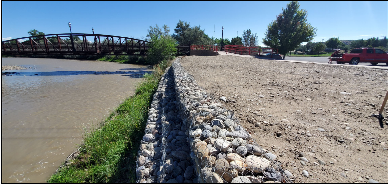
Existing Gabion Wall along Animas River near Boring B-5 View Towards the East
