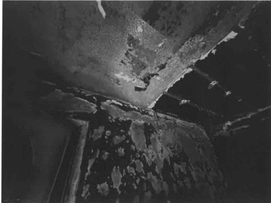
Inside of structure showing structural damage
