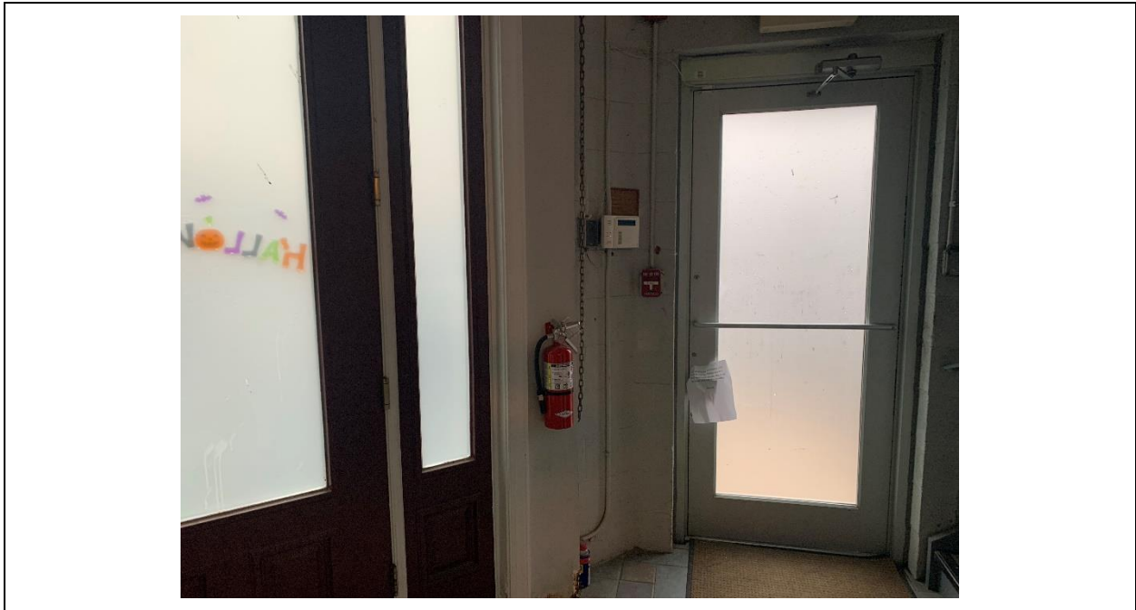
Typical Fire Extinguisher and Fire Alarm Pull-Down Station at the Subject Property
