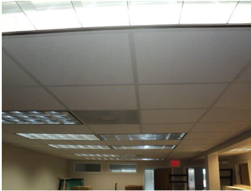
Homogeneous Material No. 21 – Non-ACM 2' X 2' White textured pinhole Lay-in Ceiling Tile located in Portion of the 2 nd Floor Mezzanine Area in the Back
