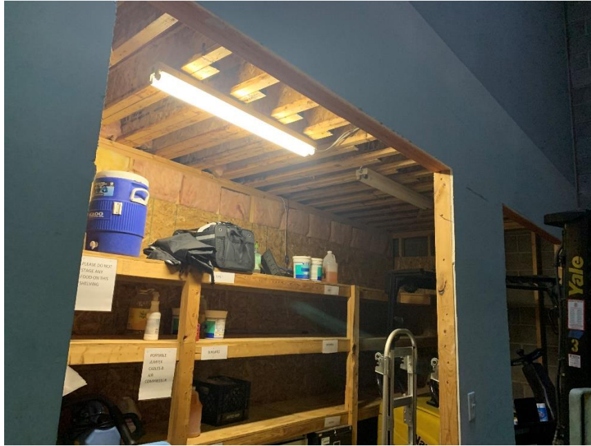
Typical Fluorescent Lighting in the Storage Area of the Arlington Food Assistance Center at the Subject Property
