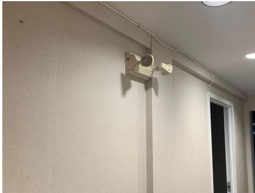
Different Type of Emergency Lighting at the Subject Property
