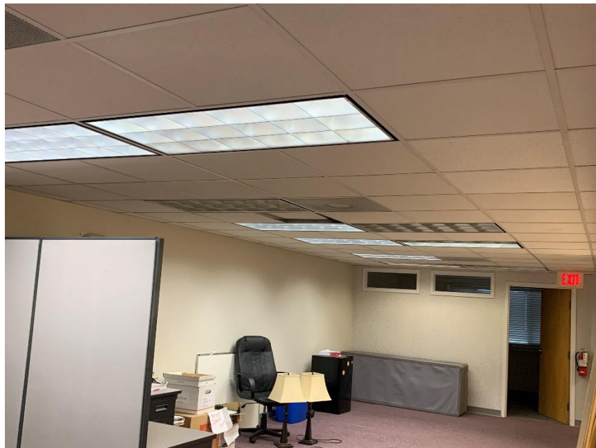
Recessed Fluorescent Lighting in the office Space of the 2 nd Floor Front Mezzanine Area of the Subject Property
