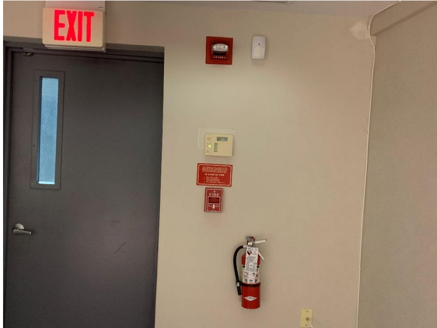
Fire Extinguisher, Pull-Down Station, Fire Strobe, Alarm System Control Panel and Motion Detector at the Subject Property
