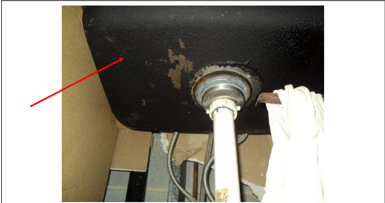
Homogeneous Material No. 11 – ACM Black Sink Bowl Mastic Coating located in Kitchen of the Inner Ear Studio
