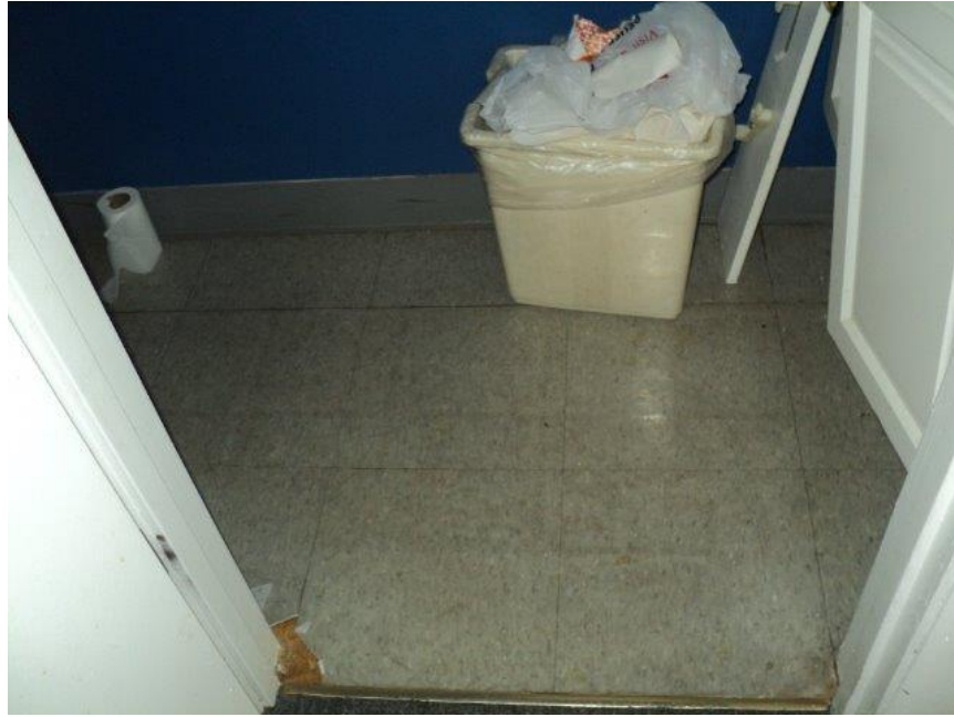
Homogeneous Material No. 5 – Non-ACM Grey 12" X 12" Vinyl Floor Tile with Light Yellow Mastic located throughout 1 st Floor and Restrooms in 2 nd floor front Mezzanine Area
