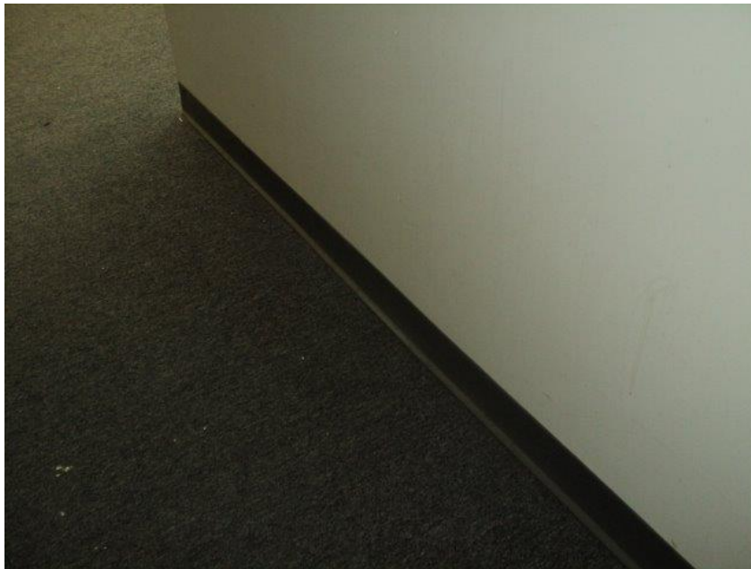
Homogeneous Material No. 4 – Non-ACM Grey 4” Vinyl Cove Base with Cream and Yellow Mastic located throughout 1 st Floor and 2 nd floor front Mezzanine Area
