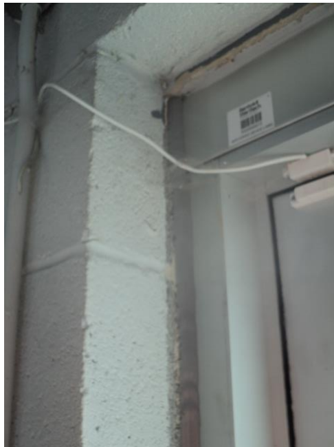
Homogeneous Material No. 2 – Non-ACM Grey Caulk located at the Interior Door in the 2 nd Floor Front Mezzanine Area
