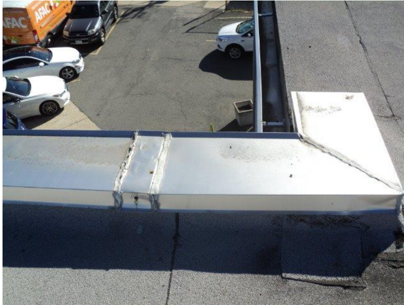
Homogeneous Material No. 20 – Non-ACM Grey Mastic – Grey HVAC Duct Mastic located on the Lower Roof of the Building
