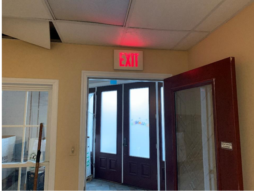
Lighted Exit Sign near the Front Entrance of the Arlington Count Food Assistance Center
