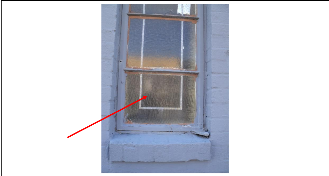
Homogeneous Material No. 15 – ACM White/Off-White exterior Window glazing compound located in the Exterior Metal Window of Inner Ear Studio
