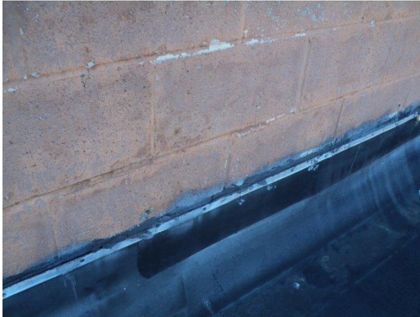
Homogeneous Material No. 17 – Non-ACM Black flashing caulk located on the Lower Roof of the Building
