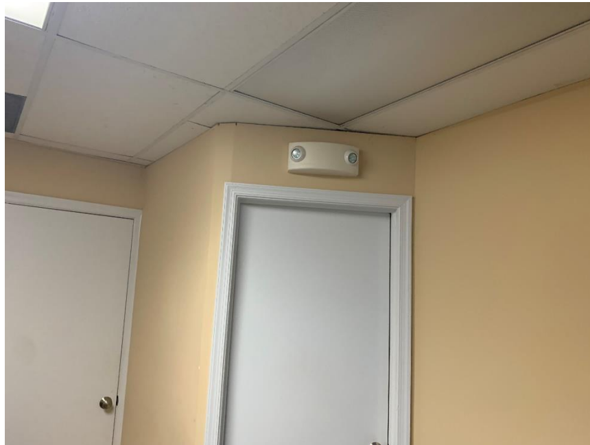
Typical Emergency Lighting at the Arlington Count Food Assistance Center
