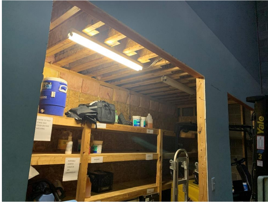
Typical Fluorescent Lighting in the Storage Area of the Arlington Food Assistance Center at the Subject Property
