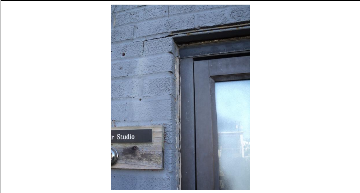
Homogeneous Material No. 13 – Non-ACM Grey Exterior Door caulk located outside the Inner Ear Studio
