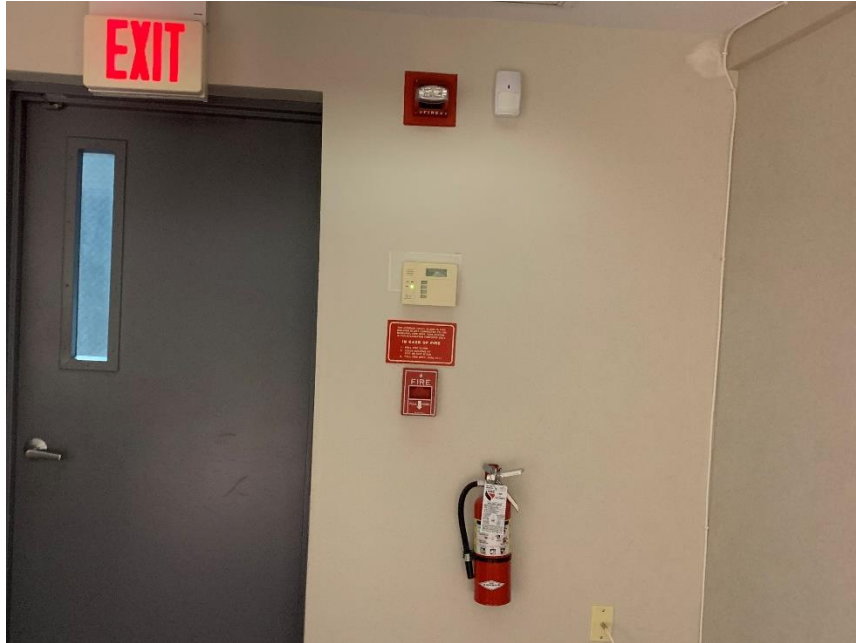
Fire Extinguisher, Pull-Down Station, Fire Strobe, Alarm System Control Panel and Motion Detector at the Subject Property
