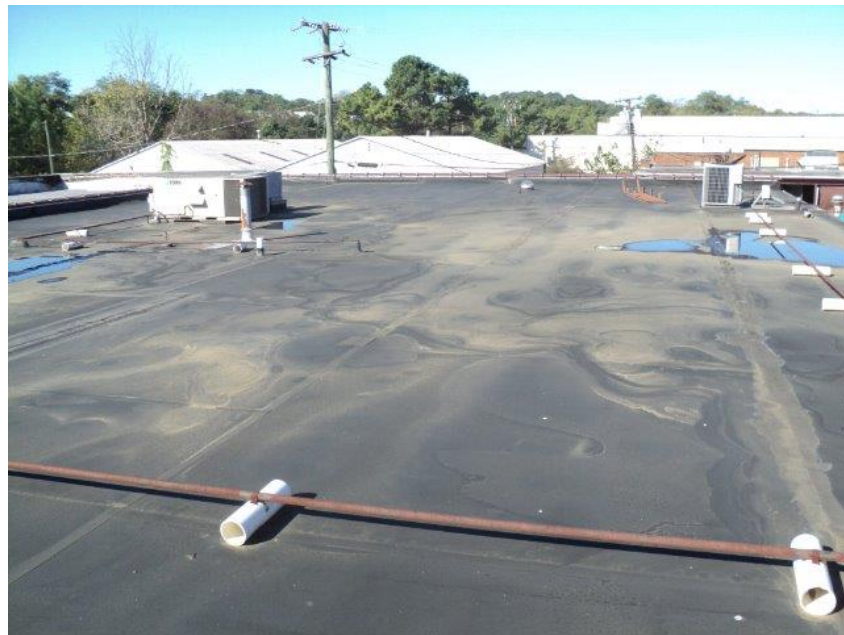
Homogeneous Material No. 18 – Non-ACM Black asphalt Sheet Roofing located on the upper Roof of the Building
