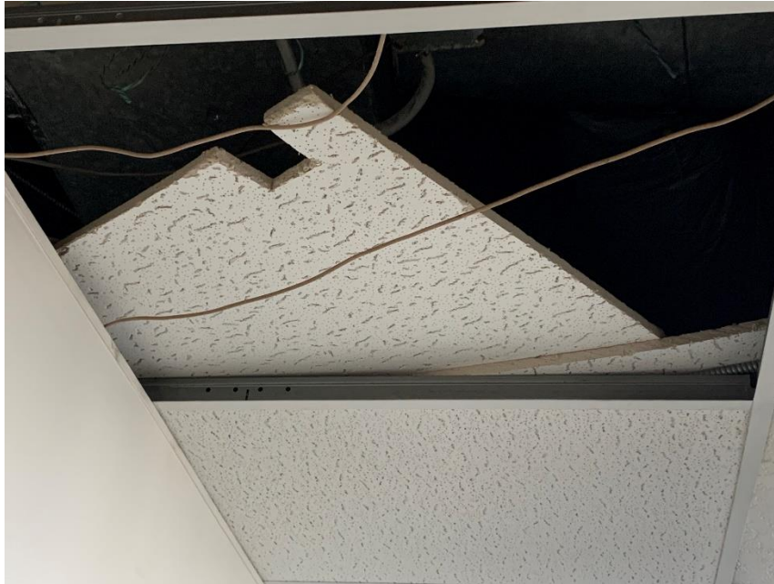
Homogeneous Material No. 3 – Non-ACM 2’X4’ White Textured Lay-in Ceiling Tile (dots with dashes design), located in all of 1 st floor and 2 nd floor front Mezzanine Plus part of back Mezzanine Area
