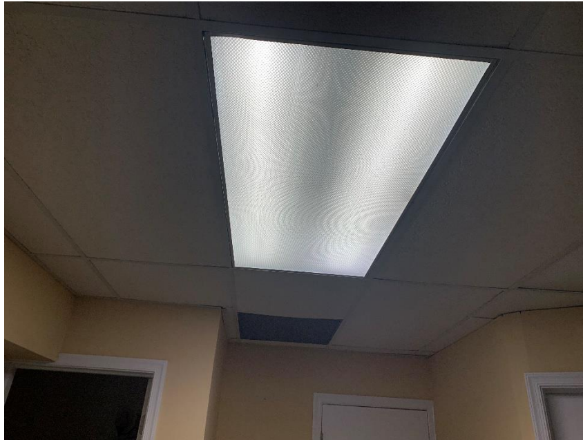
Typical fluorescent Lighting at the Subject Property
