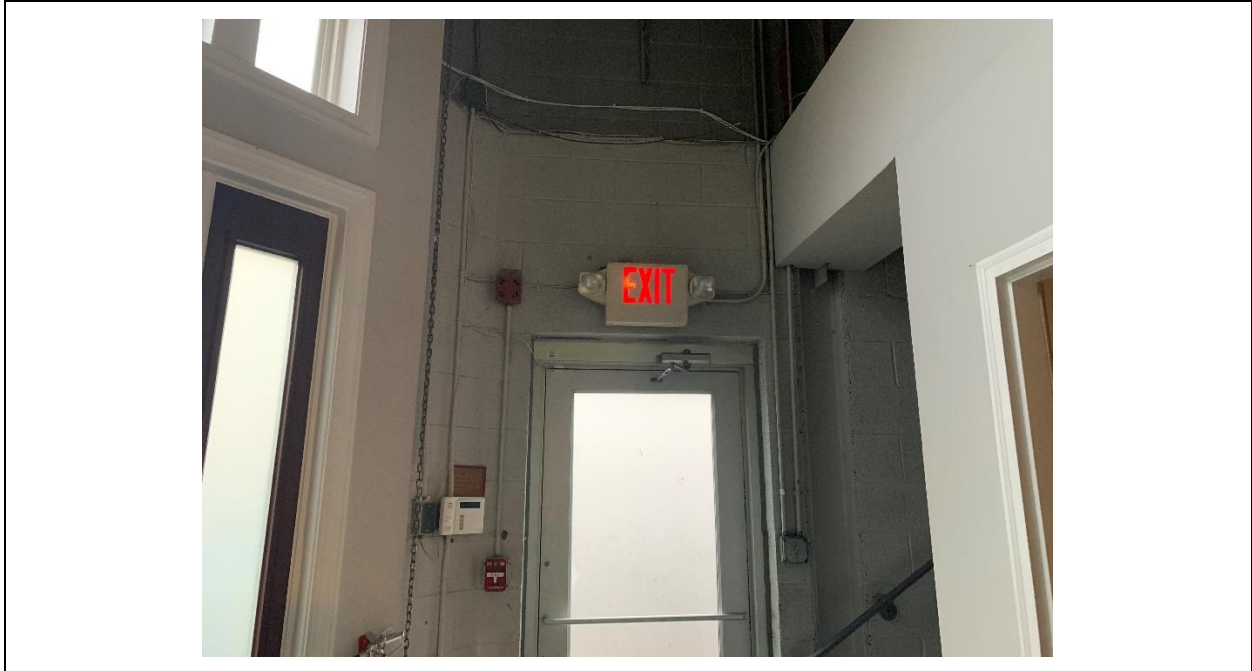
Typical Lighted Sign and Emergency Lighting Combination at the Subject Property
