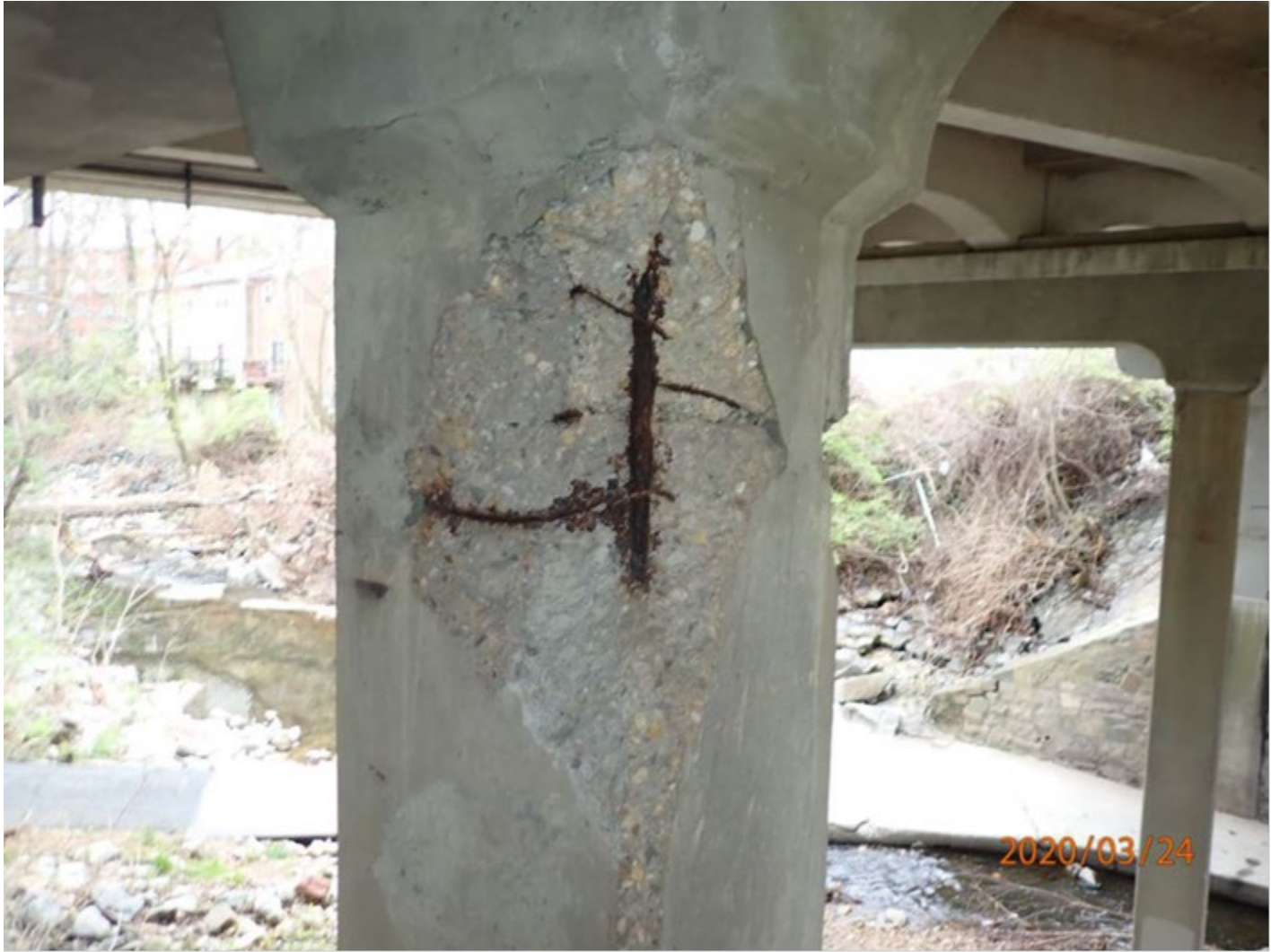
Picture 3 - Typical spall/delamination with exposed rebar on piers.
