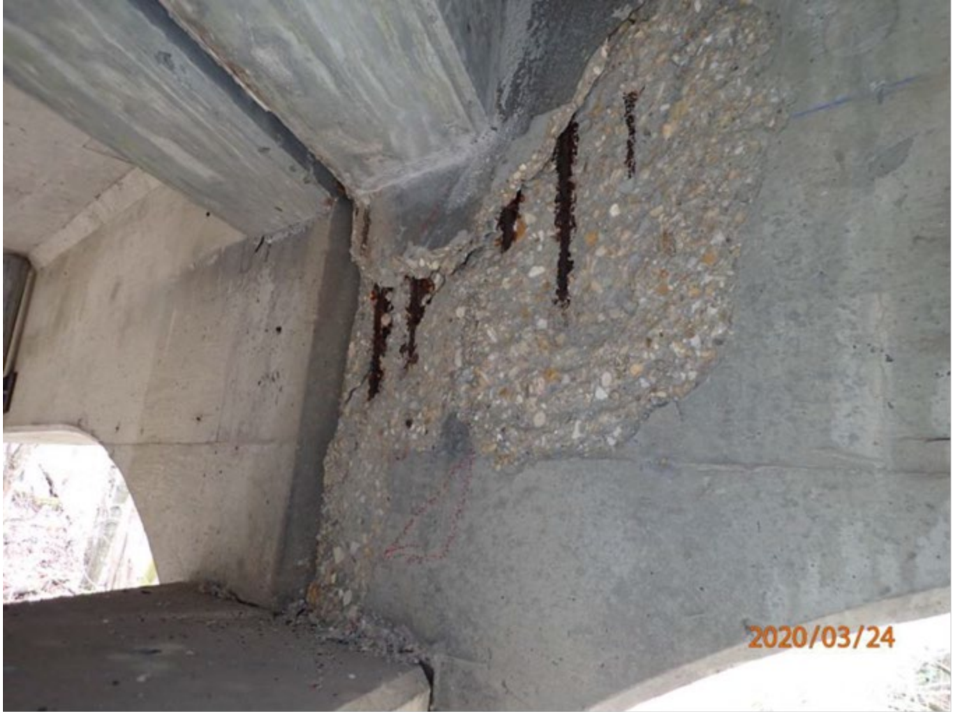
Picture 2 - Typical spalls /delamination with exposed stirrups beams end.
