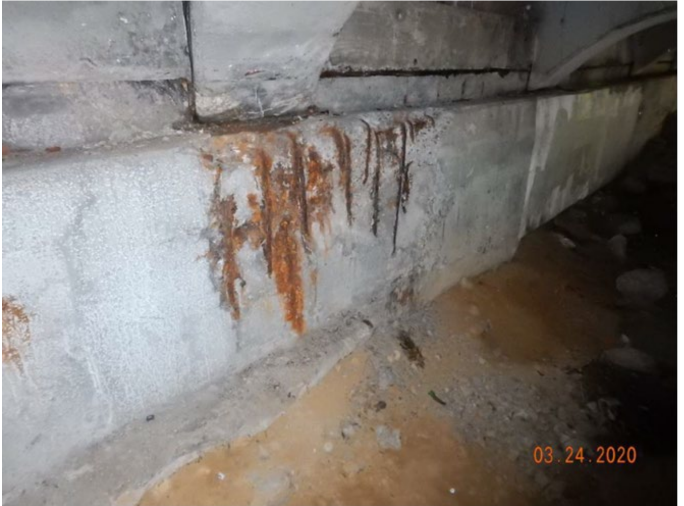
Picture 4 - Typical Spall/delamination on abutment A breast wall
