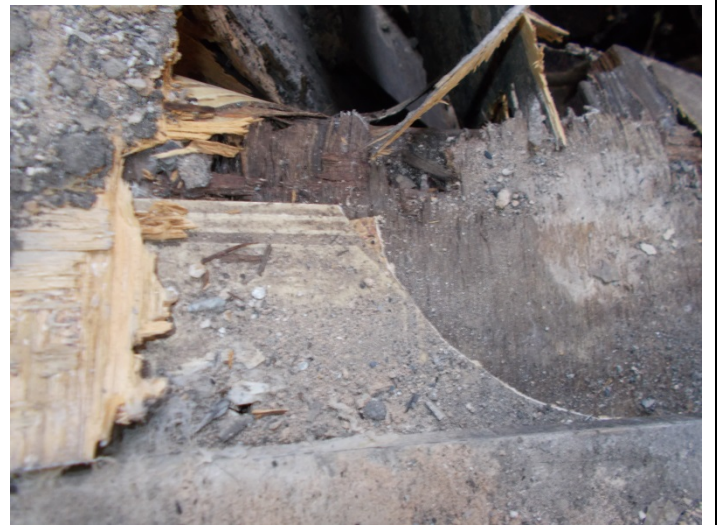
Photo 16 – 3 layers of vinyl flooring with & without mastics in the back damaged area.
