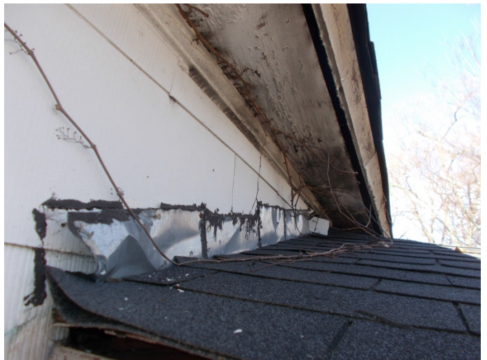
Photo 6 – Black mastic on roof flashing.
