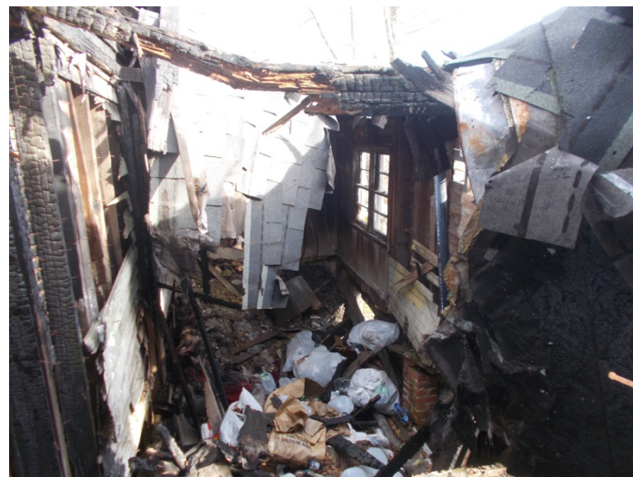
Photo 17 – Back damaged area.
