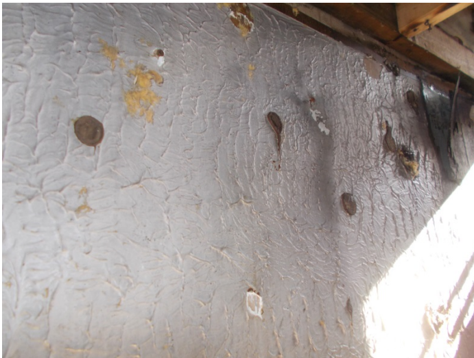
Photo 9 – Black mastic dots behind drywall walls.
