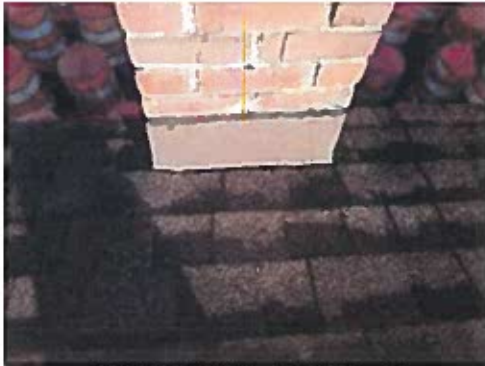
HOMOGENEOUS AREA 07 BRICK MASTIC (BLACK)
