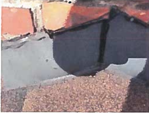
HOMOGENEOUS AREA 07 BRICK MASTIC (BLACK)
