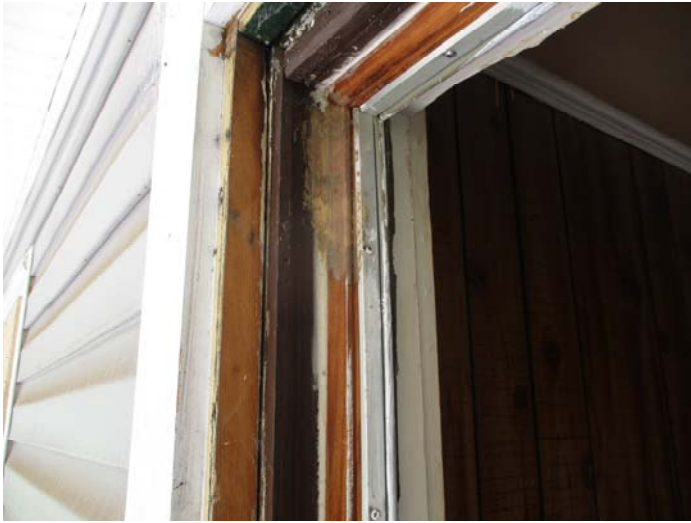
Photo 15 – Wooden door caulk
