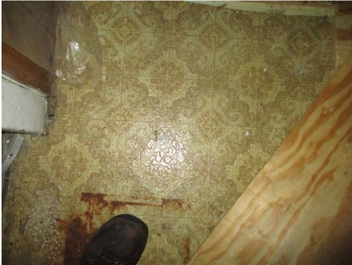
Photo 7 – Brown small square pattern roll vinyl floor & mastic in the back entry (2nd layer under wood)
