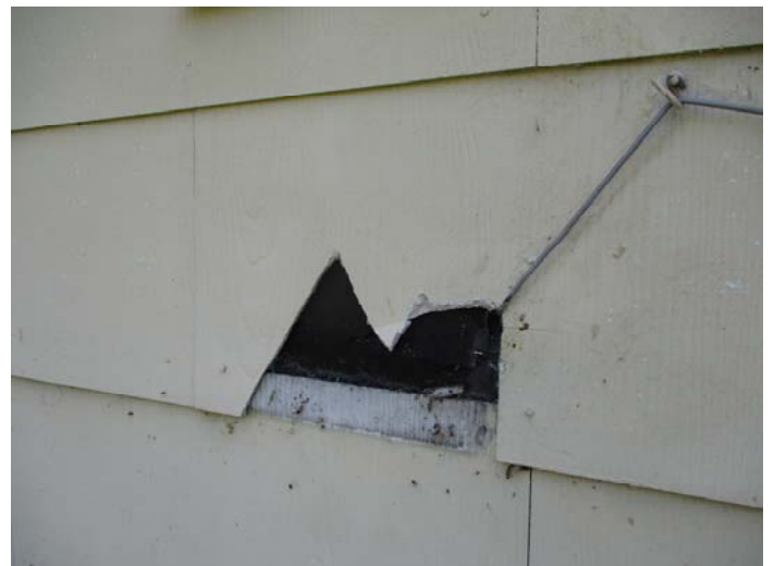
Photo 12 – Transite siding with felt paper beneath
