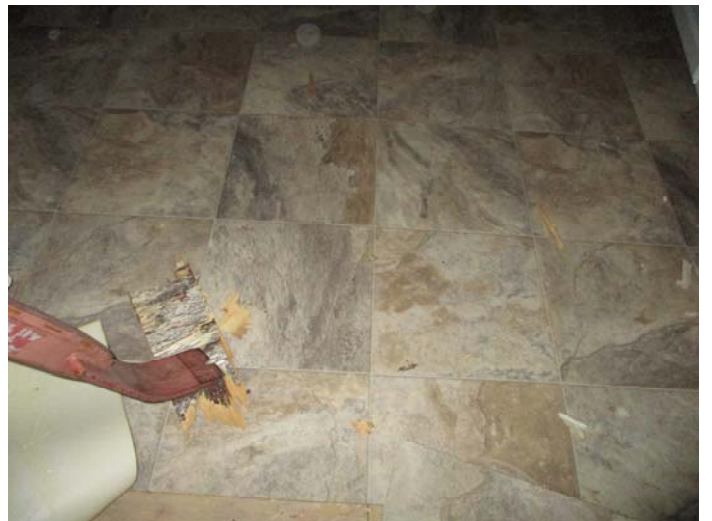
Photo 4 – 12" x 12" stone square pattern roll vinyl floor with no adhesive in the kitchen & back entry (top layer)
