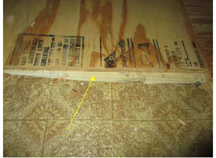
Photo 8 – Tan & gray flower pattern vinyl floor & adhesive patch in the back entry (under wood)
