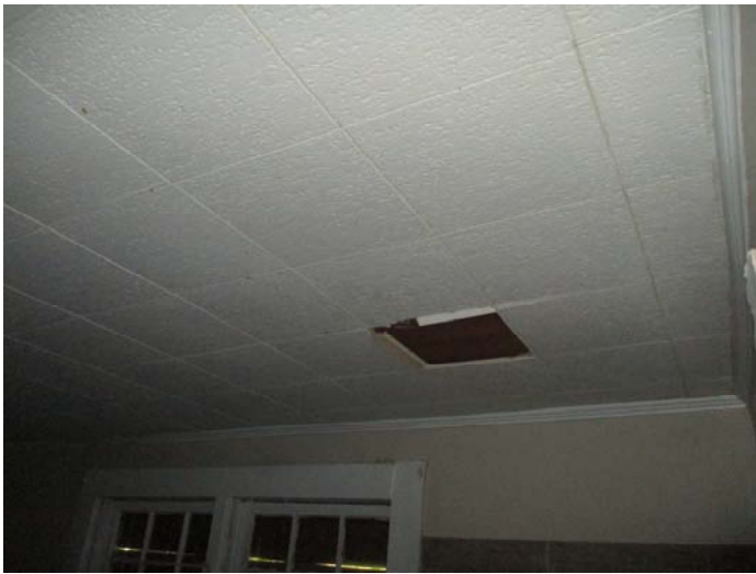
Photo 9 – 12" x 12" ceiling tiles with no mastic in the kitchen
