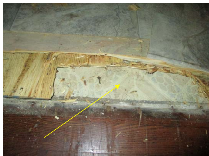
Photo 5 – Tan & gray flower pattern vinyl floor & adhesive in the kitchen (2 nd layer under wood)
