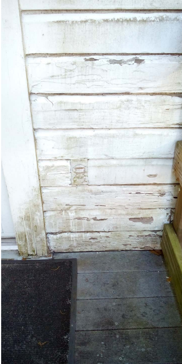
North Wall detail – showing example of wood that needs replacing.
