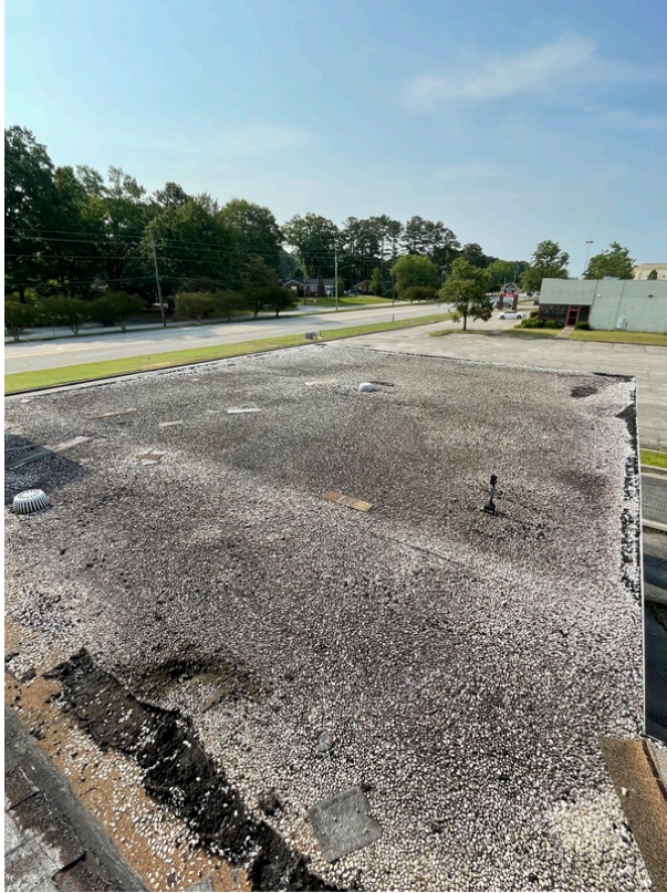
General view of the canopy roof on the Former Bank structure with asbestos-containing Brown Felt Paper beneath Gravel and Black Tar (HA 6)
