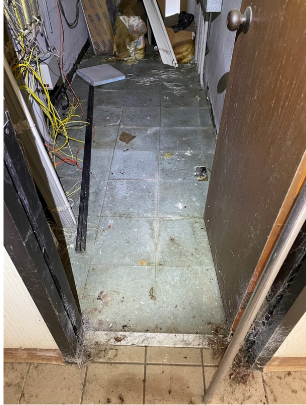
General view of asbestos-containing Tan/Black Mastic beneath 12" x 12" Green Floor Tile (HA 14)
