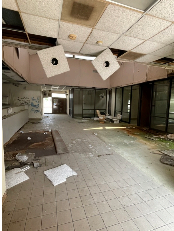
General view of the interior of the Former Bank structure on the Subject Property
