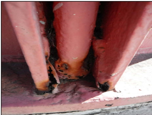
Riser Foundation Bolt
