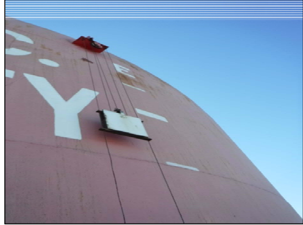
Broken Level Indicator
