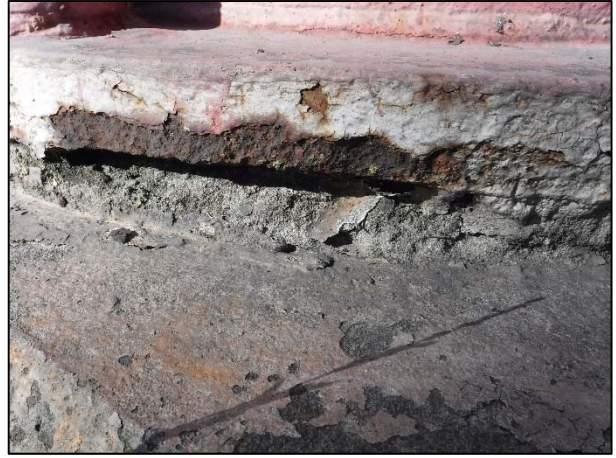
Erosion Under Column Base Plate
