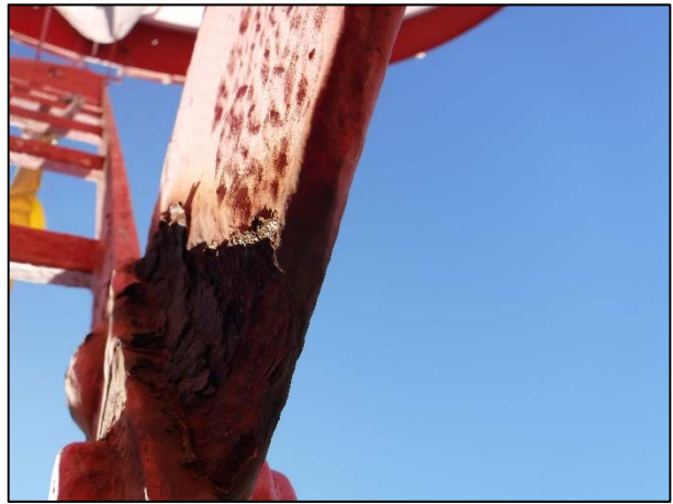
Corroded Ladder Standoff
