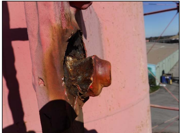
Severe Corrosion of Ladder Bolts
