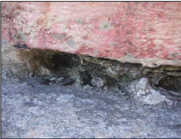
Erosion Under Column Base Plate
