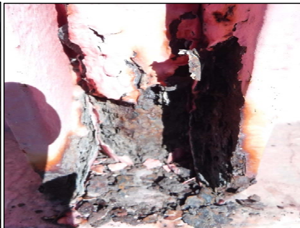
Riser Foundation Bolt
