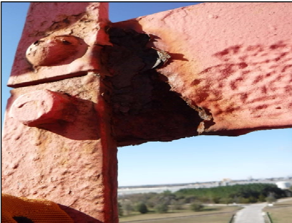
Corroded Ladder Standoff
