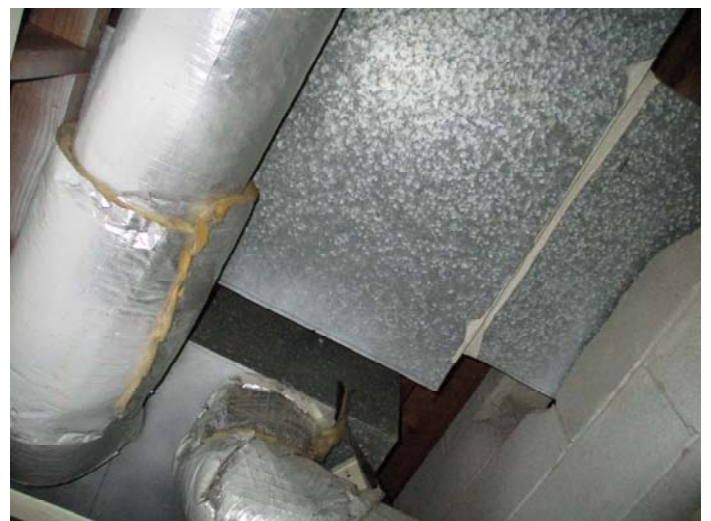
Photo 24 – A-Tape on HVAC
