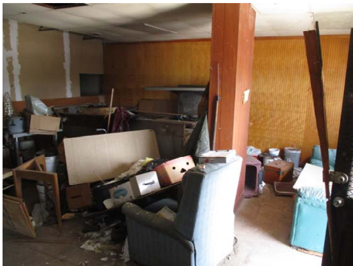
Photo 23 – Typical view of items and debris throughout the building
