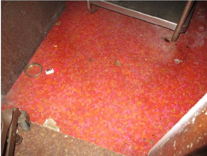
Photo 13 – Red pattern vinyl floor & adhesive in the left side 2nd bathroom on the right & right side 2nd room
