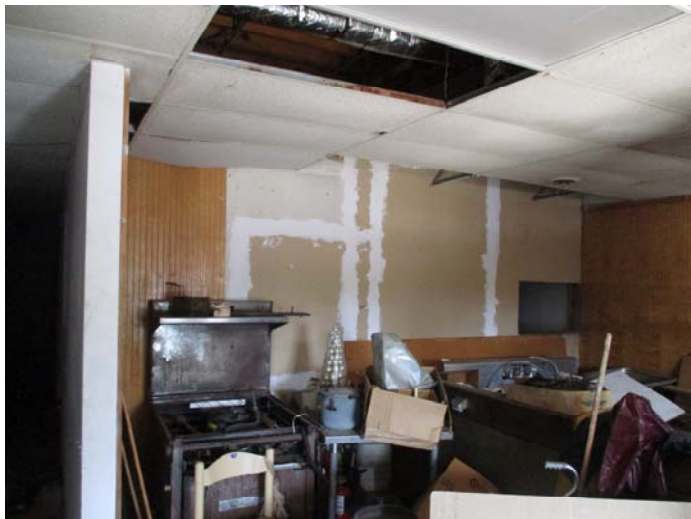
Photo 21 – Drywall with joint compound & tape in the left side walls & bathrooms & throughout the right side except in the back room
