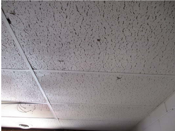
Photo 18 – 2' x 4' fissure ceiling tiles in the right side
