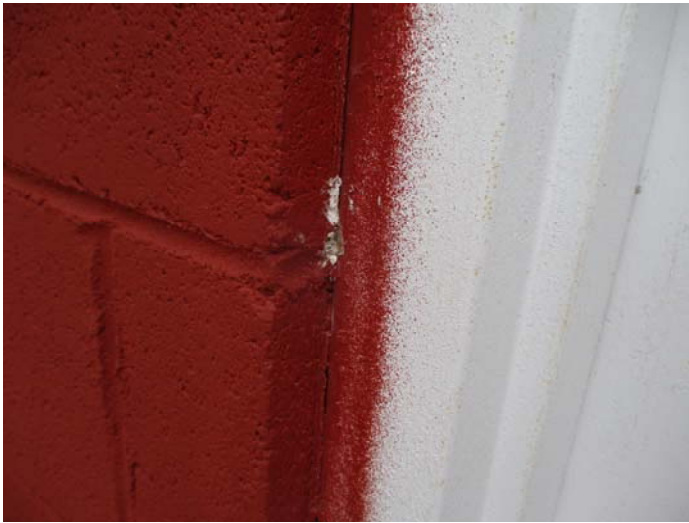
Photo 7 – Red metal door caulk
