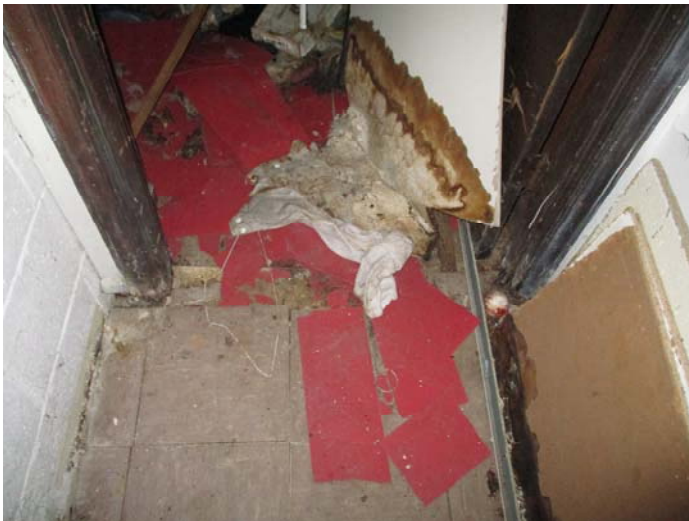
Photo 17 – 12" x 12" red floor tile with no mastic in the right side 4th room on the right
