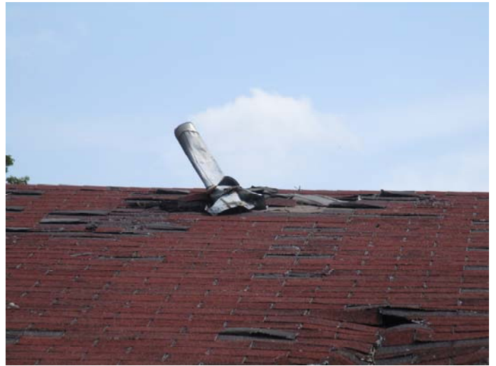
Photo 8 – Tar on 1 roof vent – assumed positive
