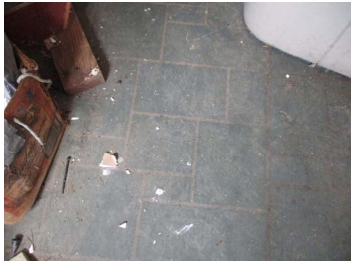
Photo 10 – Green square & rectangle pattern vinyl floor & adhesive in the left side front area
