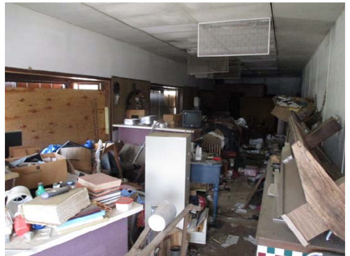
Photo 22 – Typical view of items and debris throughout the building
