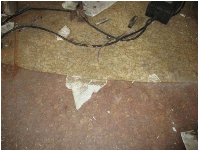
Photo 9 – Typical view of the tan & brown vinyl floor & adhesive. Exists as single layers & 2 nd layers
