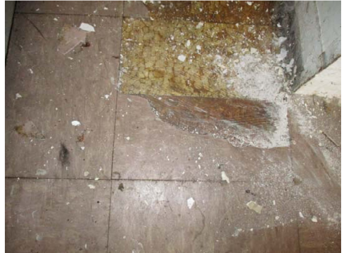
Photo 14 – Top layer of 12" x 12" tan/gray peacock floor tile & brown adhesive in the right side front room, hallway & right side 1st room
