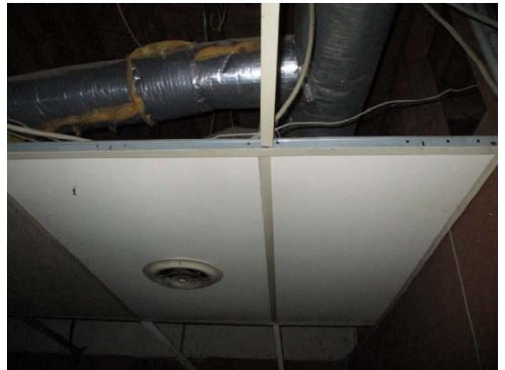
Photo 18 – 2' x 4' smooth ceiling tiles in the right side 4th room on the right & both bathrooms
