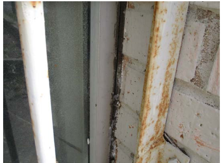
Photo 10 – Black caulk over tan caulk on metal windows
