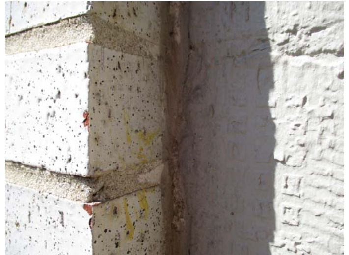
Photo 4 – Gray caulk on exterior siding & stucco
