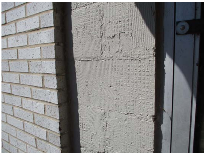
Photo 5 – Gray caulk on exterior siding & stucco
