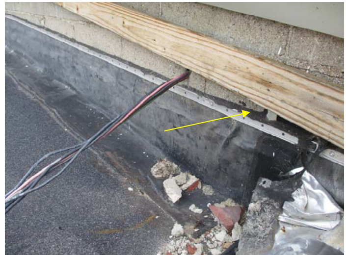
Photo 4 – Flashing caulk on the front roof
