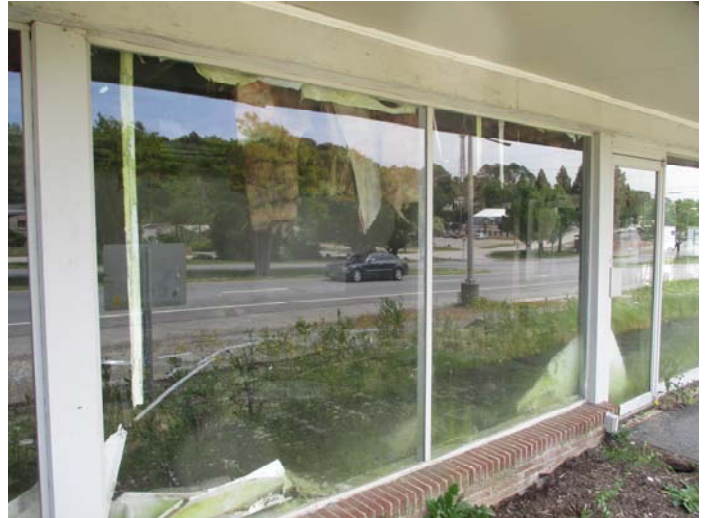
Photo 8 – Front metal windows with caulk over glazing
