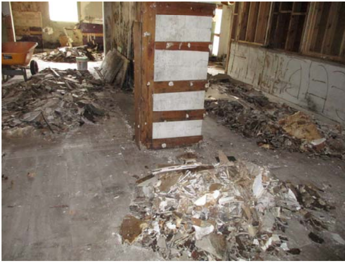
Photo 13 – Drywall with joint compound in debris piles
