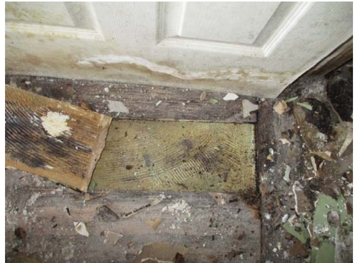
Photo 20 – Adhesive under wooden floors in the front area - left side
