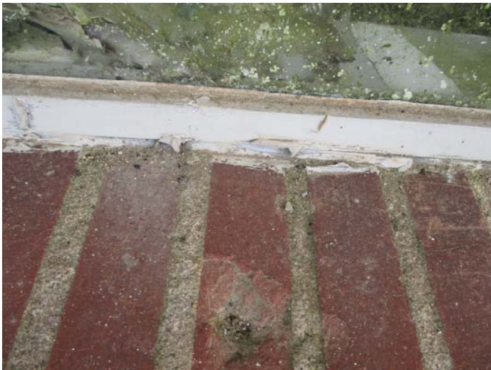
Photo 9 – Front metal windows with caulk over glazing
