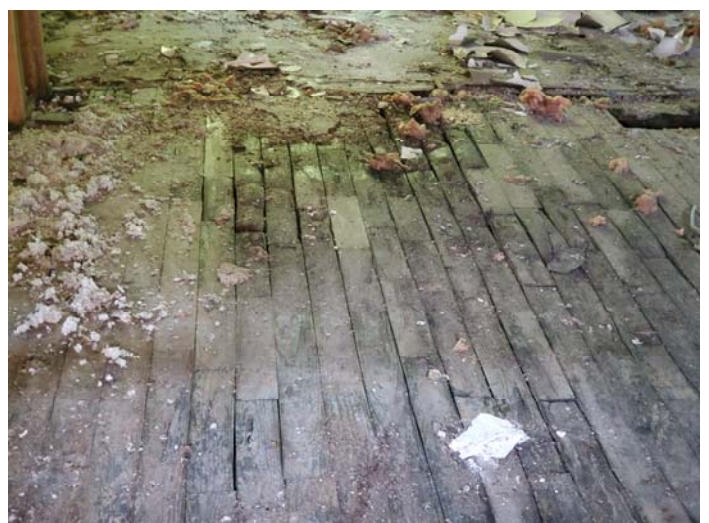
Photo 12 – Rotten wood on right side of duplex creates unstable floor
