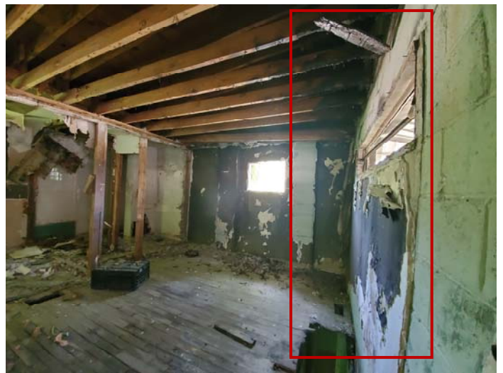
Photo 10 – Evidence of fire inside duplex
