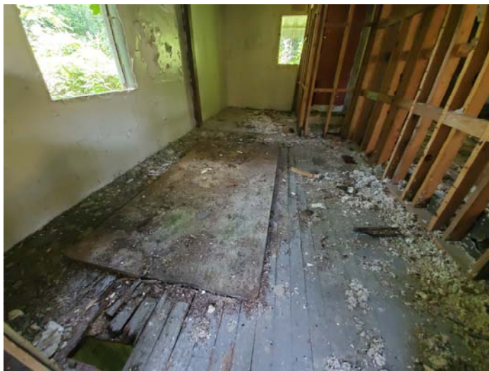
Photo 9 – Rotten wood on left side of duplex creates unstable floor
