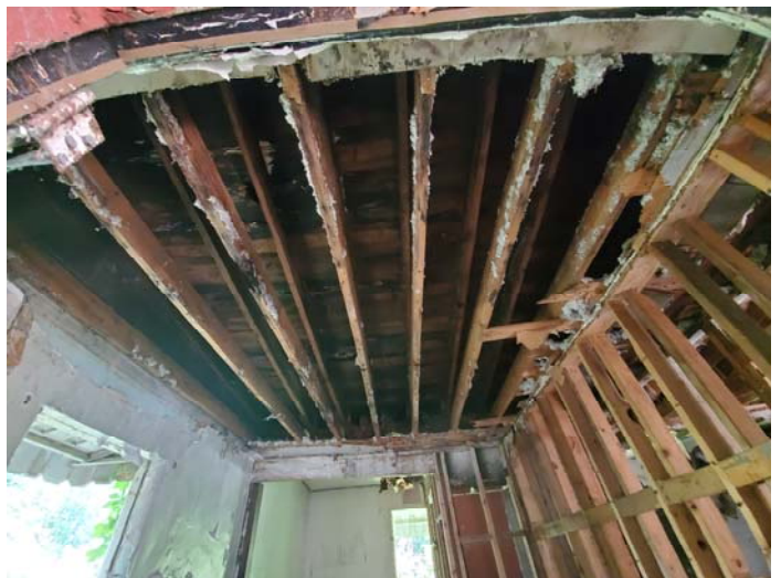
Photo 6 – Unfinished drywall sporadically located on upstairs ceiling and walls
