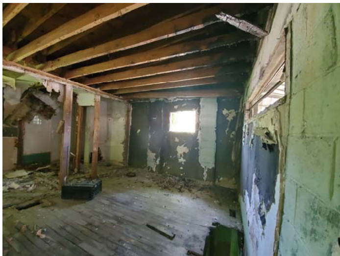
Photo 5 – Plaster with finish over unfinished drywall sporadically located on ceiling and walls
