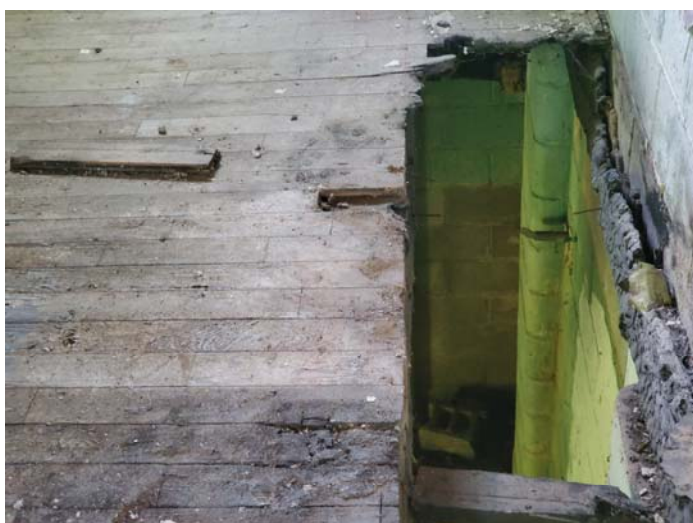
Photo 11 – Unstable floor resulting from previous fire
