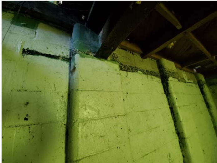
Photo 7 – Black mastic on downstairs walls
