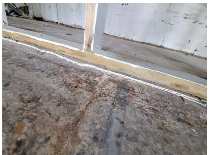
Photo 18 – Second layer of white floor tile under wood framing throughout located in section A/B
