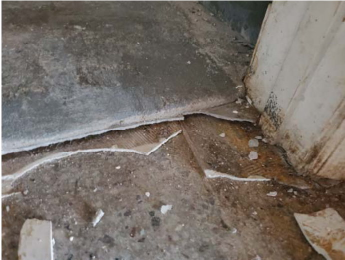
Photo 13 – Grey 12"x12" floor tile over 12"x12" tan floor tile with mastic under concrete in section A/B bathroom
