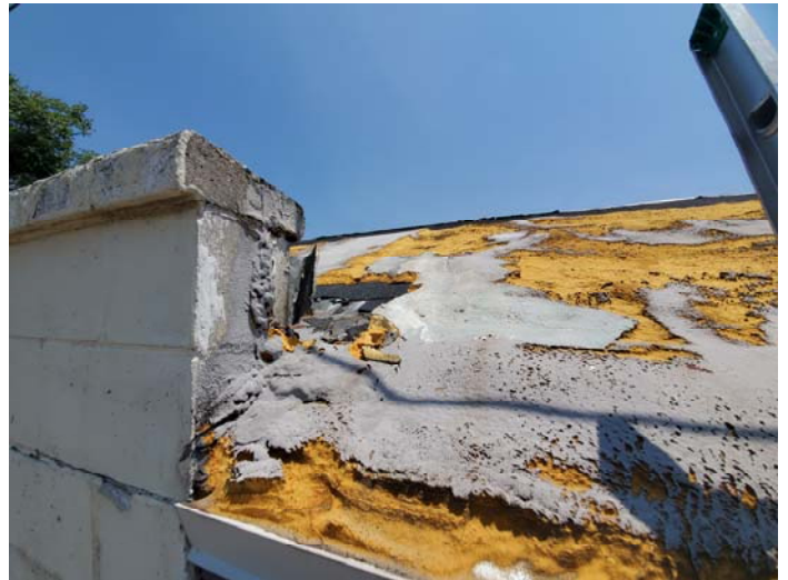
Photo 2 – Foam with grey sealant on top layer and mesh paper with tar on parapet wall.
