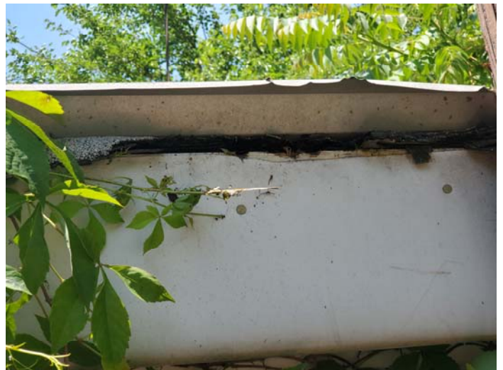
Photo 4 – Flat roof with five layers of shingles and one layer of felt paper located at back of building
