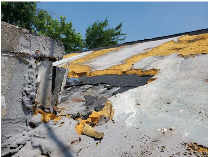
Photo 3 – Front roof has a metal roof with silver sealant and tar under two layers of shingles.
