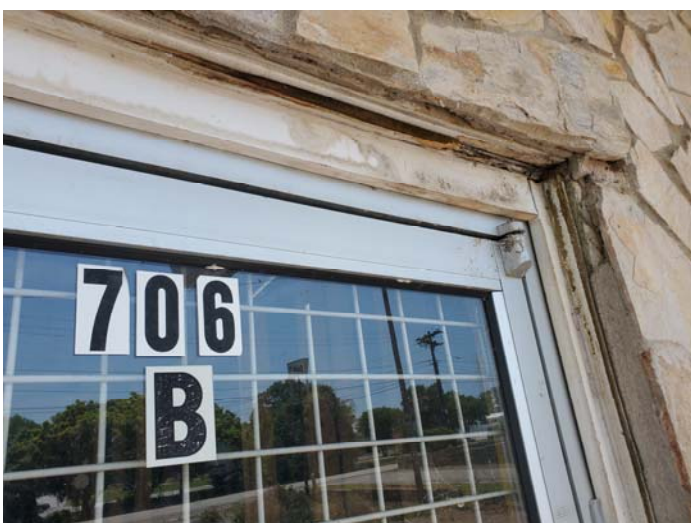
Photo 5 – 706B door frame with white caulk
