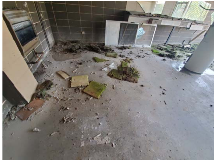
Photo 20 – 12"x12" ceiling tiles located on floor in section C
