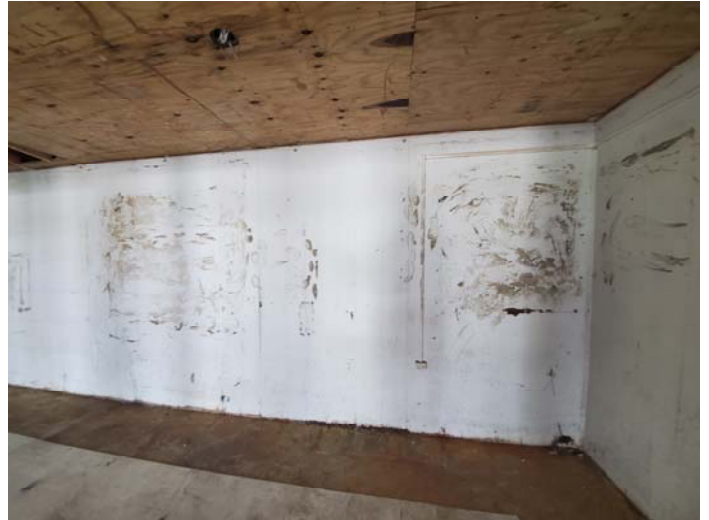
Photo 14 – Tan mastic over paneling on back wall in section A/B
