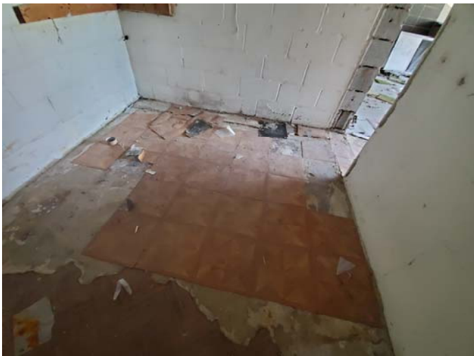
Photo 15 – 12"x12" wood pattern self-stick floor tile with adhesive in section C hallway
