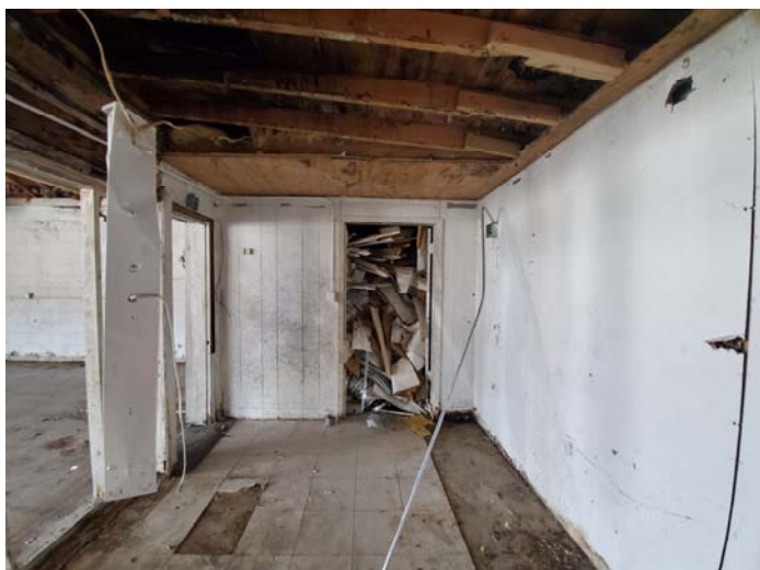
Photo 23 – Various types of building debris placed in section A/B closet.
