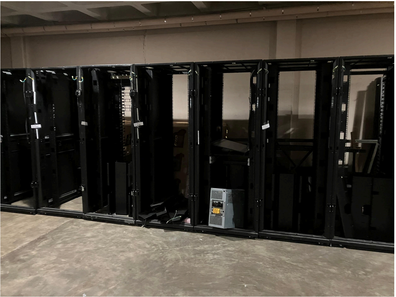
Below: Disassembled server rack system (current state)
