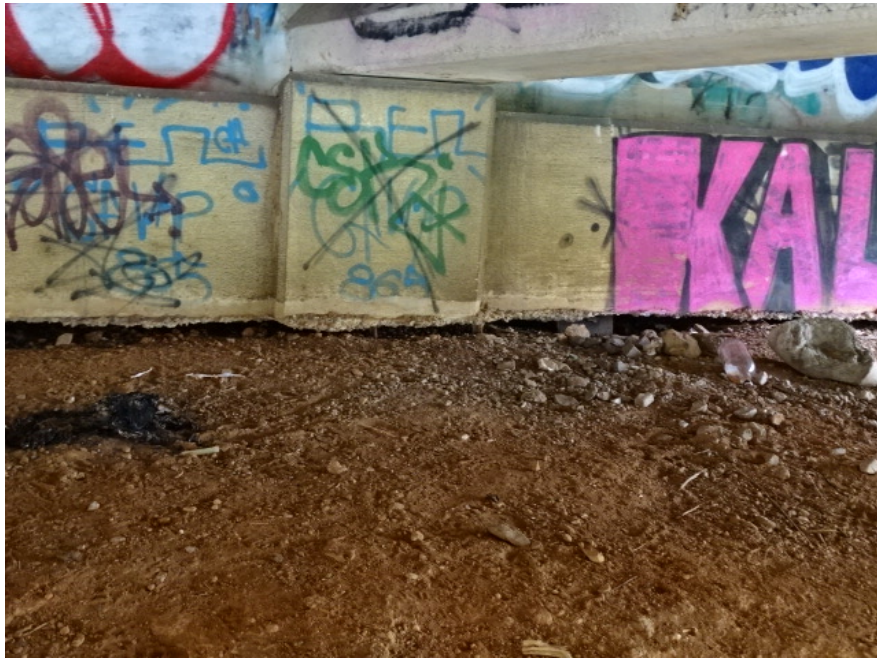
ERROSION WITH EXPOSED PILINGS - ABUTMENT 1
