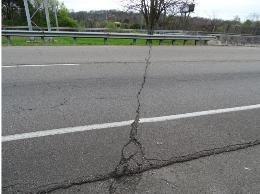
PAVEMENT RAVELING AT APPROACH 2
