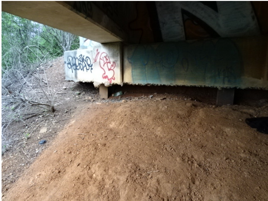
ERROSION WITH EXPOSED PILINGS - ABUTMENT 2
