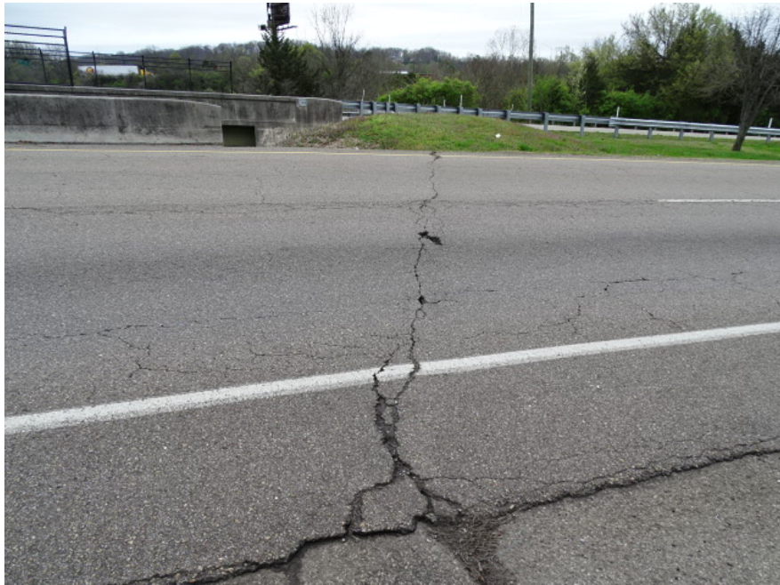
PAVEMENT RAVELING AT APPROACH 1
