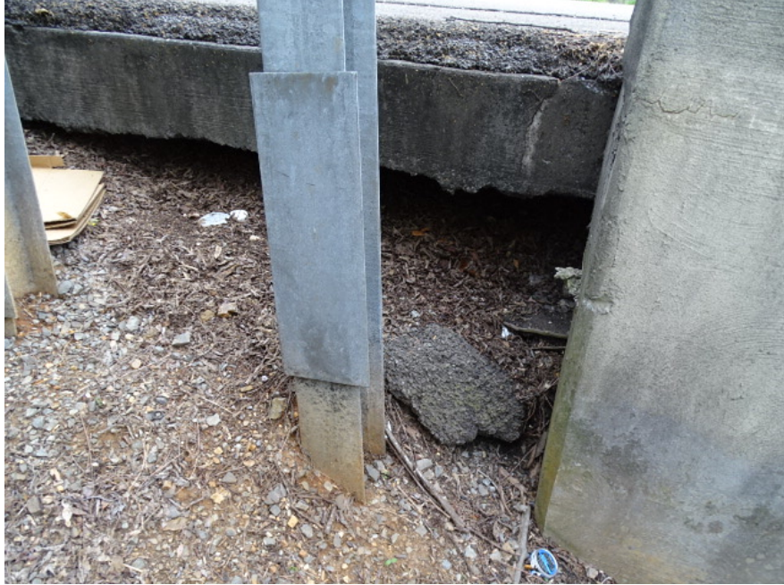
VOID UNDER APPROACH 2
