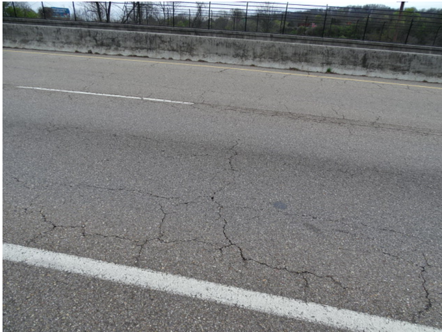
PAVEMENT RAVELING TOP DECK (TYP.)
