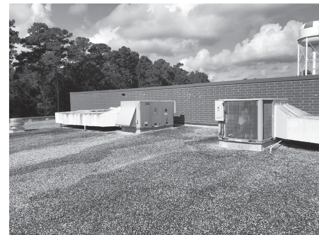
A ROOFTOP UNITS
