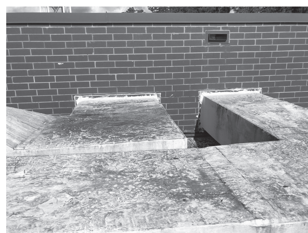
B SUPPLY AND RETURN DUCT
