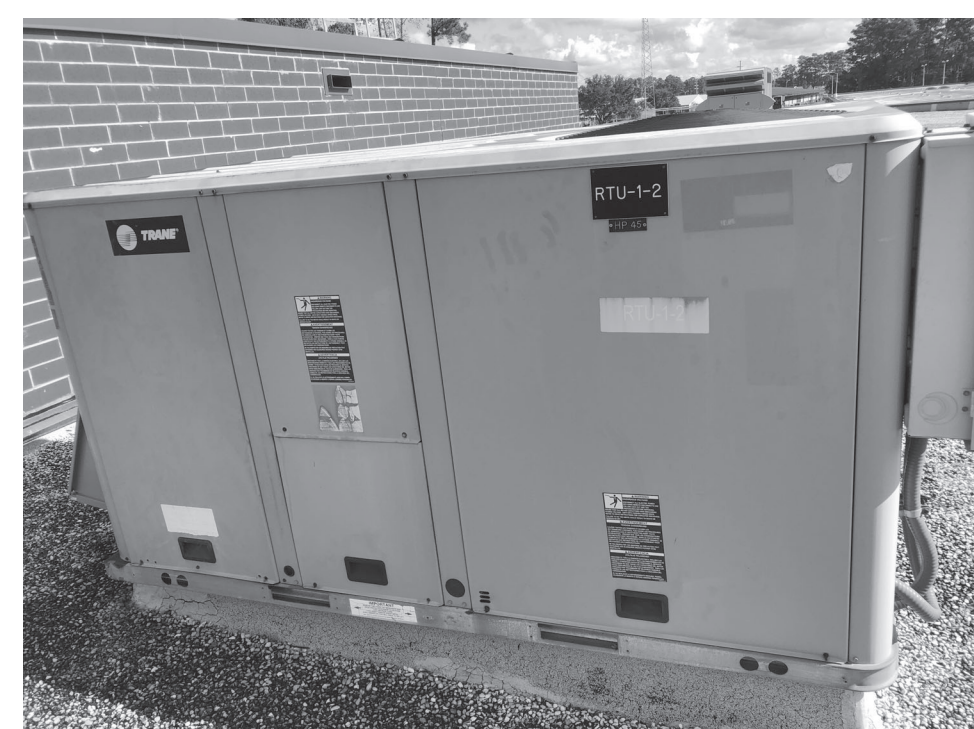
D ROOFTOP UNIT
