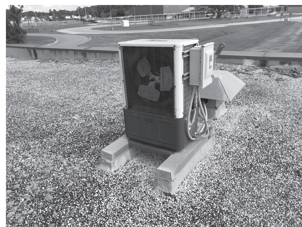
E DATA ROOM CONDENSER
