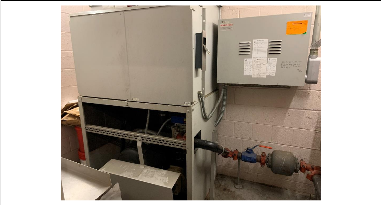
Control Box in the elevator room of the subject property building.
