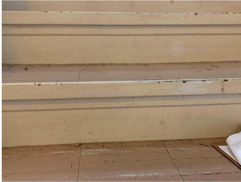
Lead-Containing Paint on the stairwell stair riser on the east side leading from the 1st floor to the 2nd floor.
