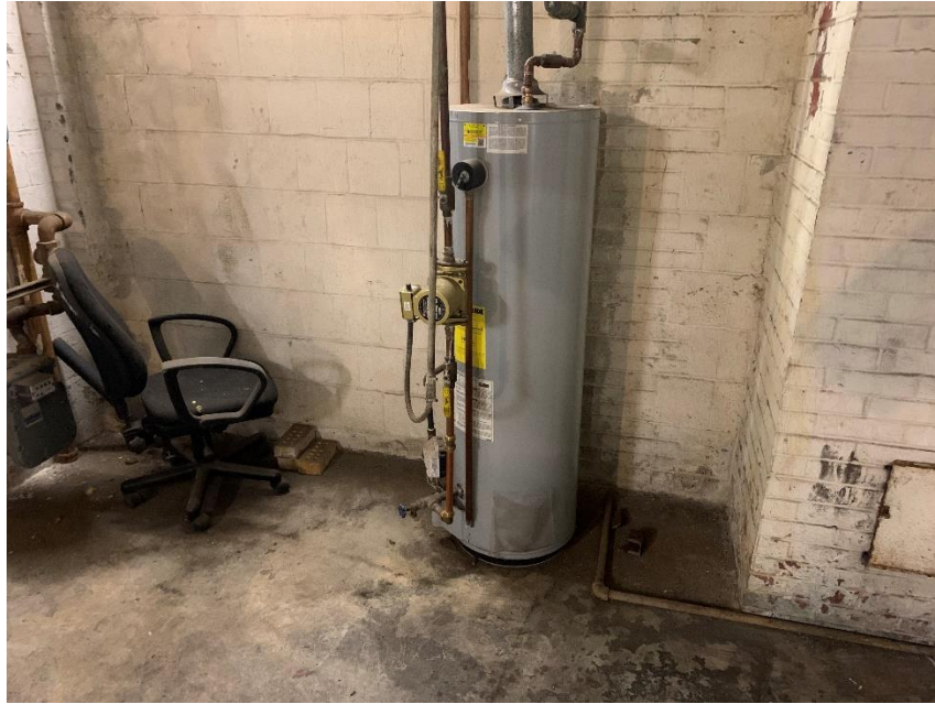
Domestic water heater (boiler) in the basement of the subject property building.
