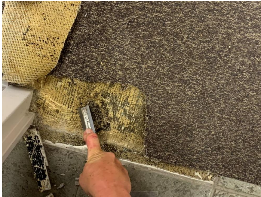
Homogeneous Material No. 21 – ACM Tan carpet glue with black mastic Located Throughout the offices on the Building 3 rd floor of the Subject Property
