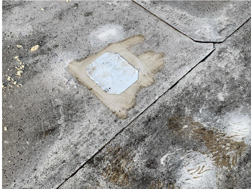
Homogeneous Material No. 1 – Non-ACM Built up Roof Field located on the roof of the Subject Property
