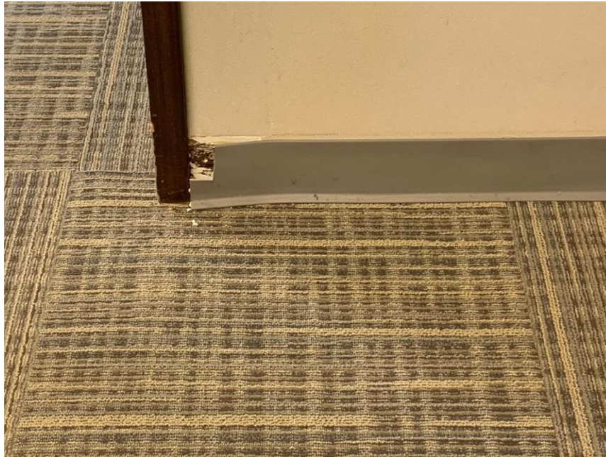
Homogeneous Material No. 15 – Non-ACM 4" Brown Vinyl Cove Base with Brown Mastic Located in the Building Main Floor, Flooring in Some of the Office Area on West Side of Building and Central Customer Area of the Subject Property
