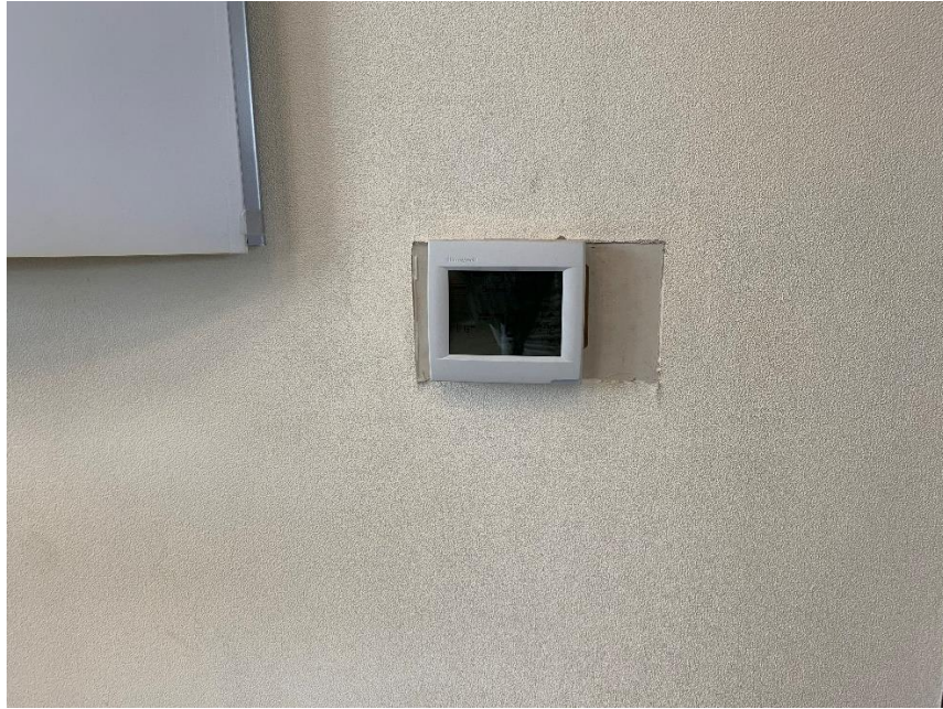
Typical digital thermostat at the subject property building.
