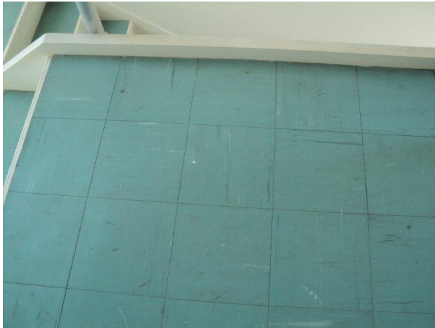
Homogeneous Material No. 20 – ACM 9” by 9” Green Vinyl Floor Tile with Black Mastic located in the building stairwell on East Side
