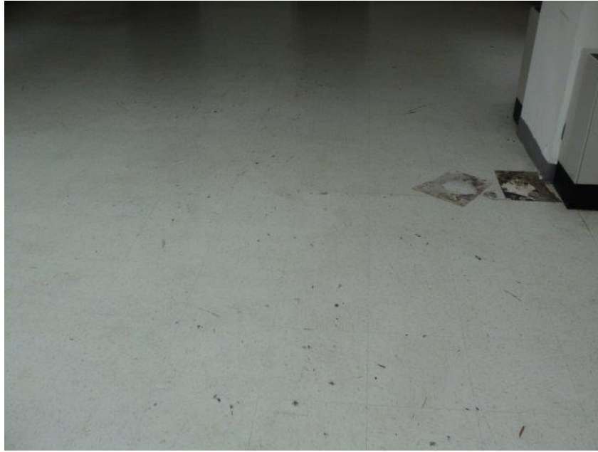
Homogeneous Material No. 19 – ACM 12” by 12” White Mottled Vinyl Floor Tile with Black Mastic and Gray/White Leveling Compound located throughout the Building 2 nd Floor Office space of the Subject Property
