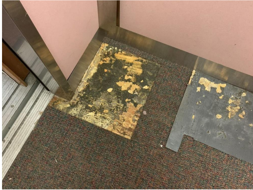
Homogeneous Material No. 9 – Non-ACM Black/Gray/Yellow Mastic located in the Building Elevator of the Subject property
