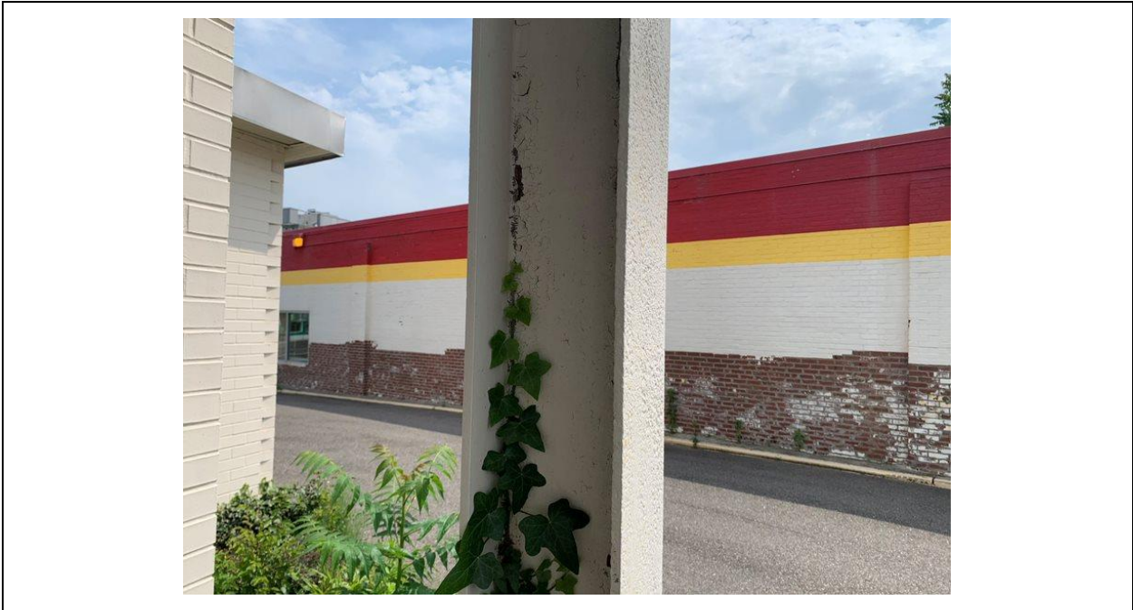
Lead-Containing Paint on the cream metal I-beam at the building rear and front entrance.
