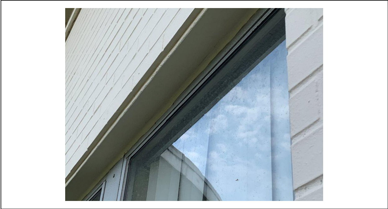
Lead-Containing Paint on the white metal window lintel at the building front entrance.
