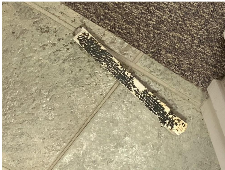
Homogeneous Material No. 22 – ACM White Setting Bed with Black Mastic located in the Building 3 rd Floor Break Room on West Side and throughout the 3 rd floor office areas of the Subject Property
