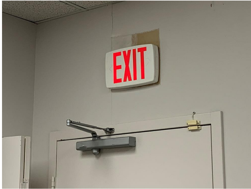
Typical Lighted Exit Sign at the subject property building.
