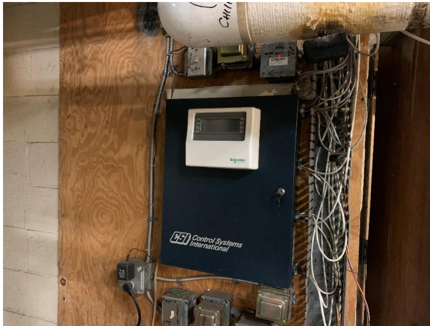
Fire Control Panel at the subject property building.
