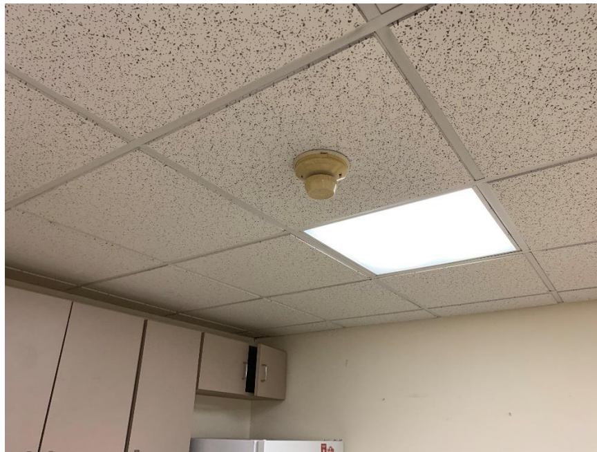
Typical Ceiling-Mounted Smoke Detector at the subject property building.
