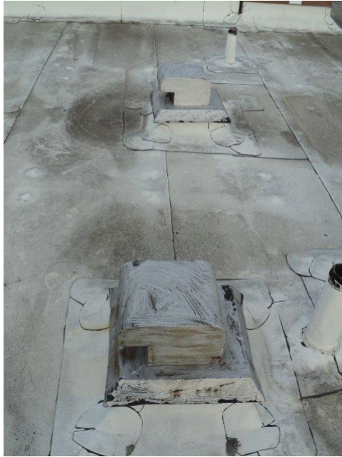
Homogeneous Material No. 3 – ACM Silver Roof Vent Coating located on the roof of the Subject Property
