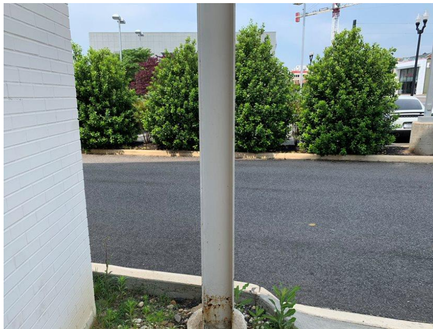
Lead-Containing Paint on the white metal column at the building front entrance.
