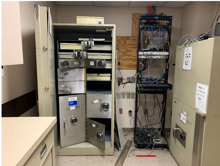
Wireless Control System components at the subject property building.
