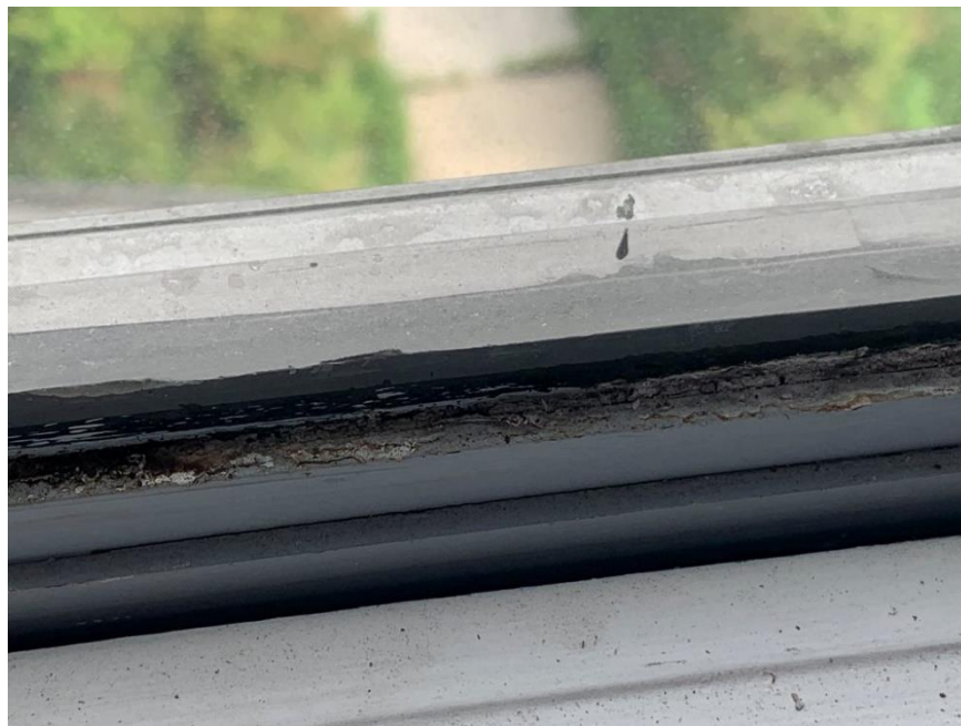
Homogeneous Material No. 24 – ACM Gray Interior Window Glazing Located in the interior windows on the 3rd floor and throughout the building of the subject property
