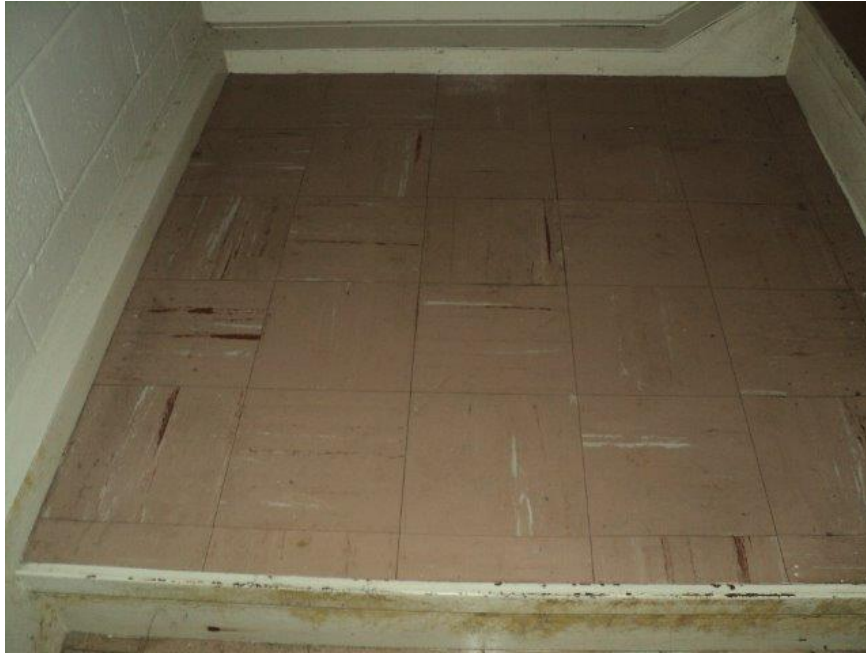
Homogeneous Material No. 7 –ACM 9” by 9” brown vinyl floor tile with black mastic located in the West Side of the Building Stairwell of the Subject Property
