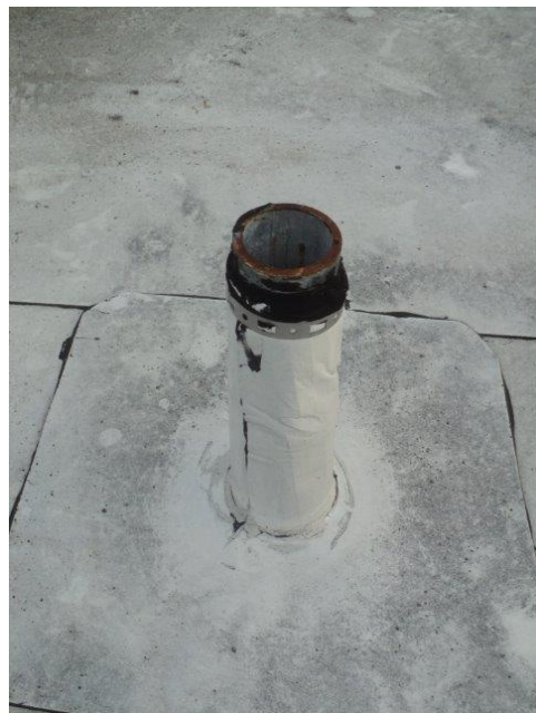
Homogeneous Material No. 4 – Non-ACM Black Vent Pipe Mastic located in the roof of the Subject Property
