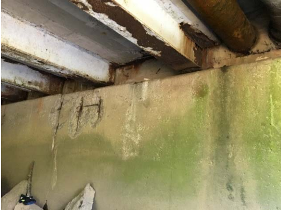
Photo 11– Spall and Delamination at Rear Abutment
