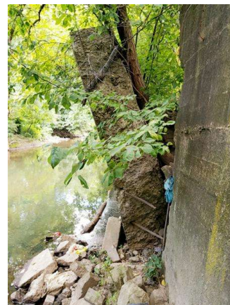
Photo 6 Severed retaining wall at southwest corner
