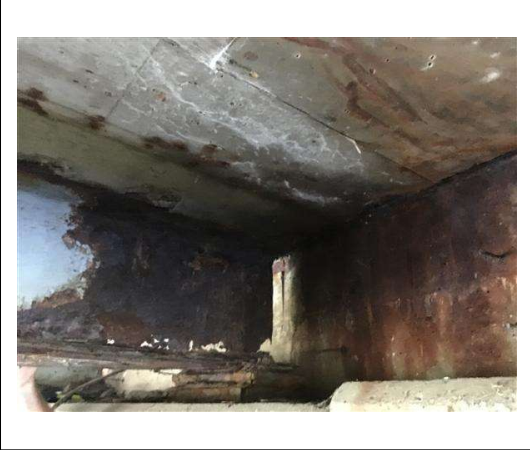
Photo 13 Failed paint at beam ends
