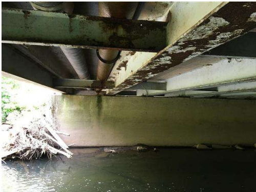
Photo 9 | Section loss to diaphragm supporting utility conduits
