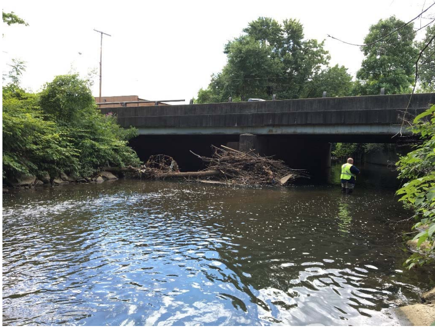
Photo 17– Timber Debris at North Side of Pier
