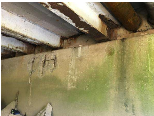
Photo 11 | Spalling with exposed rebar at West Abutment
