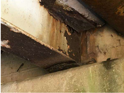
Photo 7 | Beam end deterioration
