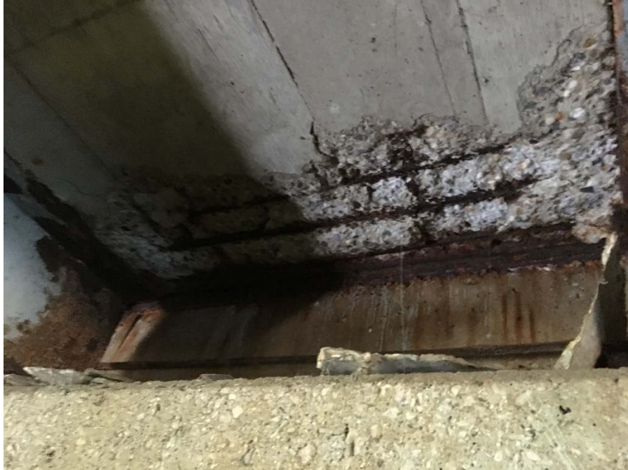
Photo 9– Spalling of deck ends with exposed rebar with section loss
