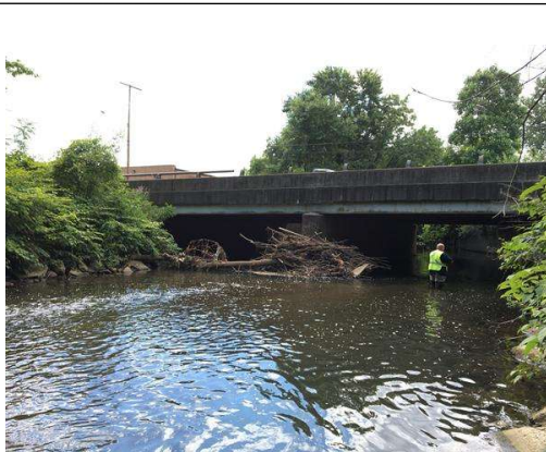
Photo 5 North Elevation with debris accumulation at Pier
