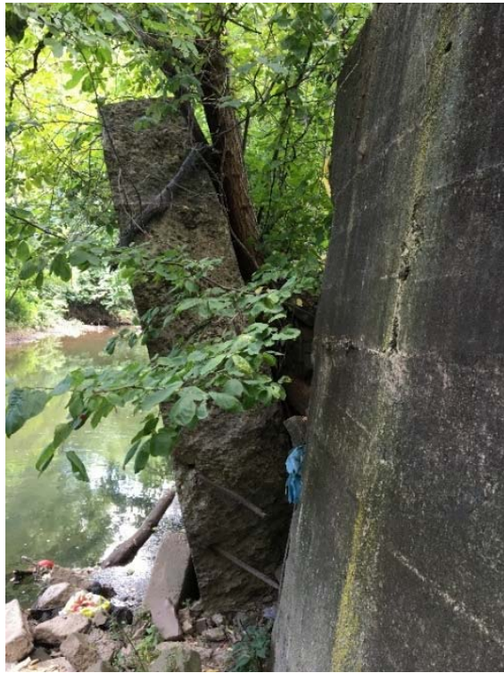
Photo 14 – Southwest Retaining Wall rotated outward
