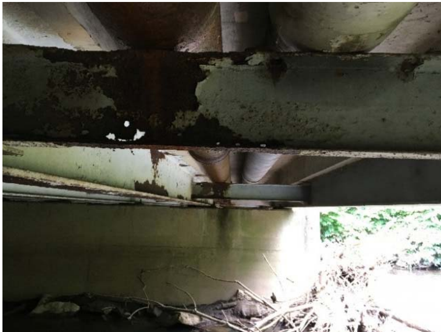
Photo 10 – Cross Frames Section Loss between Beam 1 & 2
