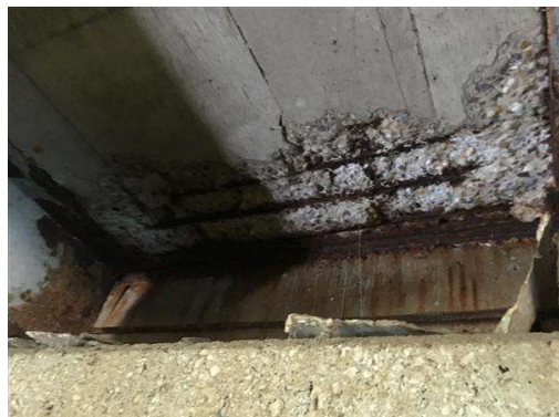
Photo 12 | Spalling with exposed corroded rebar at deck ends.
