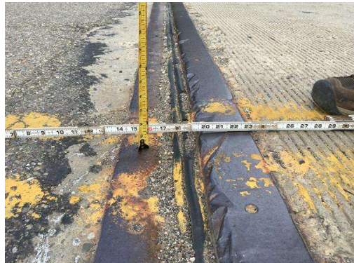
Photo 10 | Settlement at West approach
