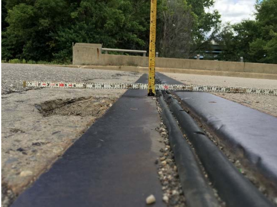
Photo 5 – Settlement at Rear Abutment Joint
