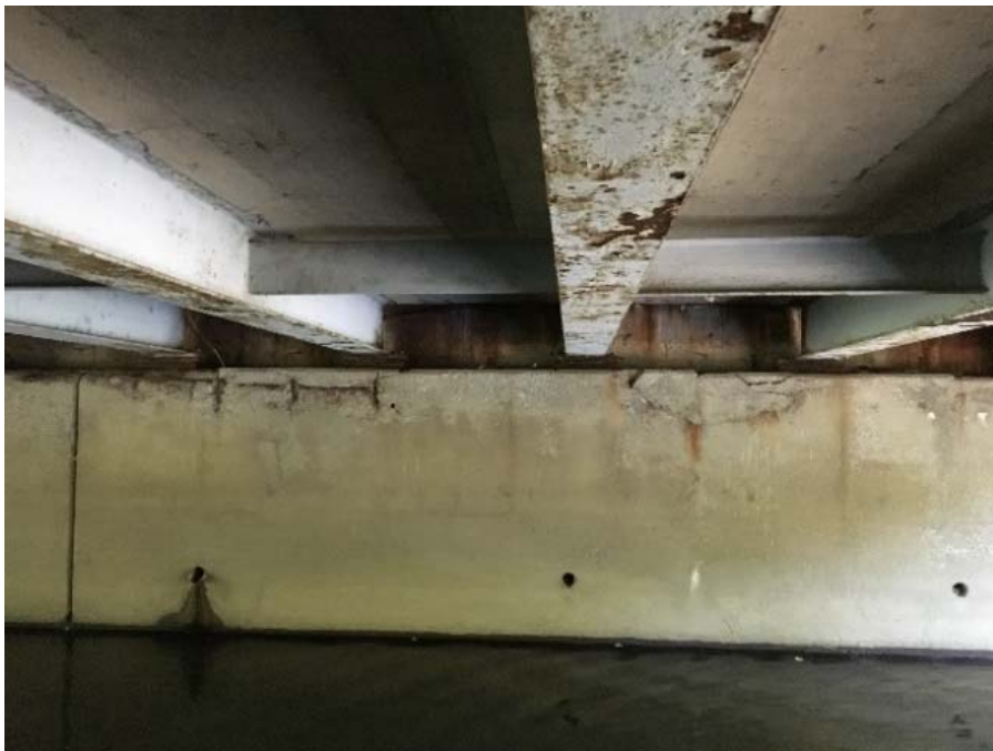
Photo 12 – Spall and Delamination at Forward Abutment
