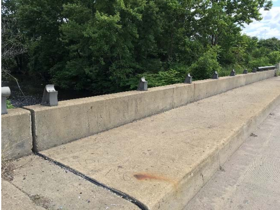
Photo 7 – Missing North Railing
