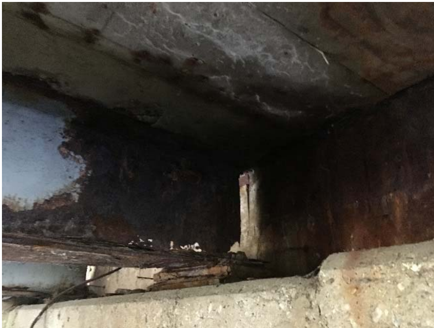
Photo 8 – Section loss in Beam 10 at Rear Abutment
