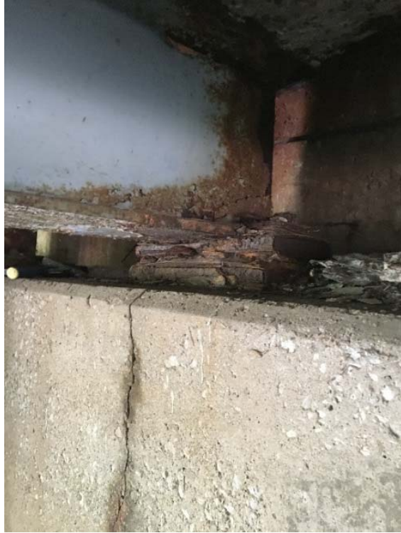
Photo 13 – Section Loss at Bearing (typ.)
