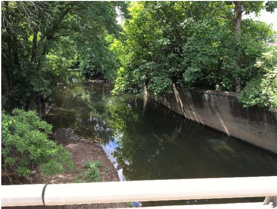
Photo 16 – Southwest Retaining Wall Rotated towards Creek (looking downstream)
