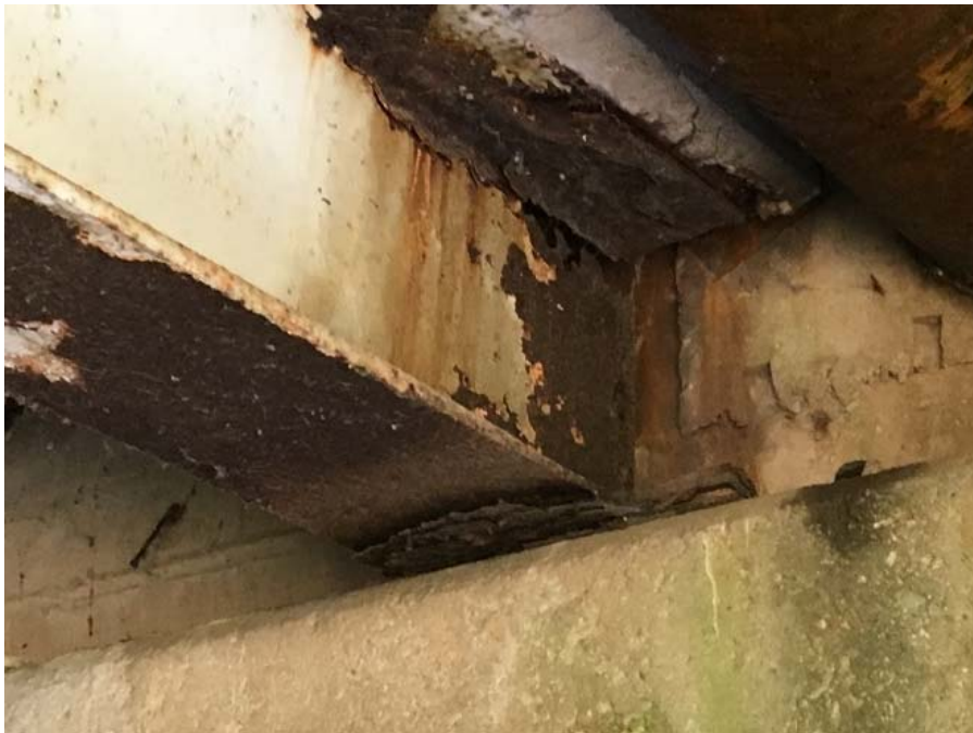
Photo 6 – Section loss in Beam 2 at Rear Abutment
