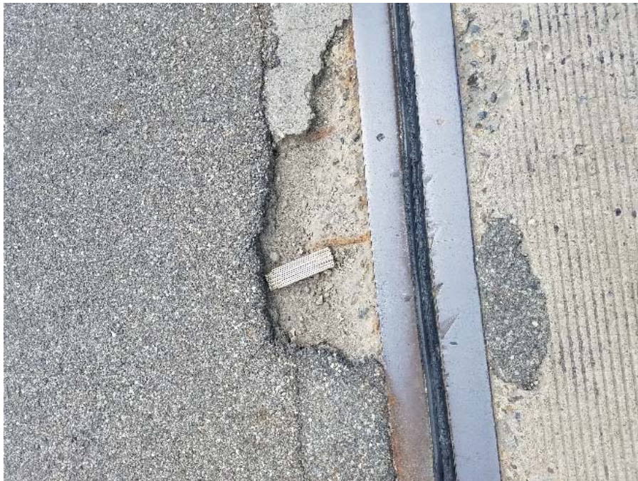
Photo 4 – Pothole near Joint
