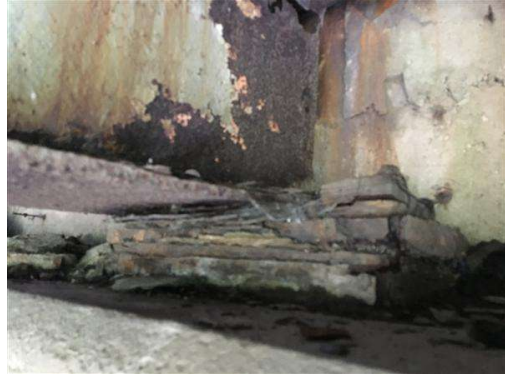
Photo 8 | Severe deterioration of bearings
