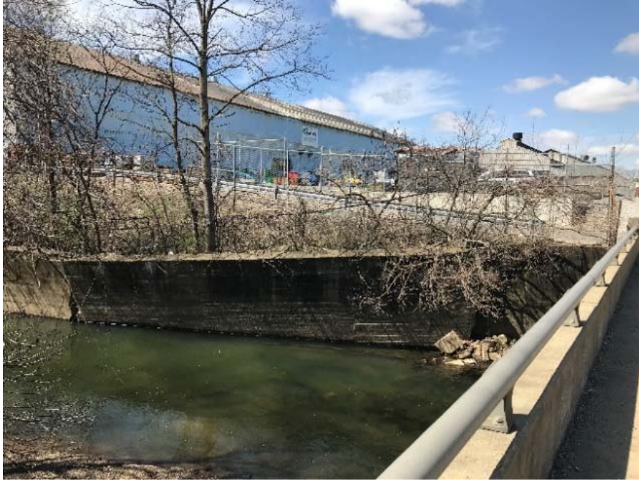
Photo 15 – Southwest Retaining Wall rotated outward
