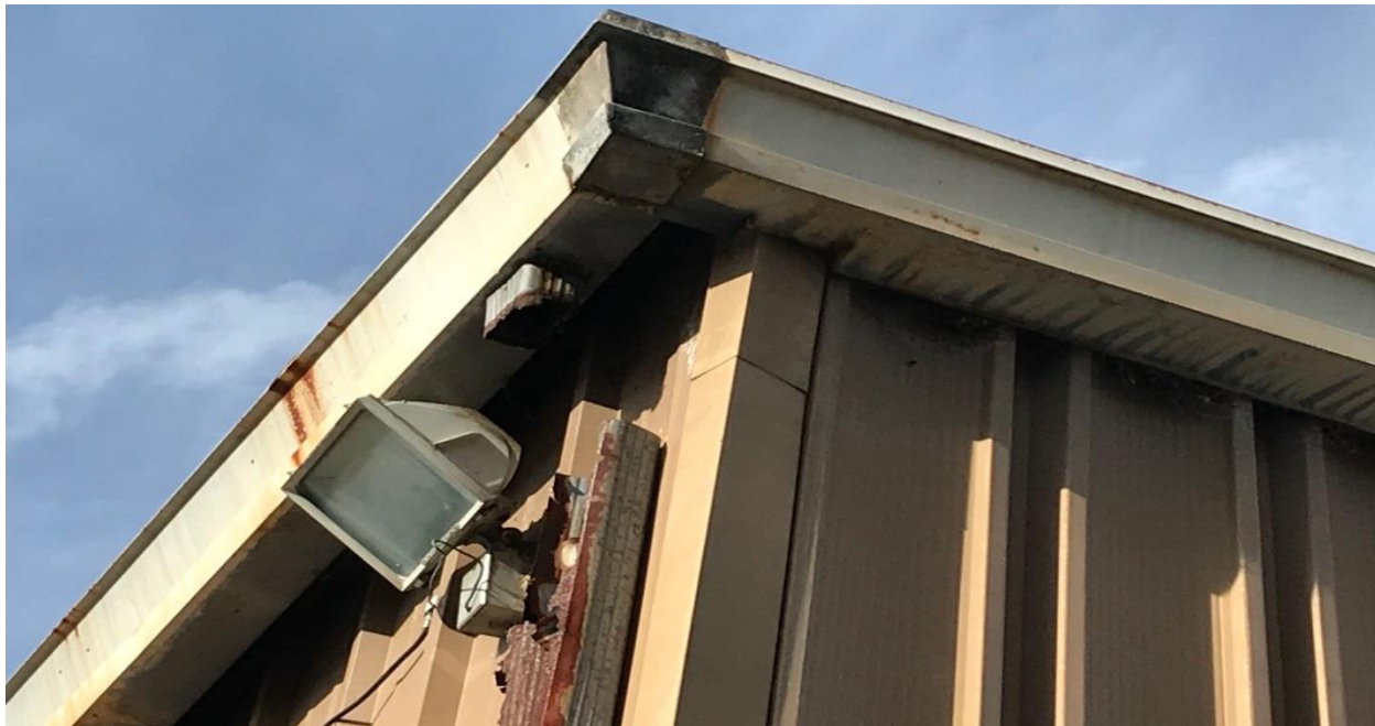
Rusted gutters and downspouts typical condition at all 4 corners
