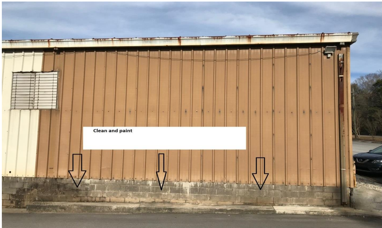
Fleet service side of building . Note rusted gutters and 2 tone metal panels . Clean and paint concrete base.
