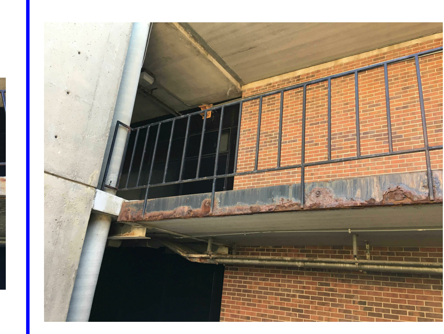
D13 Scale No Scale Elevated Walkway & Guardrail
