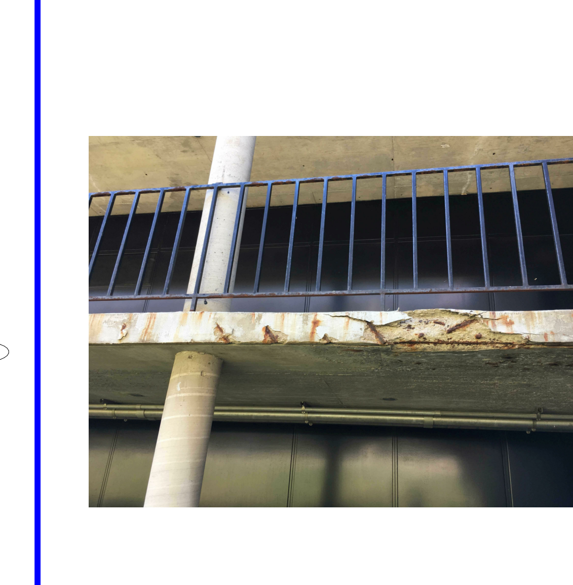
D10 Scale No Scale Elevated Walkway & Guardrail
