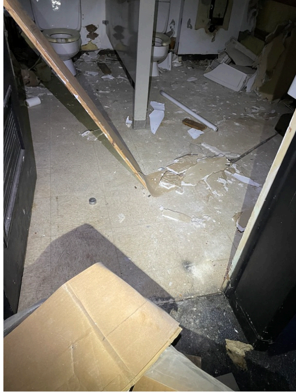
General view of asbestos-containing Black Mastic beneath 12" x 12" Tan Floor Tile (HA 215)
