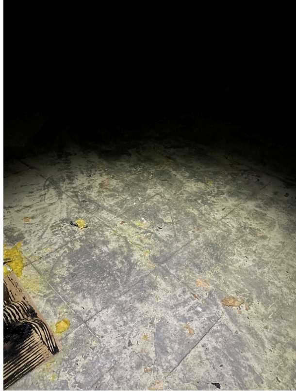
View of asbestos-containing 12" x 12" Grey/Brown Floor Tile and its associated Black Mastic (HA 37)
