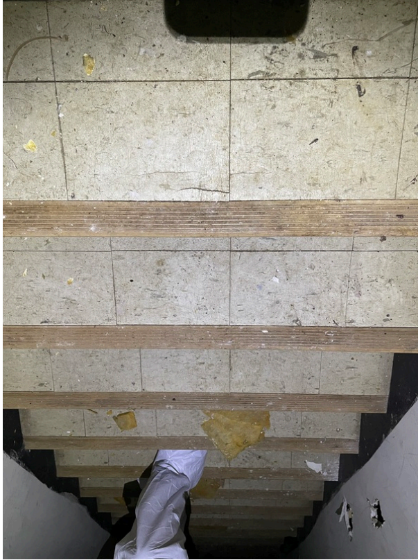
View of asbestos-containing 9" x 9" Tan Floor Tile and its associated Black Mastic (HA 207)
