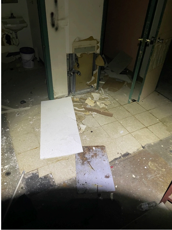
General view of asbestos-containing Black Mastic beneath 12" x 12" Tan Floor Tile (HA 138)
