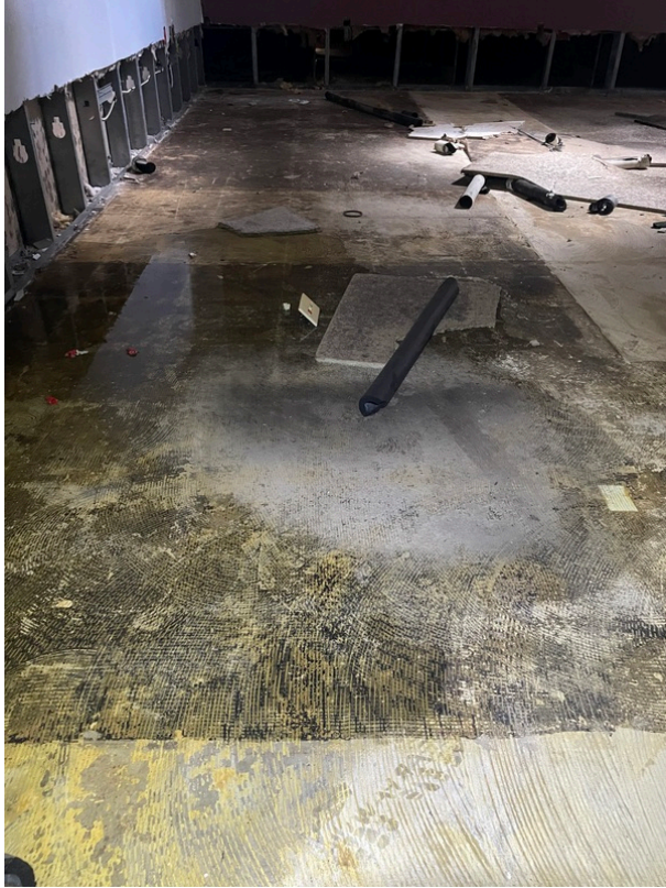
View of asbestos-containing Black/Yellow Mastic (HA 160)
