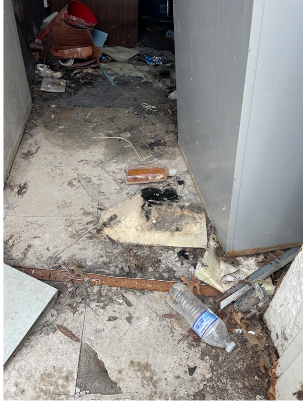
General view of asbestos-containing Black Mastic beneath 12" x 12" Brown Floor Tile (HA 217)
