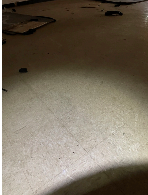
General view of asbestos-containing 9" x 9" Tan Floor Tile and Black Mastic beneath 12" x 12" Tan with Brown Specks Floor Tile (HA 76)
