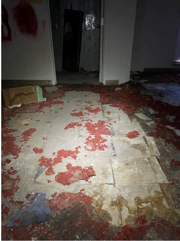
View of asbestos-containing 12" x 12" Brown/Off-White Floor Tile and its associated Black Mastic (HA 43)
