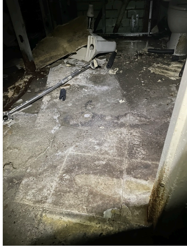
General view of asbestos-containing Black Mastic beneath 12" x 12" Grey Floor Tile (HA 139)
