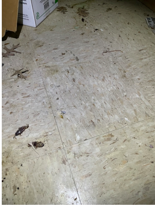
General view of asbestos-containing Black Mastic beneath 12" x 12" Tan with White Specks Floor Tile (HA 50)
