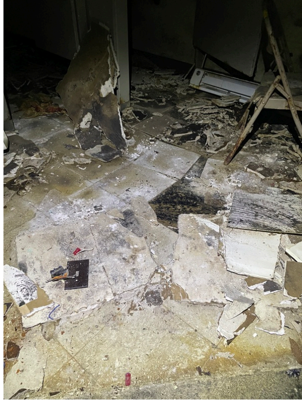
General view of asbestos-containing Black Mastic beneath 12" x 12" Tan Floor Tile (HA 206)
