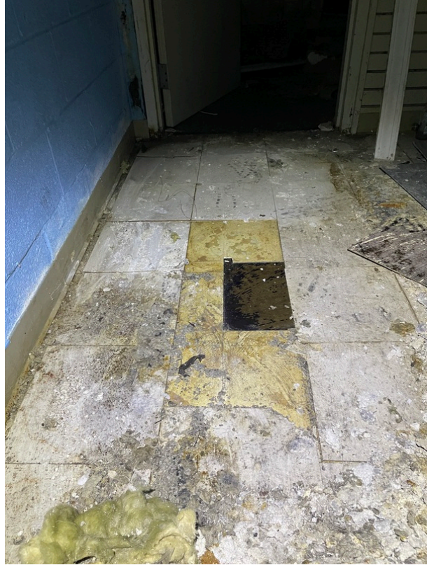
General view of asbestos-containing 12" x 12" Tan Floor Tile and Black Mastic beneath 12" x 12" Off-White Floor Tile (HA 126)
