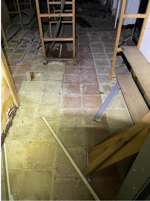
General view of asbestos-containing Black Mastic beneath 12" x 12" Red Floor Tile (HA 195)
