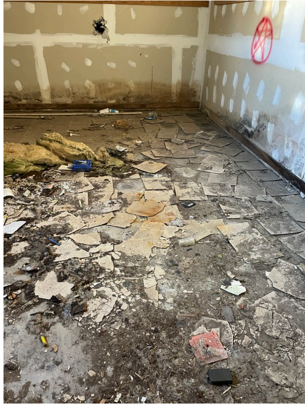
General view of asbestos-containing Black Mastic beneath 12" x 12" Tan Floor Tile (HA 178)
