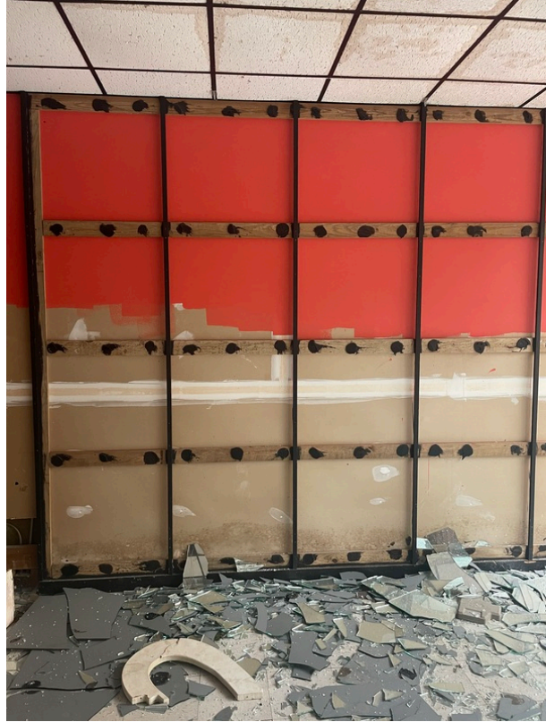
View of asbestos-containing Black Mastic Dot (HA 152)
