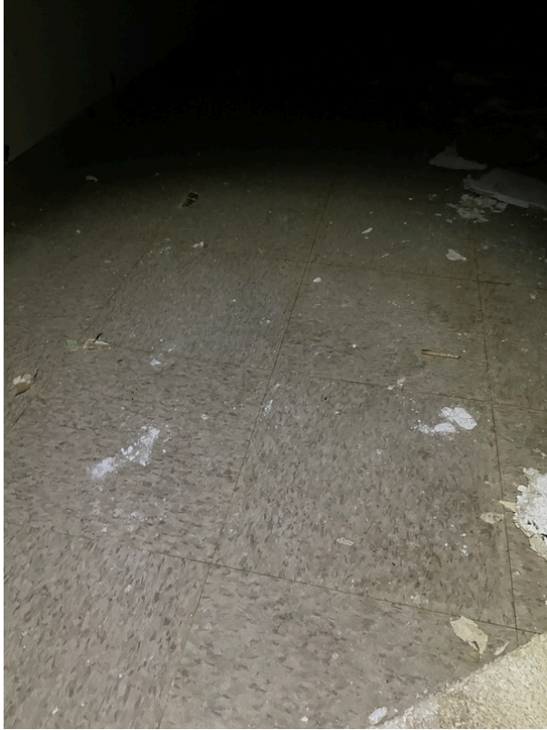
General view of asbestos-containing Black Mastic beneath 12" x 12" Tan Floor Tile (HA 68)
