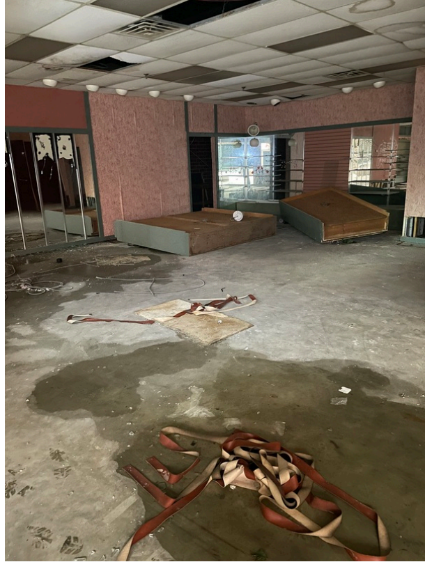
View of asbestos-containing Black Mastic Dot (HA 166)
