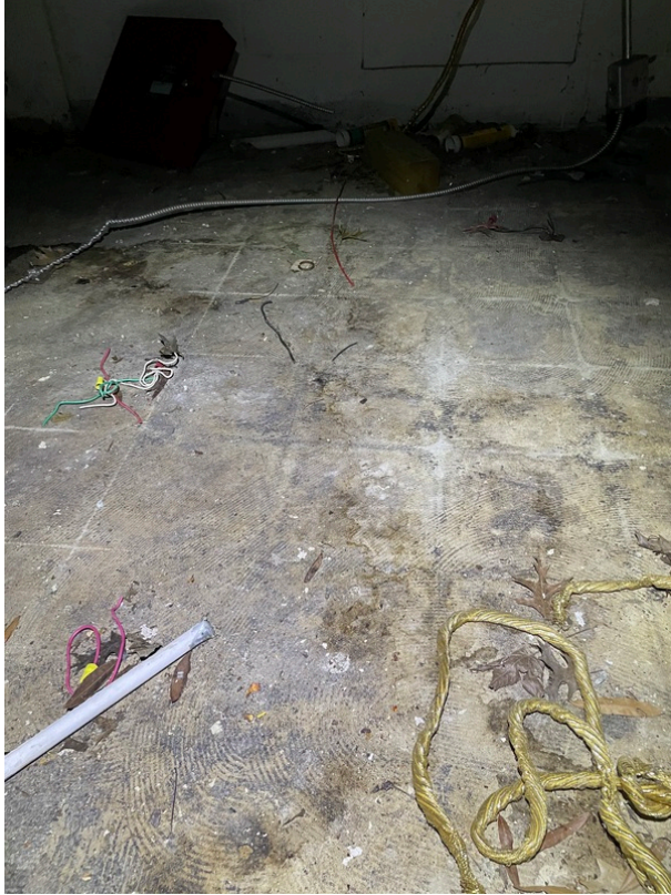
View of asbestos-containing Black Mastic (HA 204)
