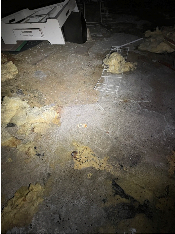
View of asbestos-containing Yellow/Black Carpet Glue (HA 188)
