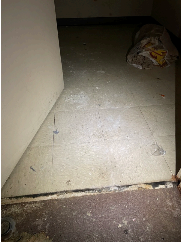
General view of asbestos-containing Black/Tan Mastic beneath 12" x 12" Tan with Brown Specks Floor Tile (HA 75)
