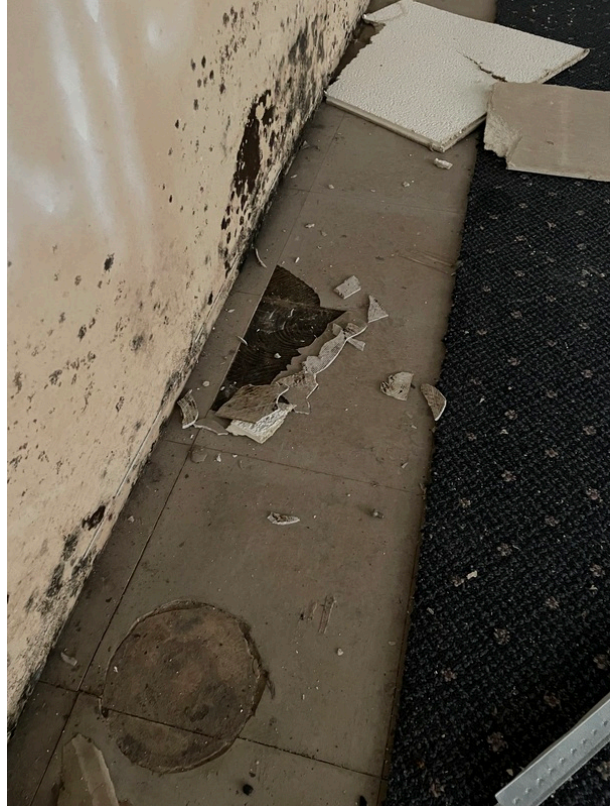
View of asbestos-containing Black/Tan Mastic beneath 12" x 12" Dark Grey Floor Tile (HA 35)
