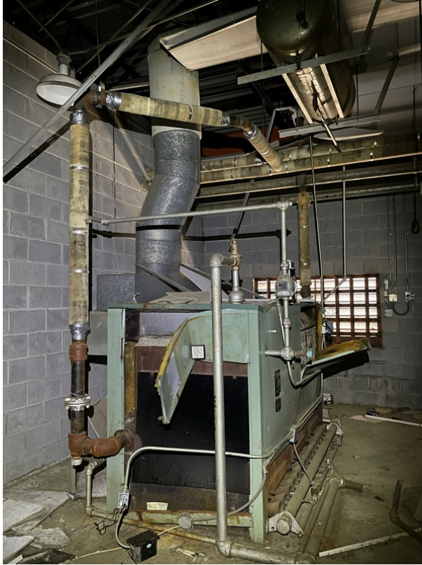
View of a boiler assumed to be asbestos-containing (HA 227)
