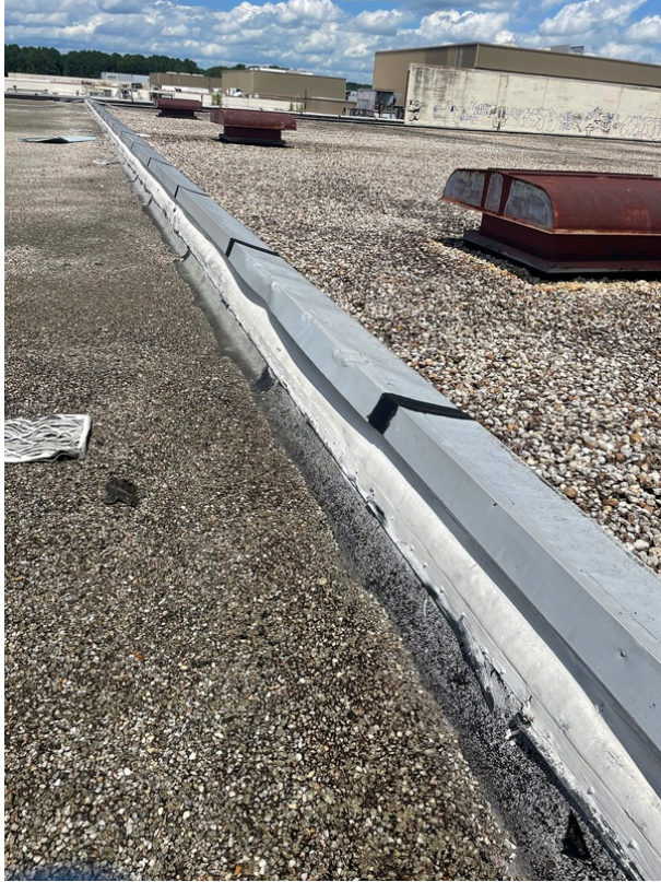
General view of asbestos-containing Black Tarpaper beneath White/Black Rolled Shingle and Black Tar (HA 21)
