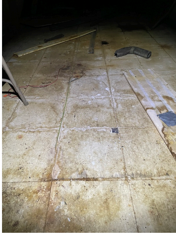
General view of asbestos-containing Black Mastic beneath 12" x 12" Off-White with Brown Specks Floor Tile (HA 208)
