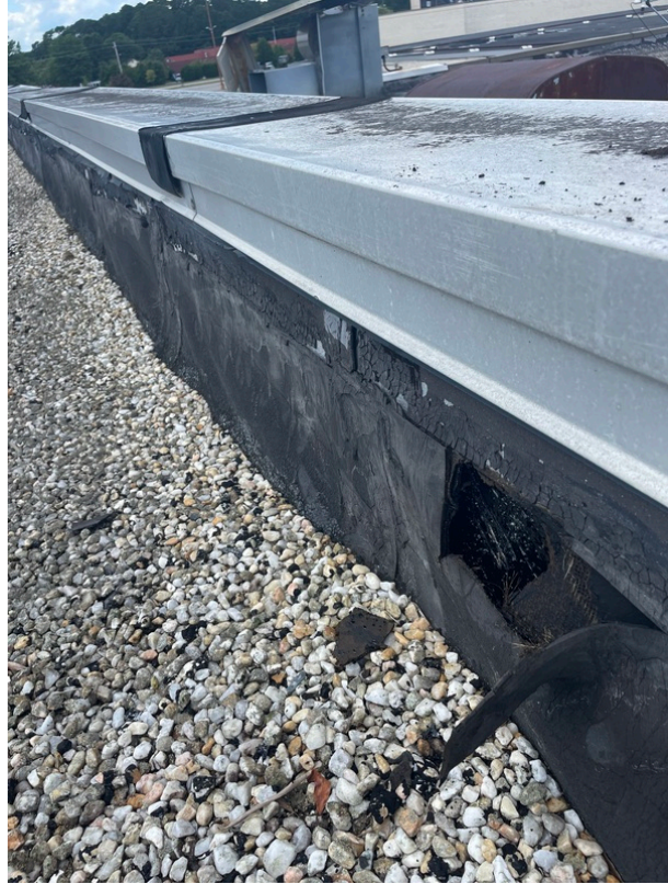
General view of asbestos-containing Black Tarpaper beneath Black Tar (HA 20)
