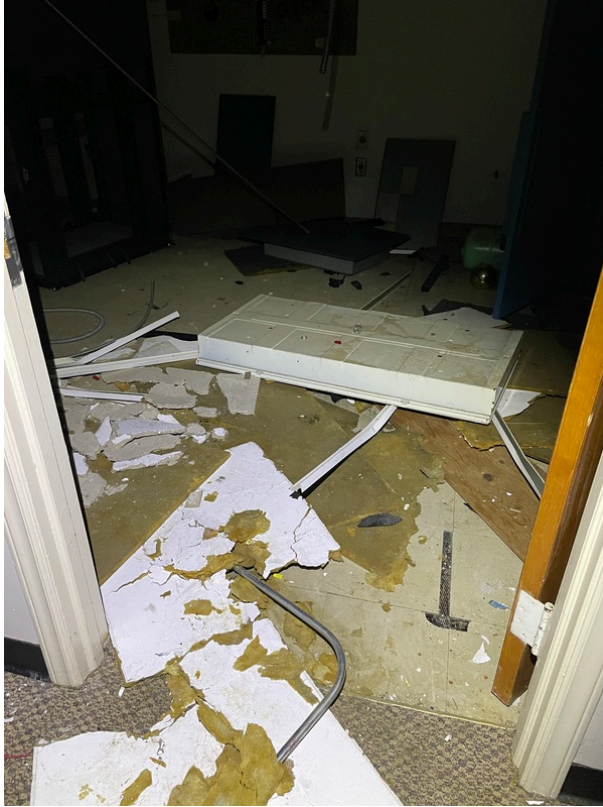
View of asbestos-containing 12" x 12" Tan with Dark Streaks Floor Tile and its associated Black Mastic (HA 46)
