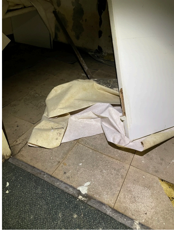
General view of asbestos-containing Yellow/Black Mastic beneath 12" x 12" Tan Floor Tile (HA 183)
