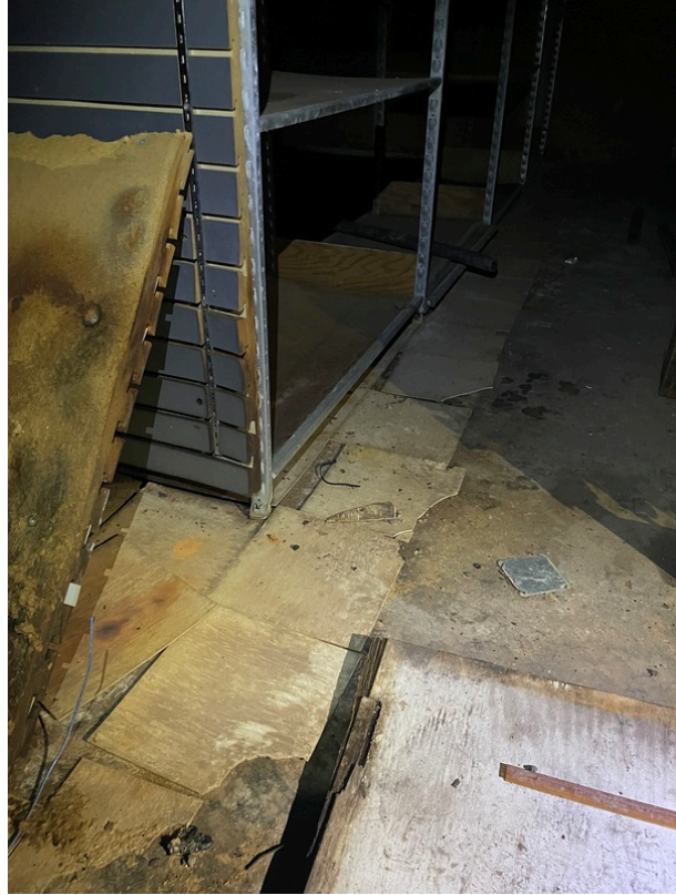
View of asbestos-containing 12" x 12" Tan Floor Tile and its associated Black Mastic (HA 180)
