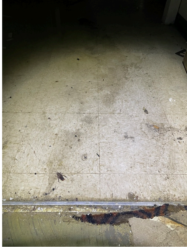
General view of asbestos-containing Black Mastic beneath 12" x 12" Off-White Floor Tile (HA 146)
