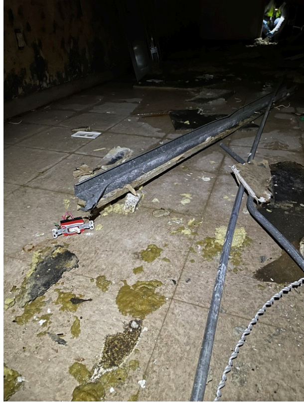
General view of asbestos-containing Black Mastic beneath 12" x 12" Tan Floor Tile and Grey Leveling Compound (HA 107)
