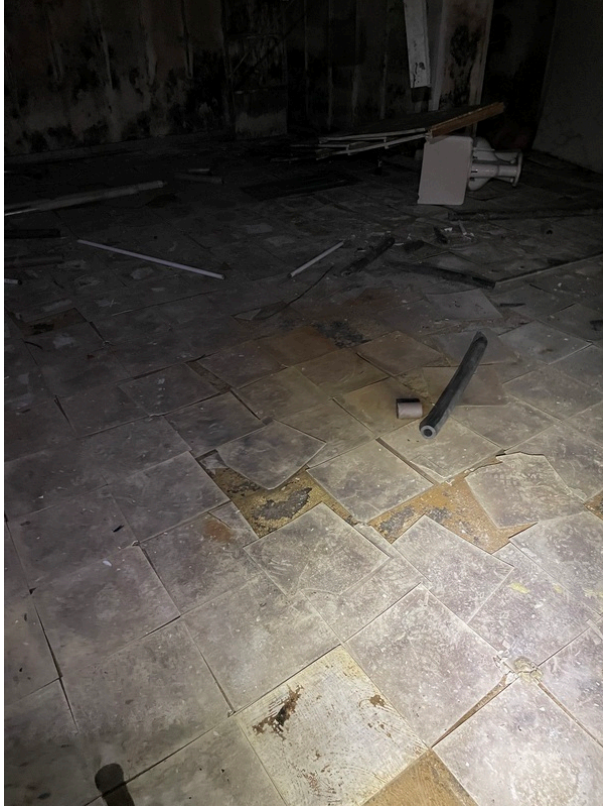
General view of asbestos-containing 12" x 12" Beige Floor Tile and its associated Black Mastic beneath 12" x 12" Tan Floor Tile (HA 184)
