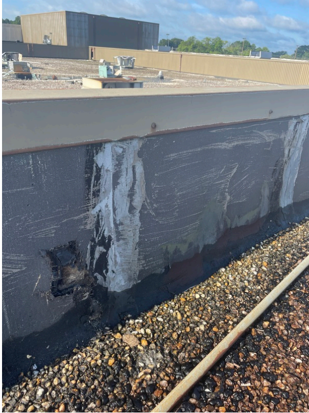
General view of asbestos-containing Grey Tar and Black Tarpaper (HA 5)
