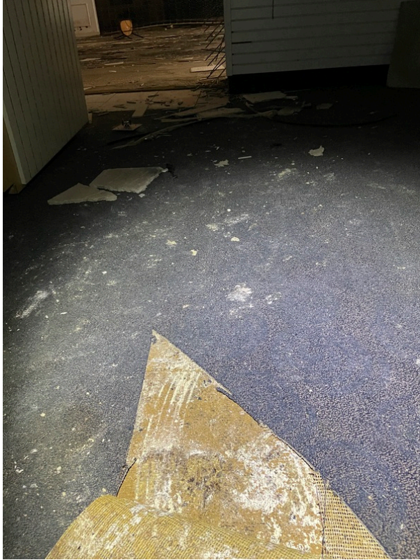
View of asbestos-containing Yellow/Black Carpet Glue (HA 193)
