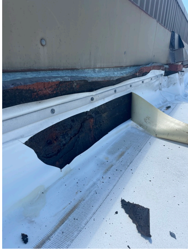
General view of asbestos-containing Black Backing beneath Black Tar (HA 12)
