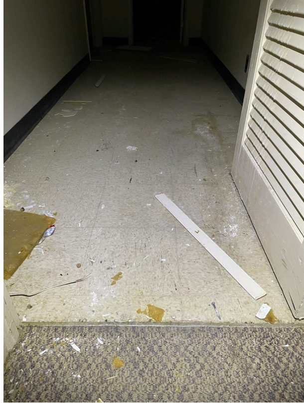
General view of asbestos-containing 12" x 12" Yellow/Off-White Floor Tile and Black Mastic beneath 12" x 12" Tan Floor Tile (HA 45)
