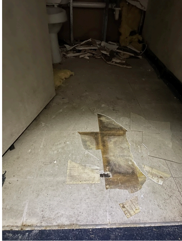
General view of asbestos-containing Black Mastic beneath 12" x 12" Tan Floor Tile and a second Floor Tile layer (HA 79)
