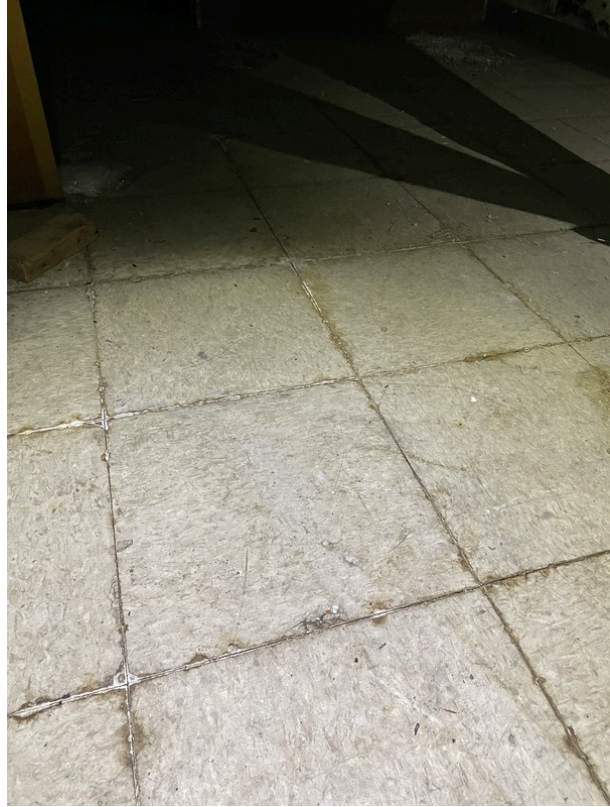
View of asbestos-containing 9" x 9" Grey/ Off-White Floor Tile and its associated Black Mastic (HA 38)
