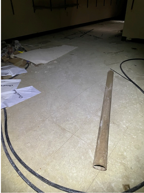
General view of asbestos-containing Black Mastic beneath 12" x 12" Tan Floor Tile (HA 211)
