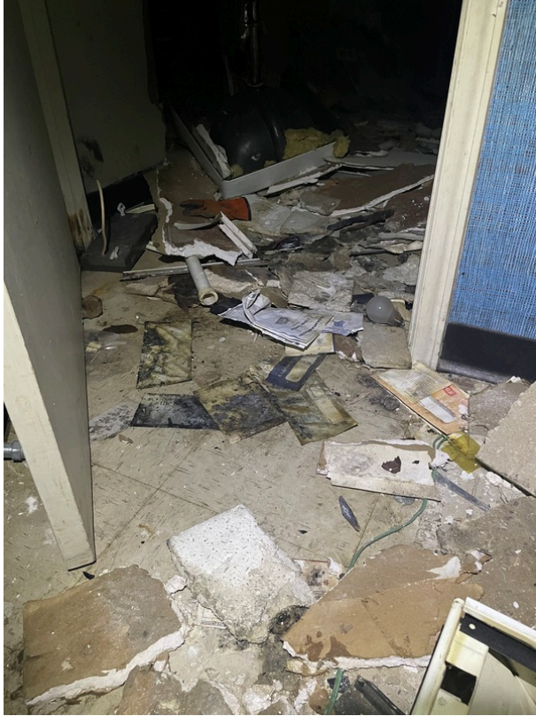
View of asbestos-containing 12" x 12" Off-White Floor Tile and its associated Black Mastic (HA 164)
