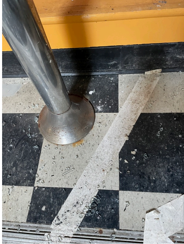
General view of asbestos-containing Black Mastic beneath 12" x 12" Off-White Floor Tile and Grey/Black Leveling Compound (HA 121)
