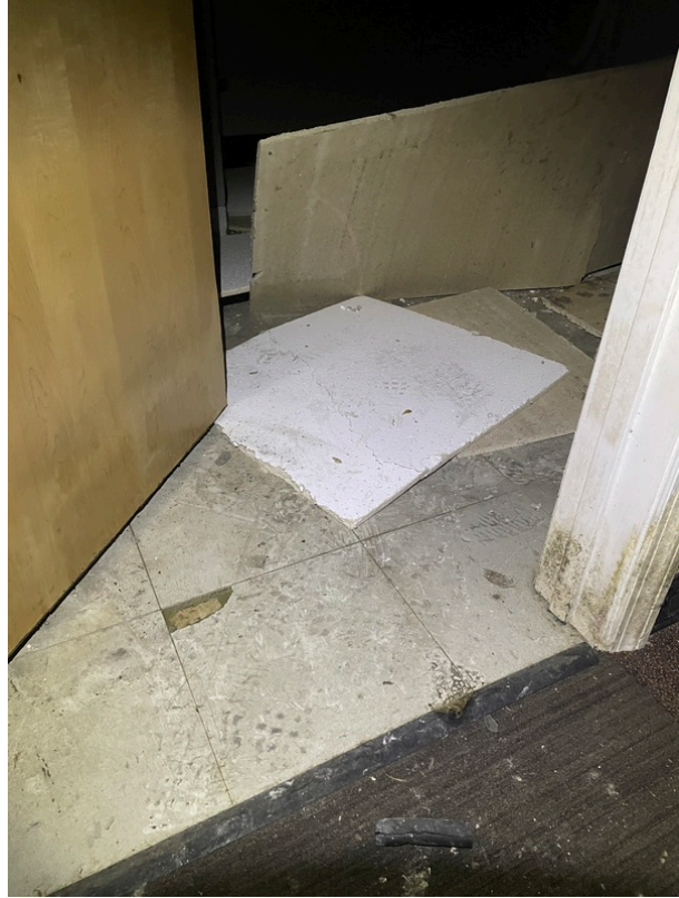
General view of asbestos-containing Black Mastic beneath 12" x 12" Tan Floor Tile (HA 116)
