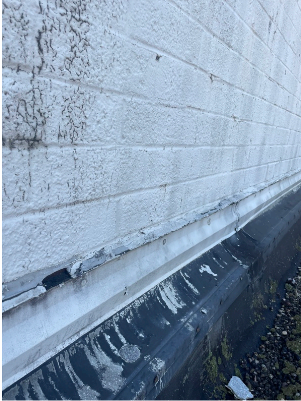
General view of asbestos-containing Black Tar beneath Grey Seam Caulk (HA 9)
