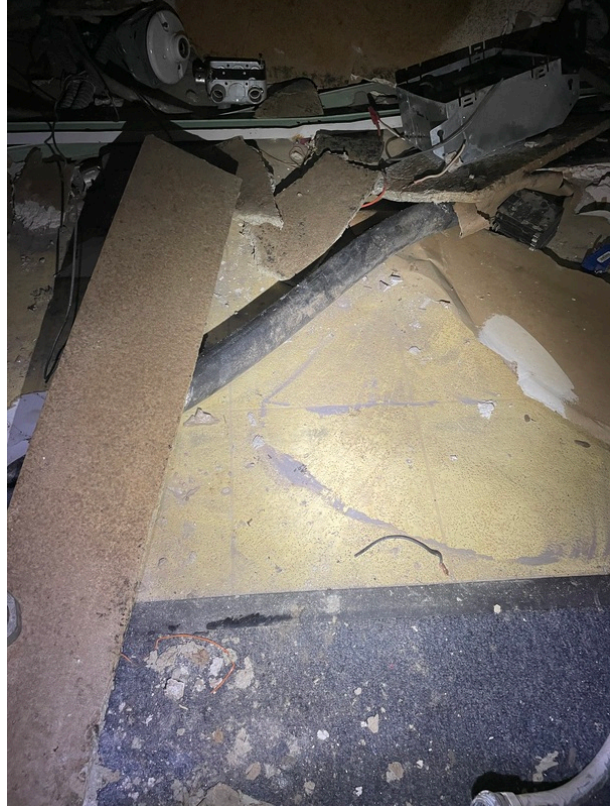
General view of asbestos-containing Tan Floor Tile and Black Mastic beneath Tan Sheet Flooring (HA 97)
