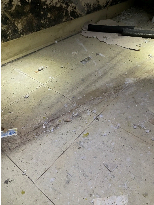
View of asbestos-containing 12" x 12" Off-White Floor Tile and its associated Black Mastic (HA 130) in Room 262
