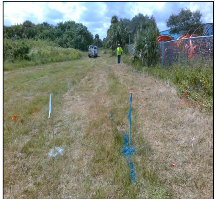
Tie 02 (From Test Hole): COMM HH
