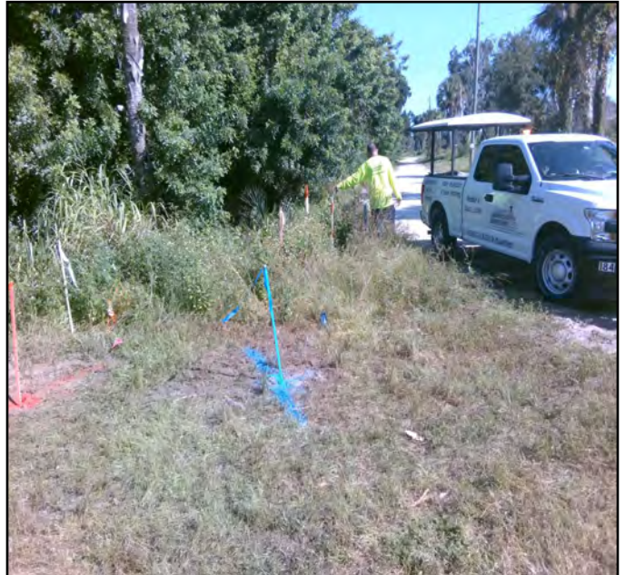
Tie 02 (From Test Hole): NORTH VALVE, WATER
