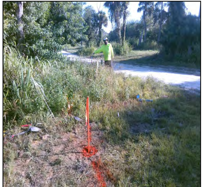
Tie 02 (From Test Hole): NORTH VALVE, WATER
