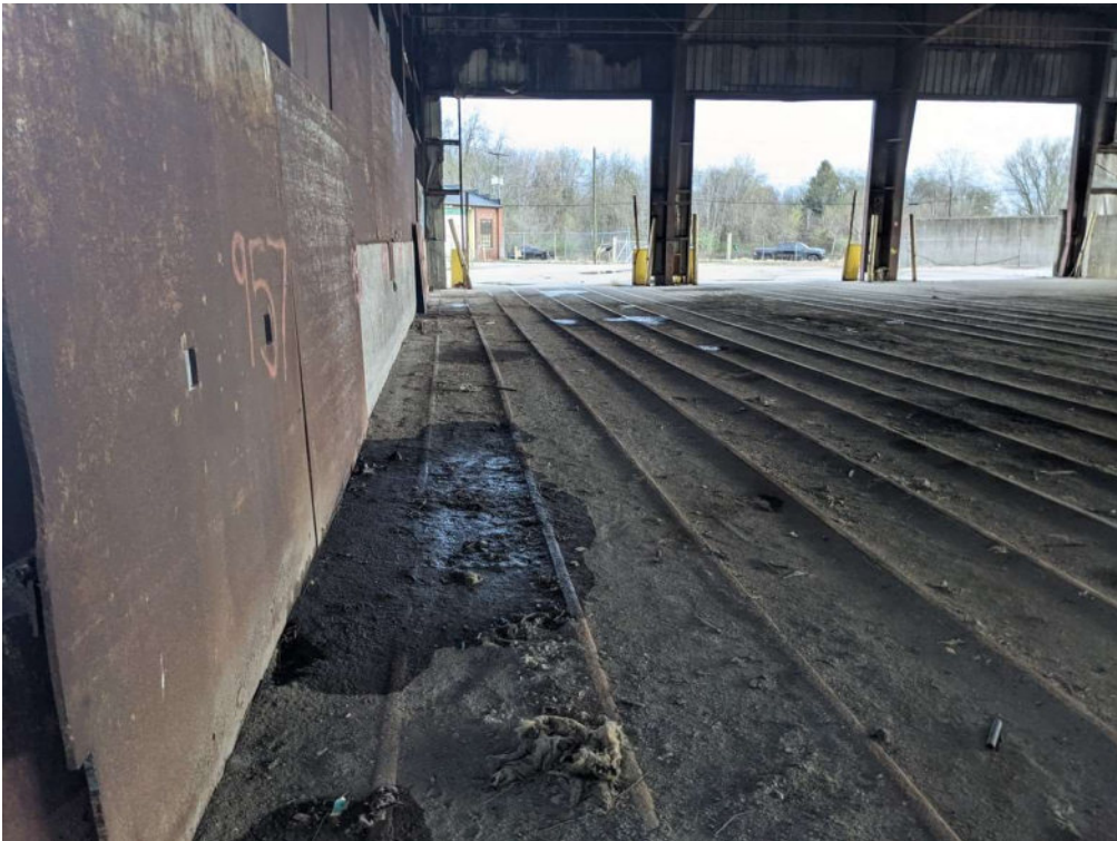
Photo 18. Inside Sorting Building, rails for trash dumpster. Staining present. Site A
