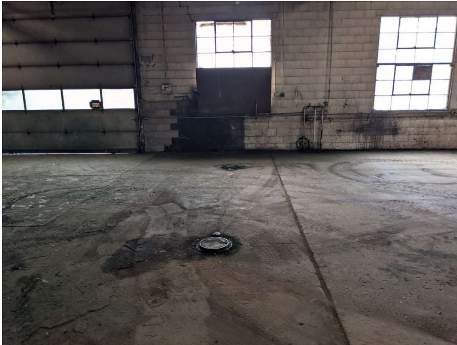
Photo 11. Hydraulic lift pistons inside Maintenance Building. Staining present. Site A
