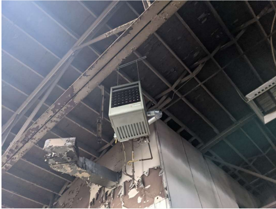
Photo 13. Overhead natural gas heaters in the Maintenance Building. Wall is for the refrigerated rooms. Potential ACM in walls. Site A.
