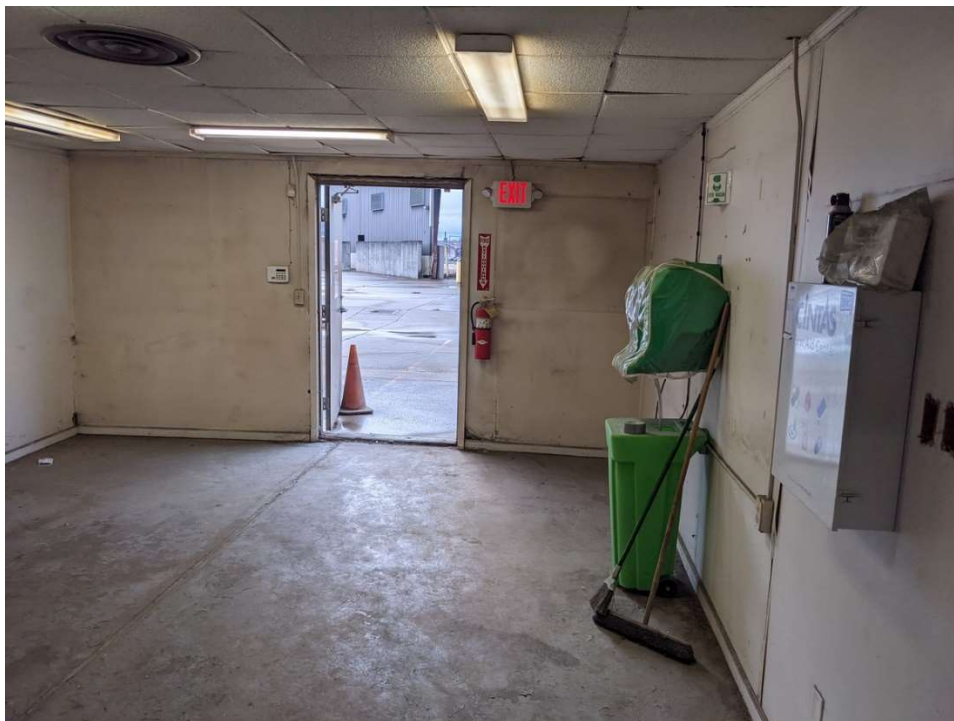
Photo 8. East side entrance of Maintenance Building. ACM potential in ceiling and walls. Site A.
