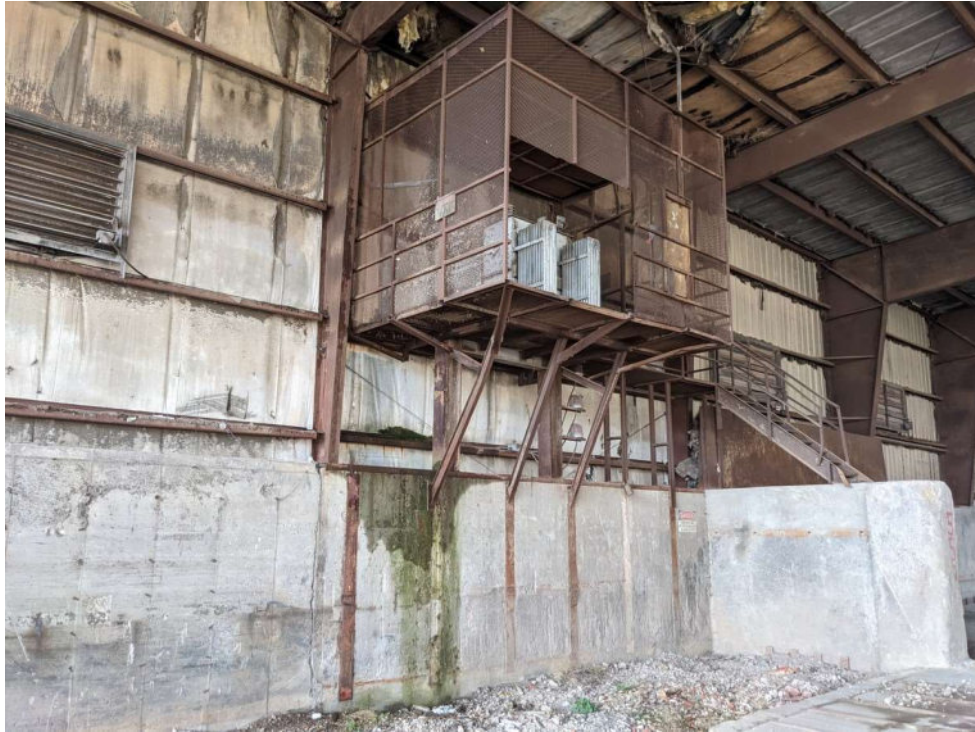
Photo 21. Closeup of transformers in Sorting Building. Staining present on wall and floor. Site A
