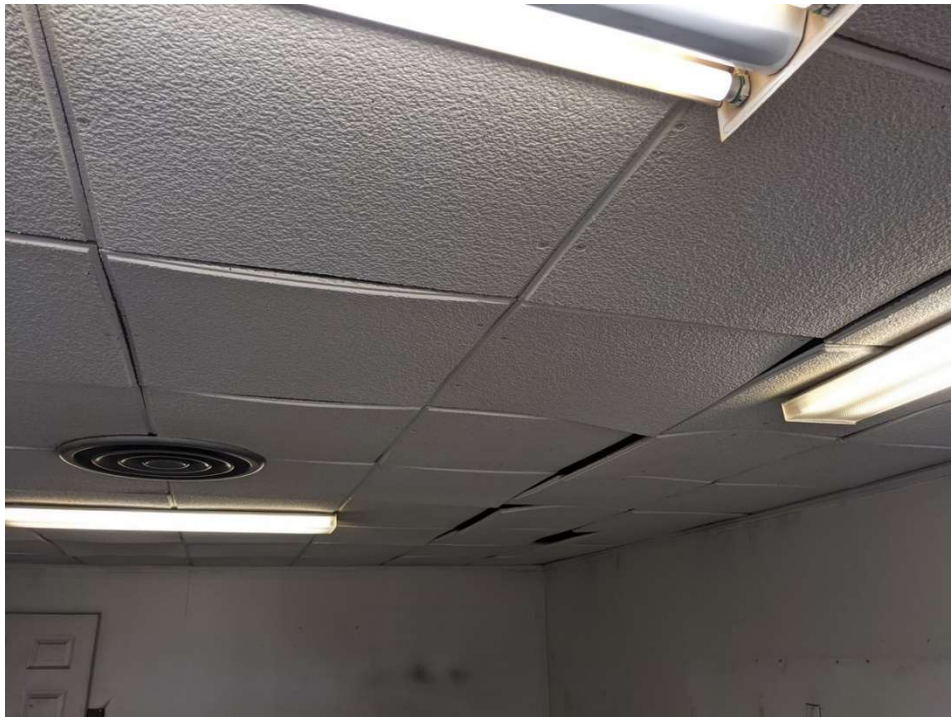
Photo 14. Potential ACM in ceiling tiles inside the Maintenance Building. Site A
