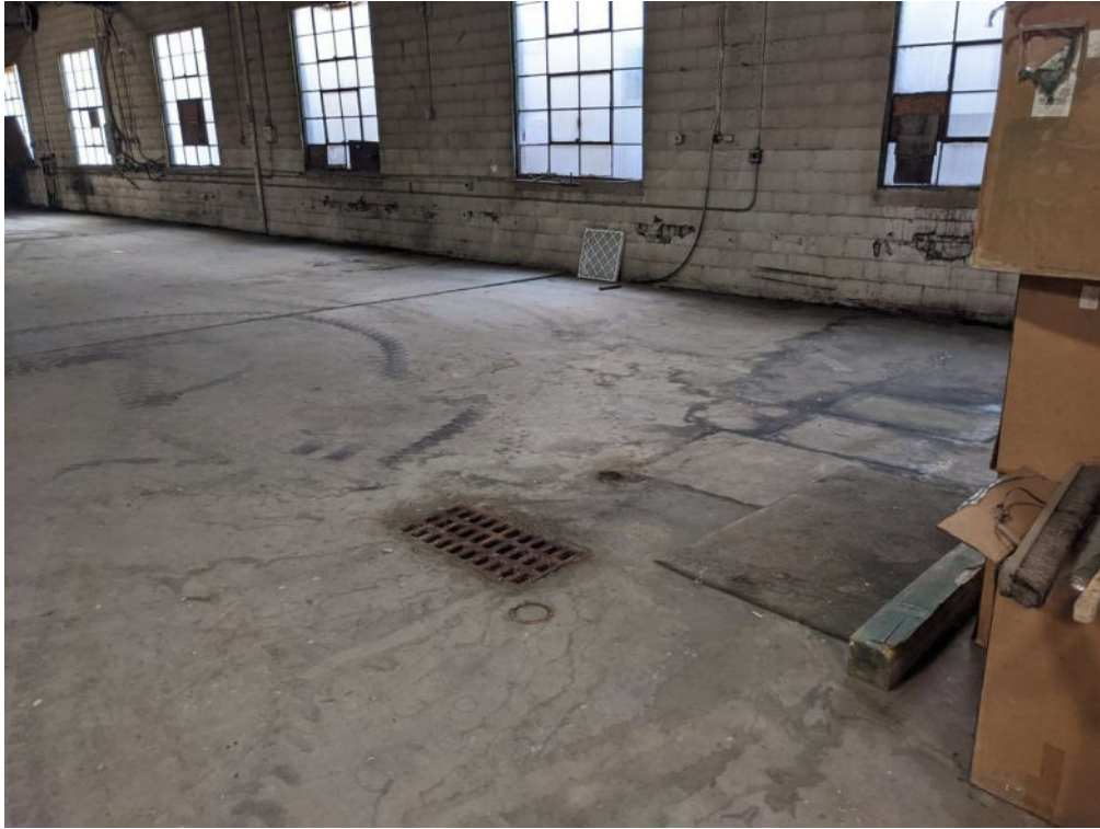
Photo 9. Floor drain inside Maintenance Building, drain to wastewater. Site A.
