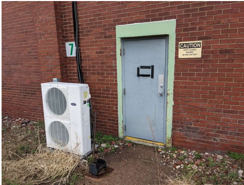
Photo 7. Air conditioning unit on southside of Maintenance Building. Site A
