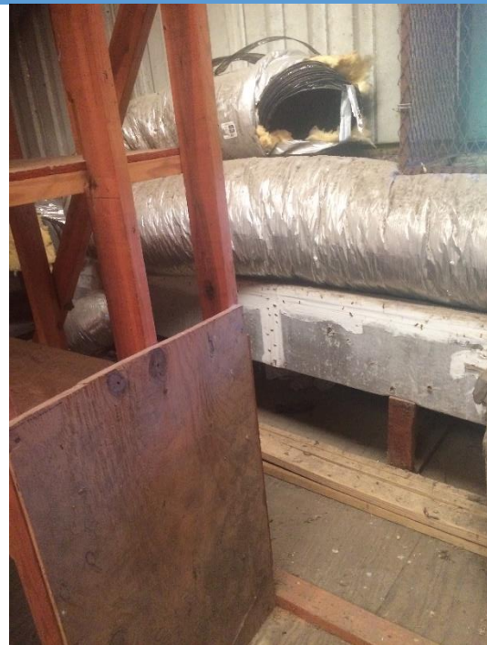
HVAC duct on 2 nd floor
