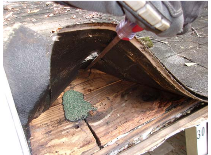
Photo 2 – Roof shingles & no felt
