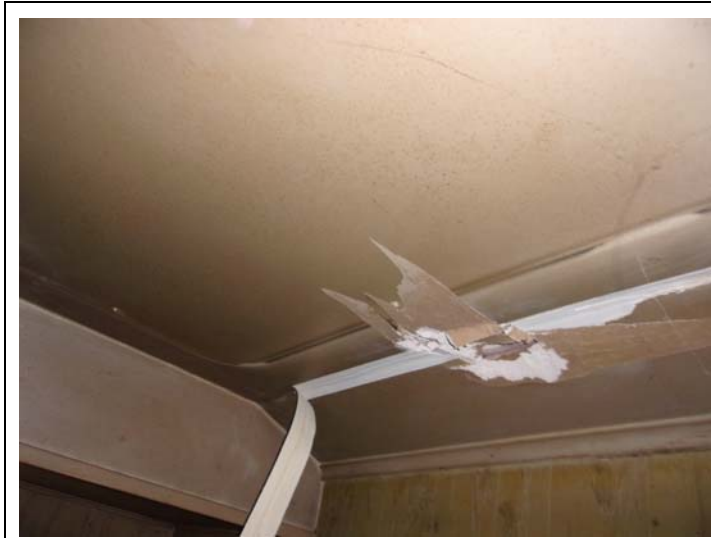
Photo 7 – Drywall with joint compound & tape in the bathroom ceiling
