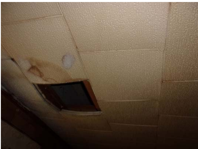
Photo 5 – 12" x 12" ceiling tiles with no mastic throughout
