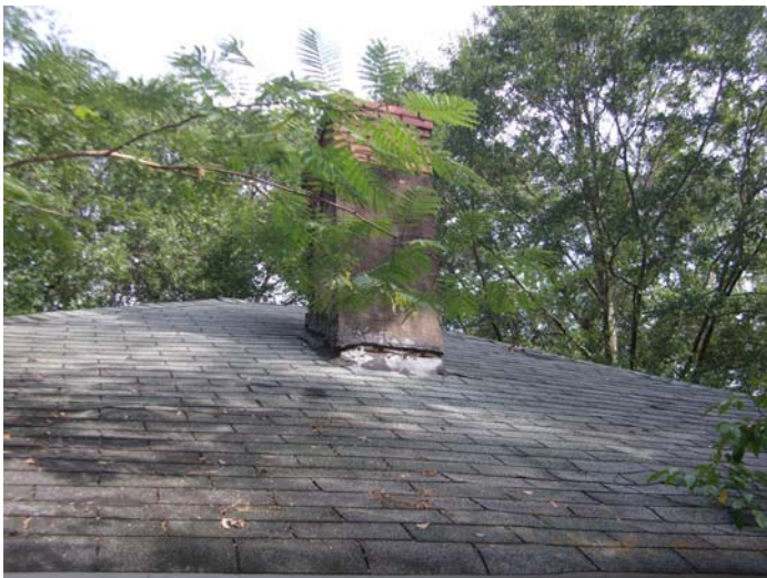
Photo 3 – 1 chimney wit mastic/tar – assumed positive
