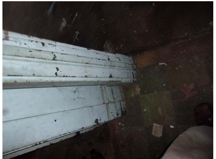
Photo 8 – Wooden window glazing
