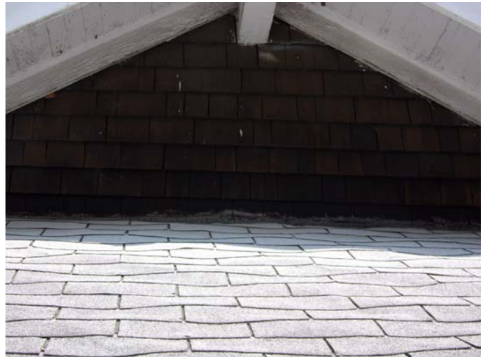
Photo 6 – Roof tar on flashing assumed positive
