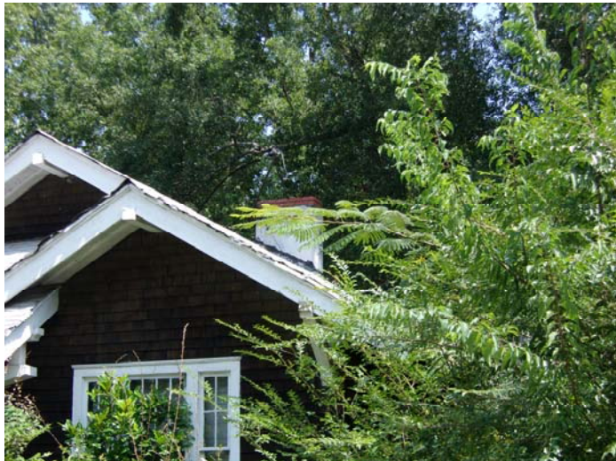
Photo 5 – Chimney assumed positive
