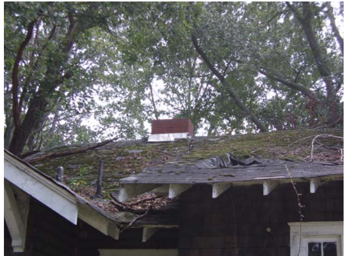
Photo 4 – Chimney assumed positive
