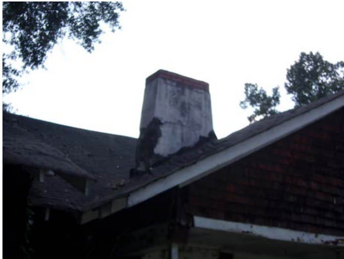
Photo 3 – Chimney assumed positive
