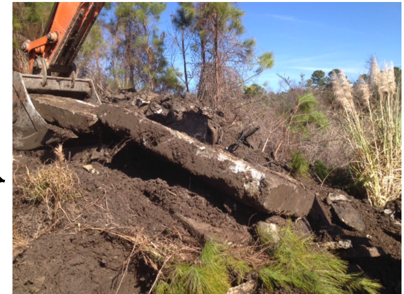
Photograph 1: Concrete Found in Mid-Atlantic Test Pit 5
