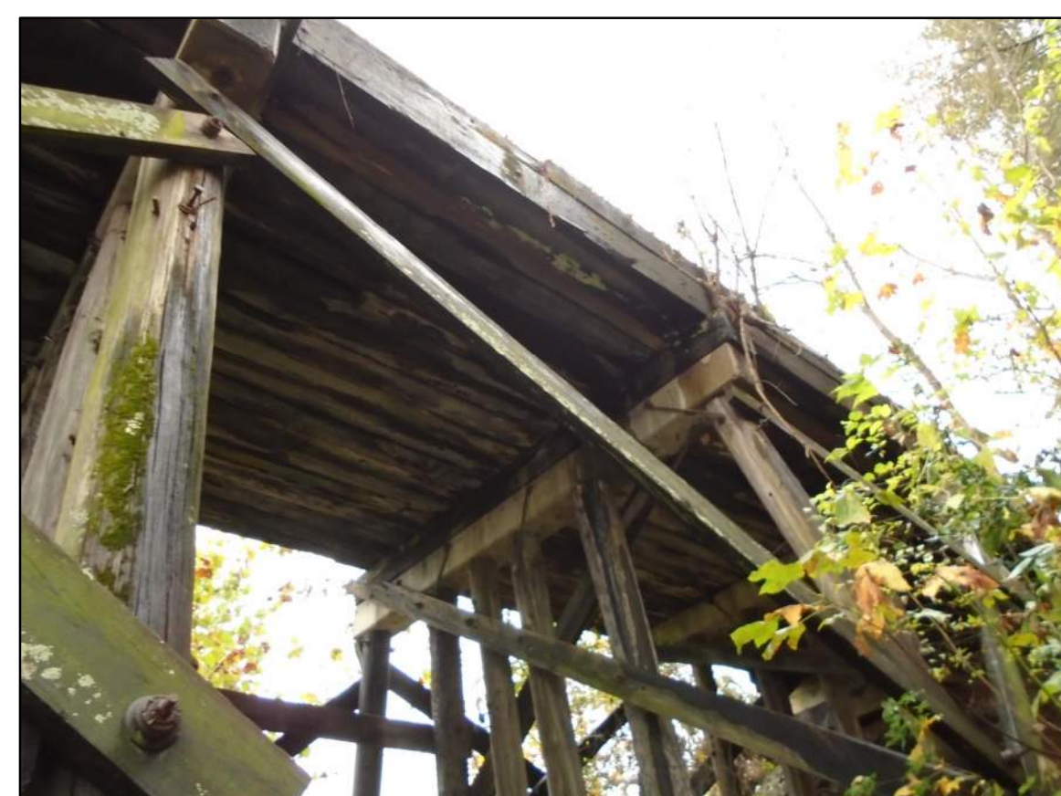
4 REPAIR PHOTO SCALE: NOT TO SCALE
