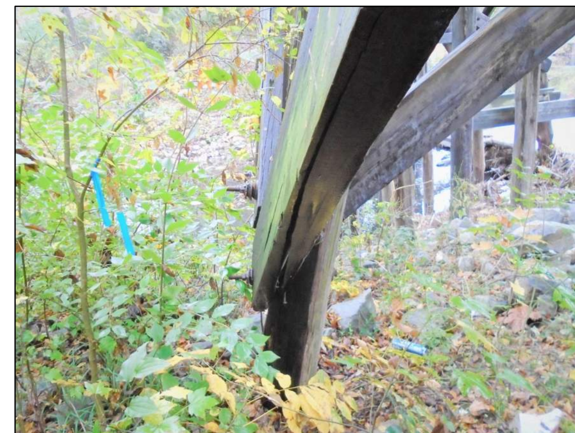
3 REPAIR PHOTO SCALE: NOT TO SCALE
