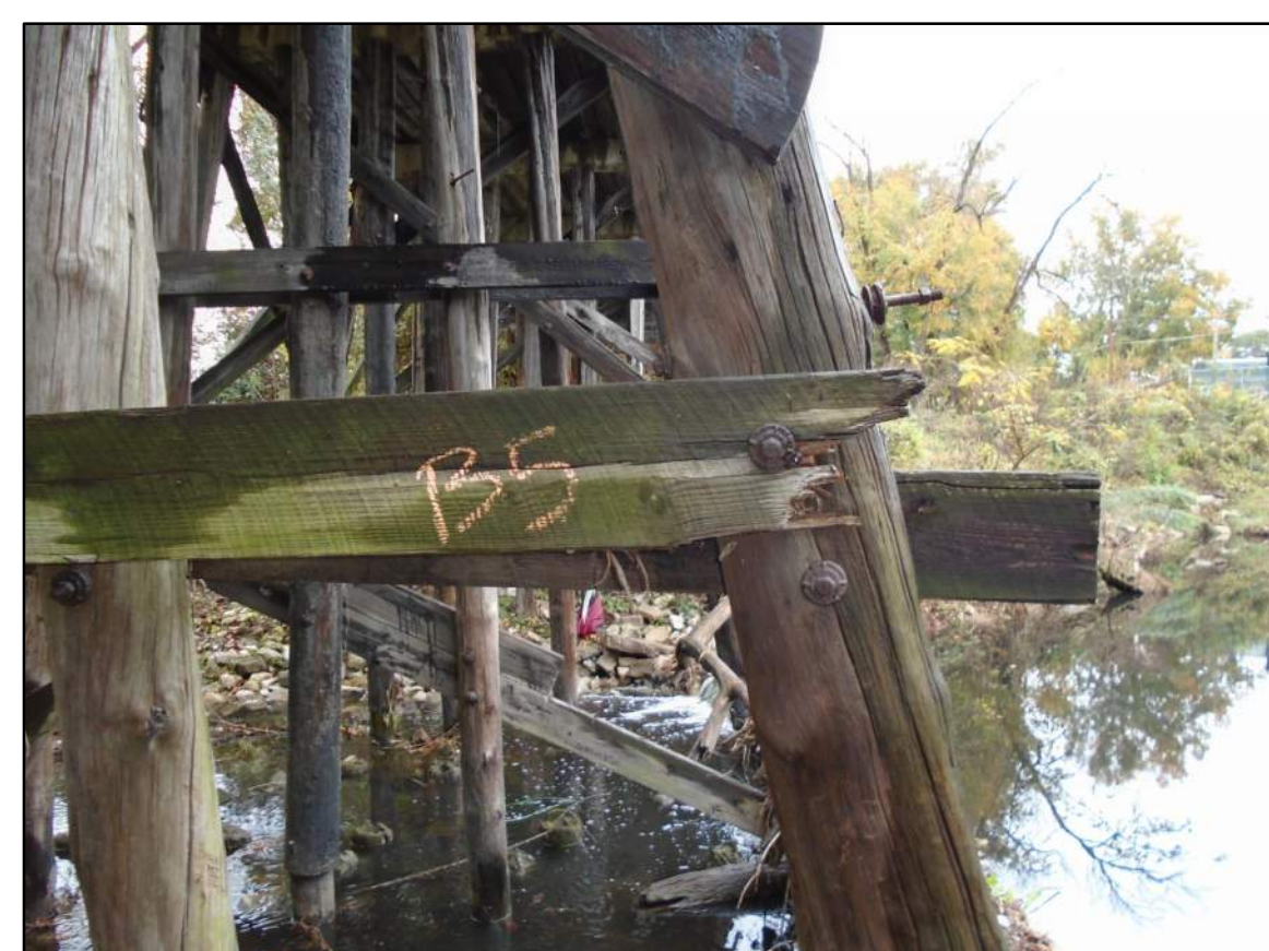
7 REPAIR PHOTO SCALE: NOT TO SCALE
