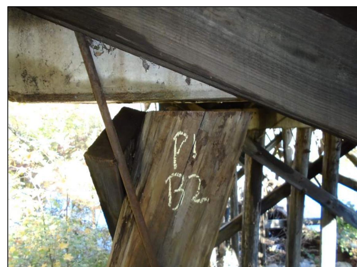
8 REPAIR PHOTO SCALE: NOT TO SCALE
