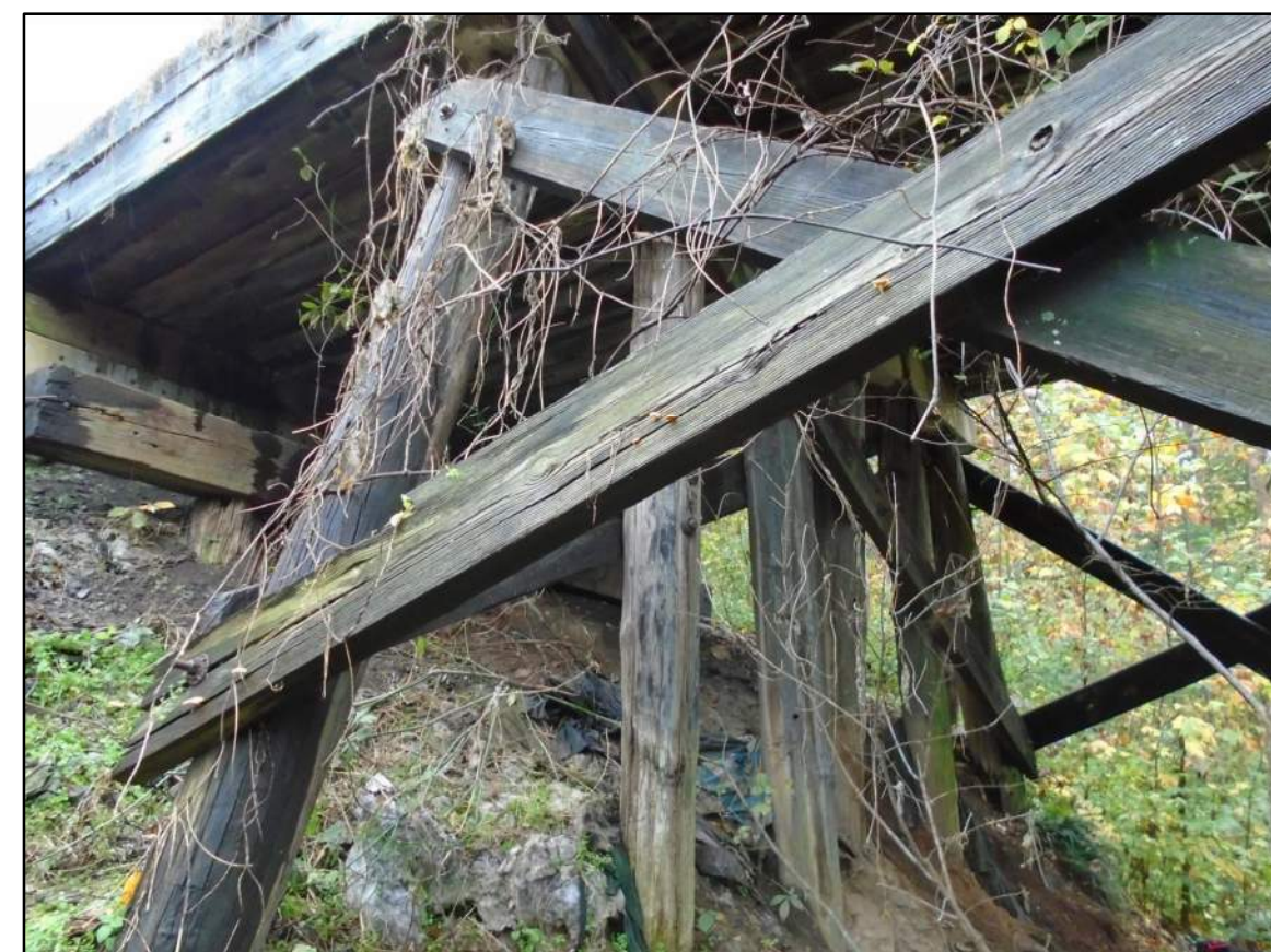
1 REPAIR PHOTO SCALE: NOT TO SCALE
