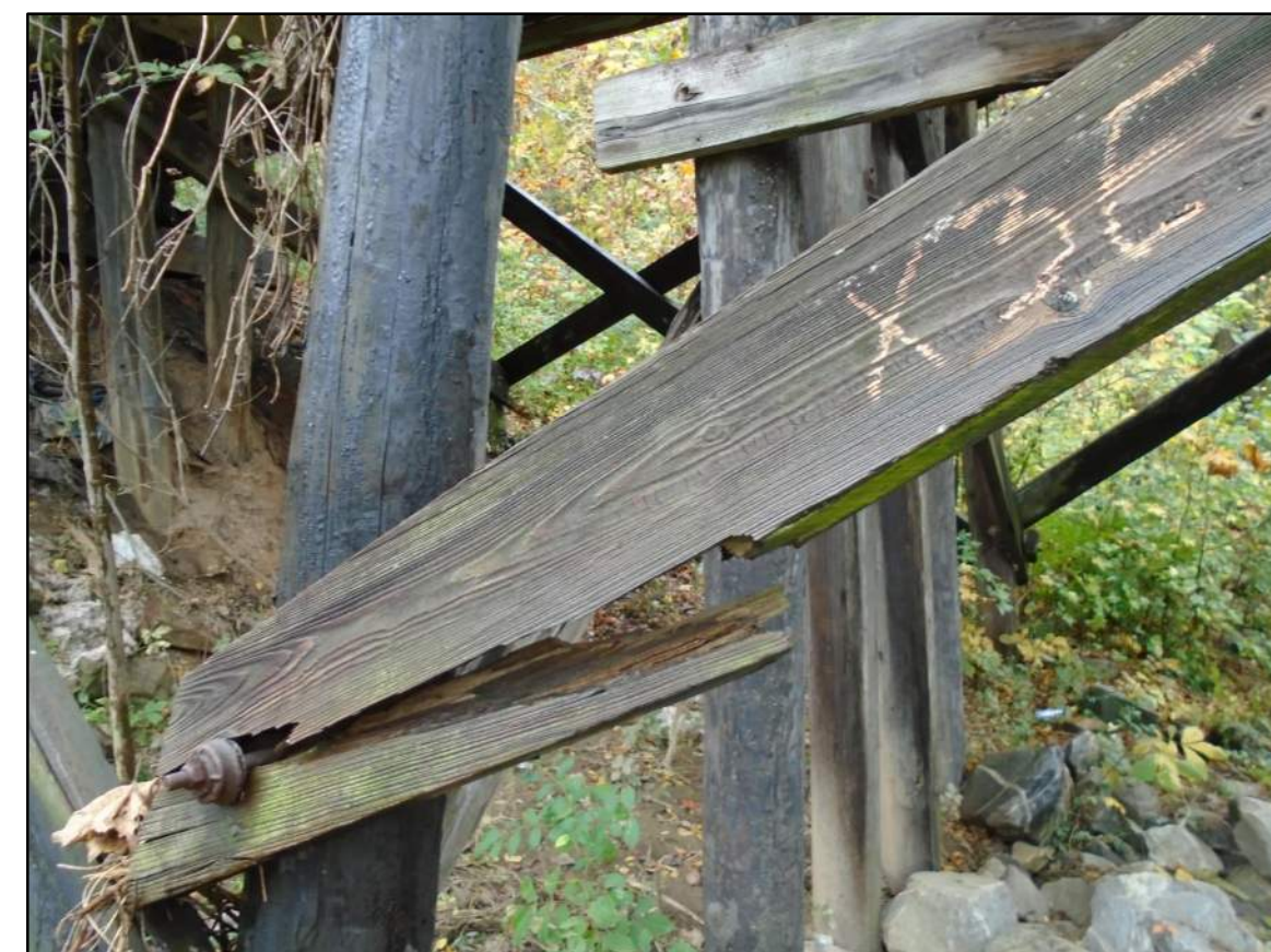
2 REPAIR PHOTO SCALE: NOT TO SCALE
