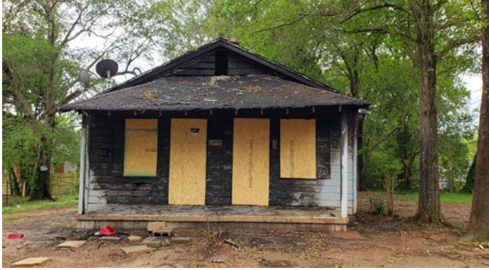
Photo 1 – 106 Norris Street in Spartanburg, South Carolina. Fire damage throughout the residence.
