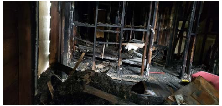
Photo 2 – Typical view of fire & structural damage throughout the interior.
