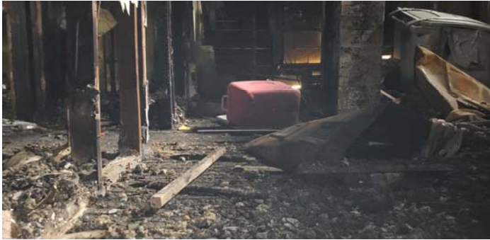
Photo 3 – Typical view of fire & structural damage throughout the interior.
