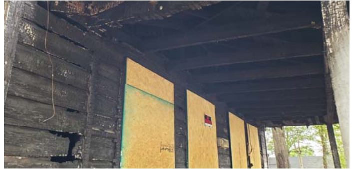
Photo 4 – Typical view of fire & structural damage throughout the exterior.
