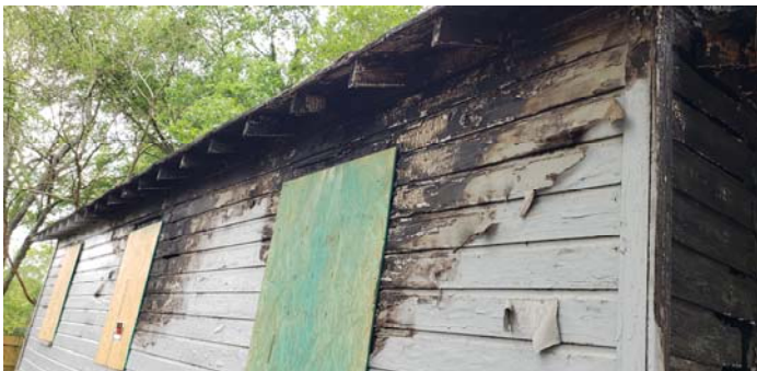
Photo 5 – Typical view of fire & structural damage throughout the exterior.
