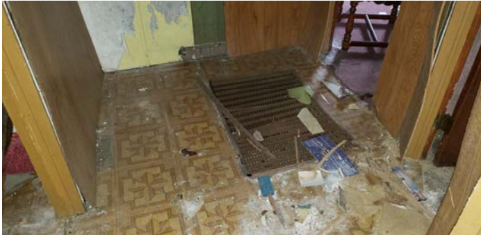
Photo 13 – Hallway with floor return that may be unstable.
