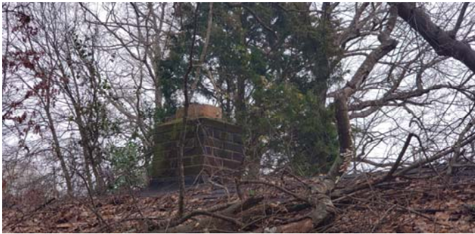
Photo 3 – Tar on chimney is assumed to be asbestos containing material.
