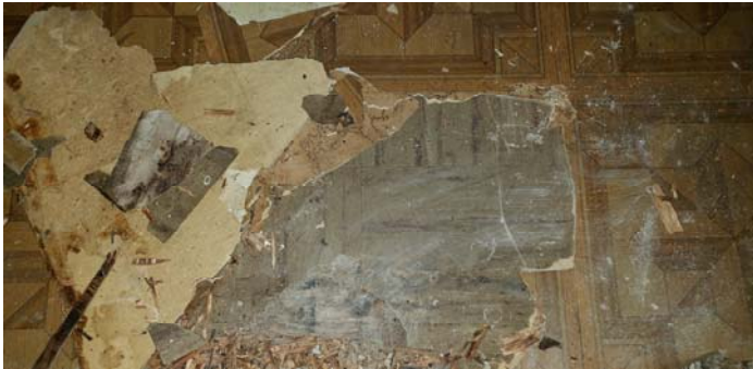
Photo 9 – Third layer of flooring in the bathroom is a 9"x9" gray tile and mastic.
