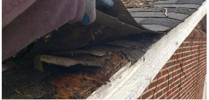
Photo 2 – One layer of black felt under four layers of shingles.
