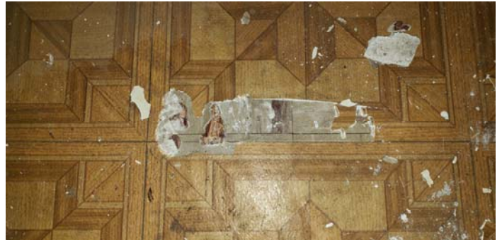
Photo 10 – Second layer of flooring in the kitchen is a thin tan/green tile and mastic.
