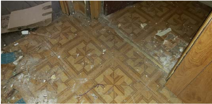
Photo 7 – 12"x12" wood star pattern self-stick flooring tile with adhesive located in hallway, top layer in bathroom and top layer in kitchen.
