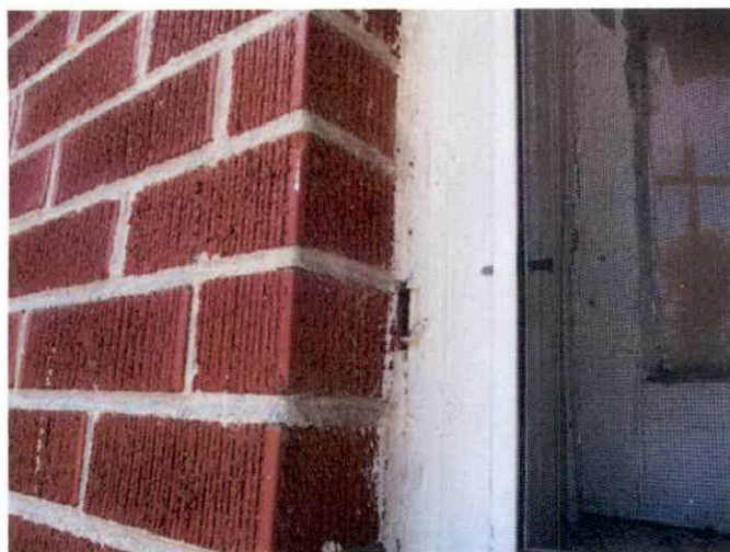
Photo 5 – Window & door casing caulk
