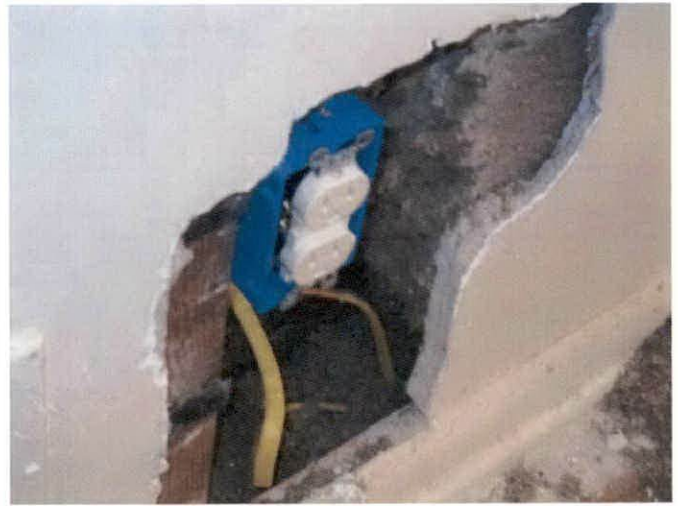
Photo 10 – Plaster with finish over unfinished drywall walls throughout
