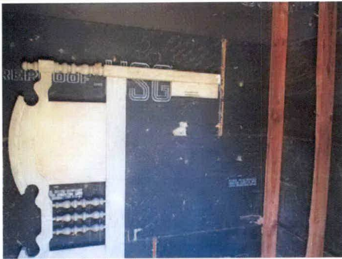
Photo 7 – Unfinished drywall in the exterior back storage room
