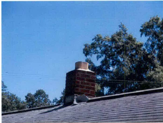
Photo 3 – 1 chimney with tar – assumed positive
